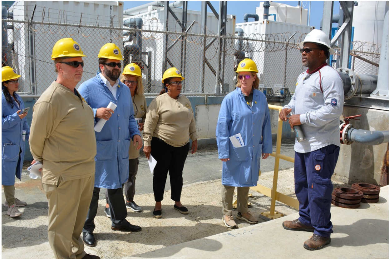
St. Croix, USVI – FEMA Administrator Deanne Criswell receives a tour of the Virgin Islands Water and Power Authority Estate Richmond Power Plant and Water Desalination Plant to discuss ongoing projects and internal operations to improve the territory’s power and water infrastructure and reliability. (FEMA Photo by Brett Walsh)
