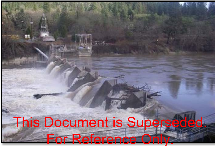
The Big Lake Dam, an unregulated structure located along Tributary A, causes upstream backwater during flood events; makes portions of River Road un-passable; and several homes receive flooded yards and basements
