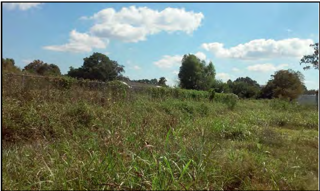
Figure 6: Fence along concrete ditch between Dillard and City New Orleans Parks and Parkways property (29.998692, -90.067592). (Source: FEMA, 10/28/2015)
