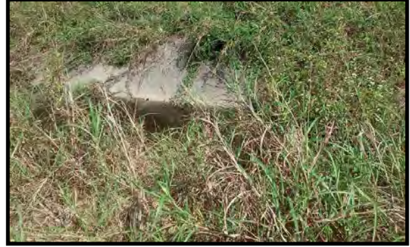
Figure 9: Concrete ditch to be improved, grass overgrown. (Source: FEMA, 10/28/2015)
