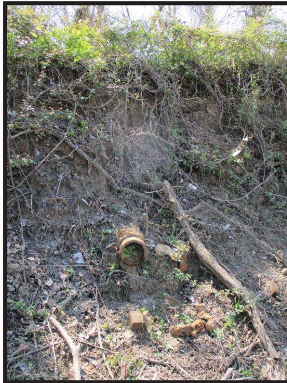
Figure 8. Revetment-2, facing east, bank profile displaying exposed cultural materials (03/15/2017).
