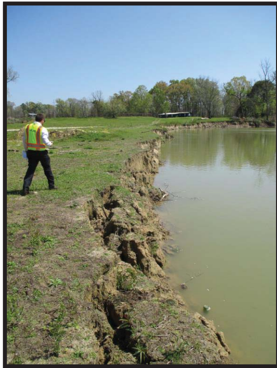
Figure 10. Displaying recent erosion, facing east from the northeastern extent of the proposed Revetment-1 area (03/15/2017).
