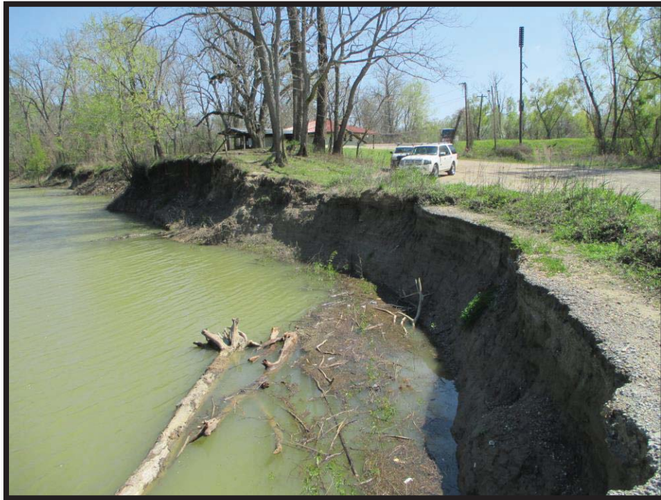
Figure 7. Revetment-2, cut-bank facing northeast, displaying ongoing erosion (03/15/2017)
