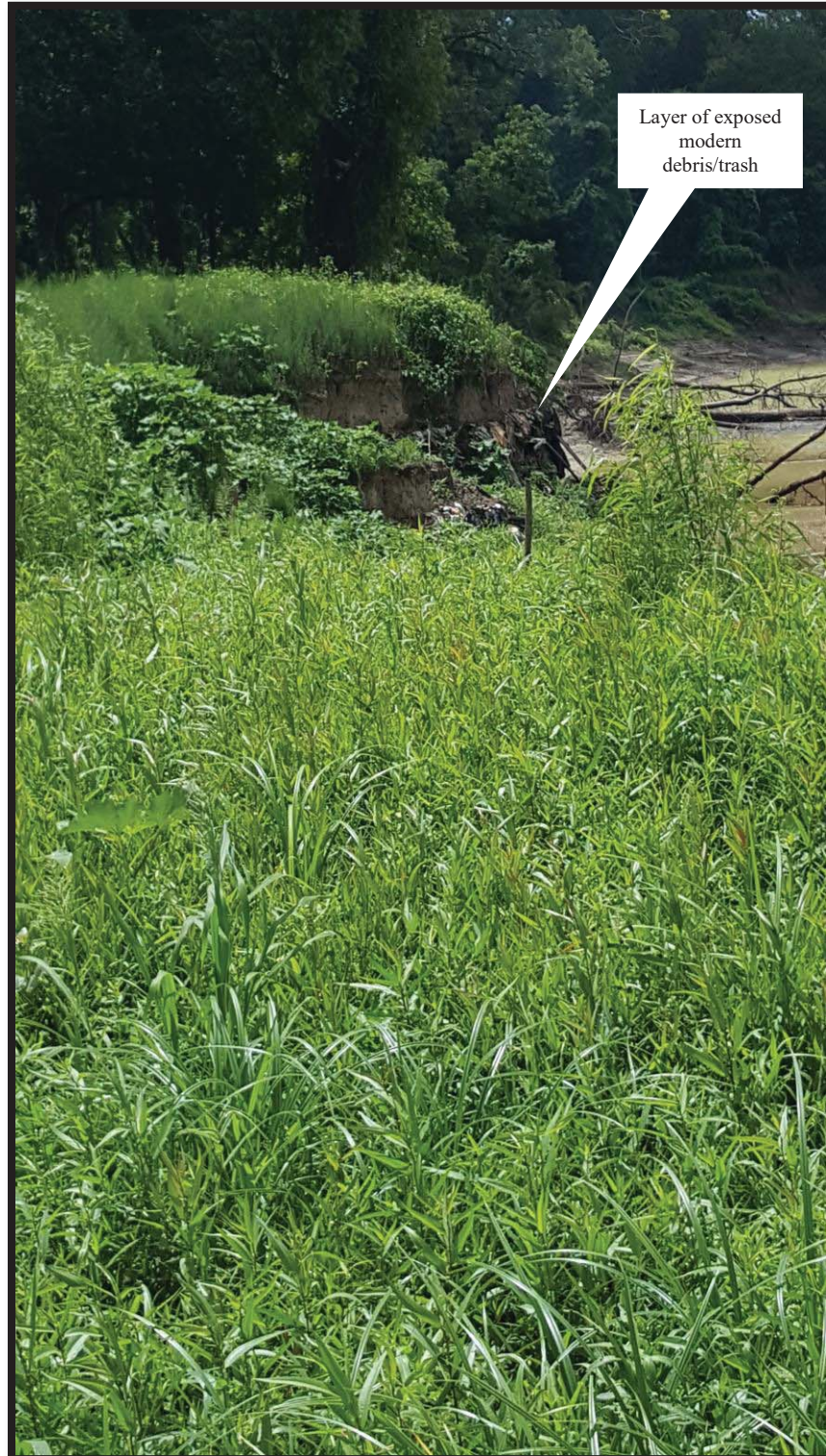
Figure 5. Revetment-1, facing southeast, displaying modern debris/trash deposit (07/28/2016).
