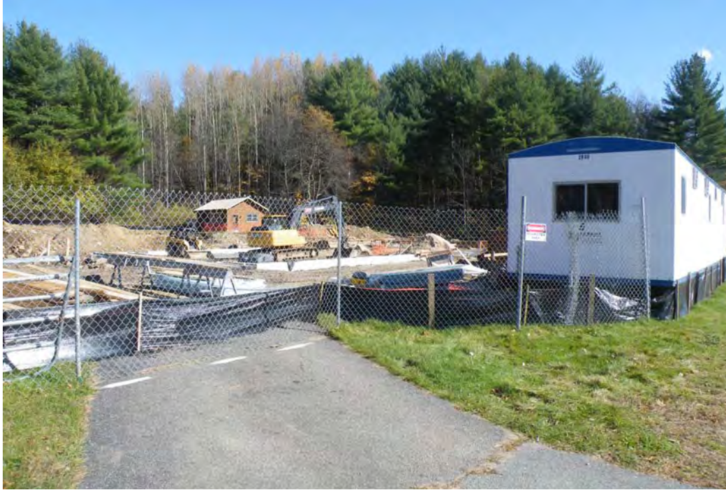
Figure 4. View southeast along New York State Route 9N at construction site for the new Keene fire station.
