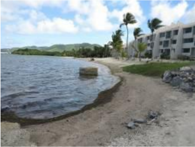
Photograph 1. Due to erosion over time, manhole (MH) 0438 between Sugar Beach and Colony Cove is now more than 10 feet off shore. (Photograph courtesy of Bioimpact, Inc.).
