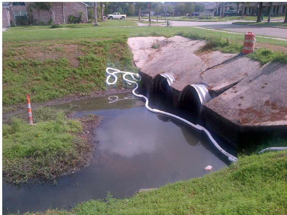
Figure 14: Location of proposed 20 Arpent arch bridge. These existing culverts would be removed
