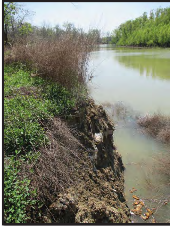
Figure 9. Revetment-1, facing southeast, displaying modern debris/trash deposit (03/15/2017).
