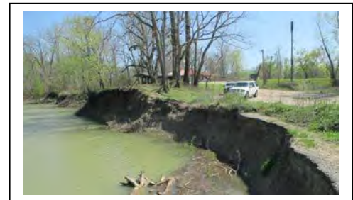
Cut bank at Bayou Sara facing northeast, showing the ongoing erosion. FEMA
