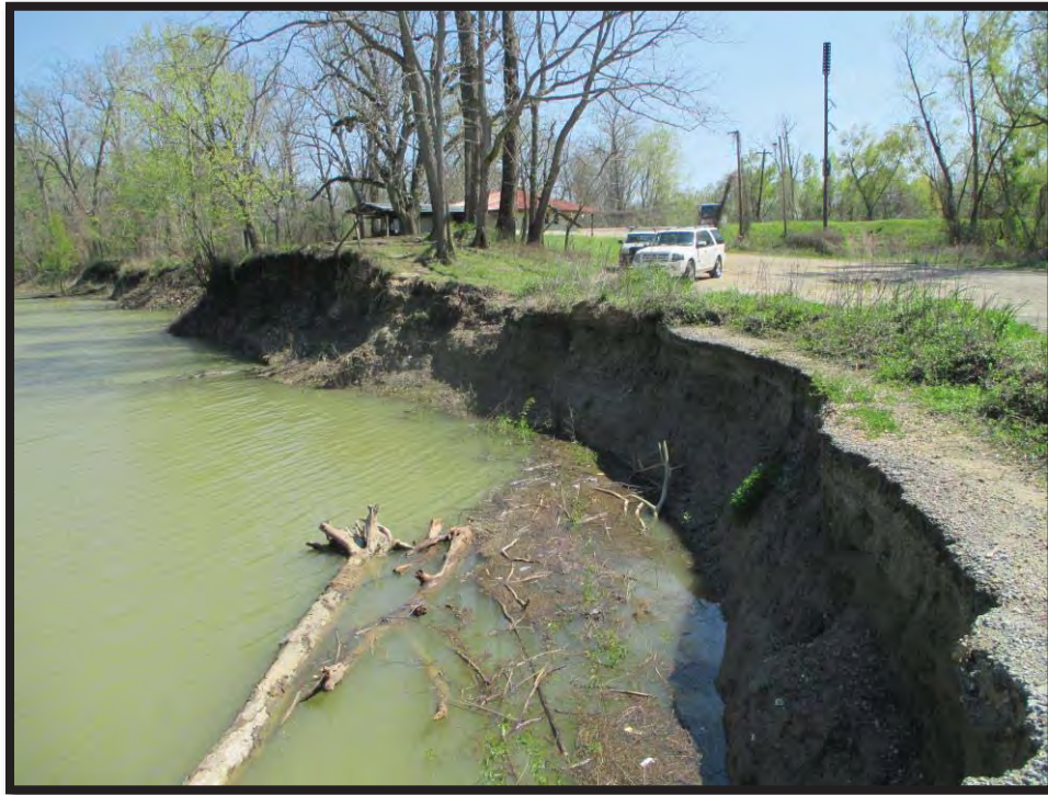
Figure 7. Revetment-2, cut-bank facing northeast, displaying ongoing erosion (03/15/2017)
