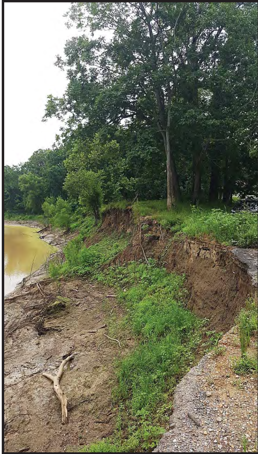
Figure 6. Revetment-2, facing northeast, displaying heavy bank erosion during low water (07/28/2016).
