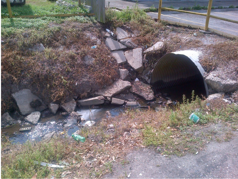
Figure 11: Area where new culvert will be replaced with boxed culvert on Palmisano Canal going downstream
