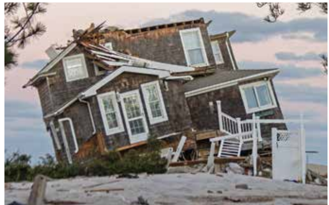
This house in Mantoloking, New Jersey, was destroyed by the storm surge of Hurricane Sandy
