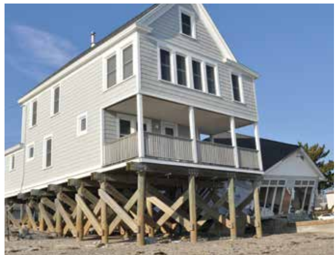
This elevated home in Milford, Connecticut, sustained minimal damage from Hurricane Sandy while neighboring homes were destroyed
