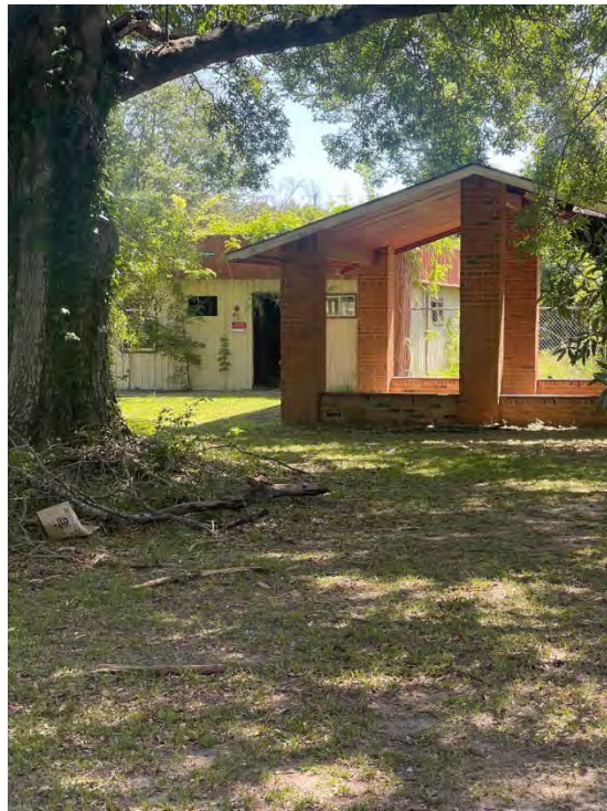
Photo 12. View of damaged maintenance shed building.
