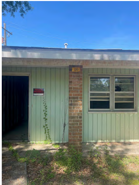
Photo 2. View of existing damaged duplex housing unit # 130.
