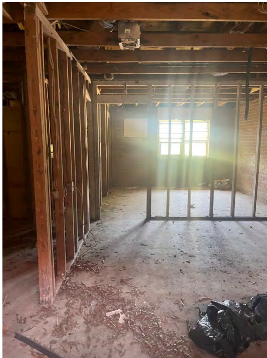
Photo 10. View of interior of damaged housing unit
