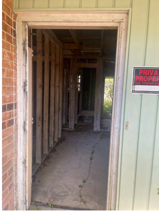
Photo 3. View of interior of damaged housing unit.
