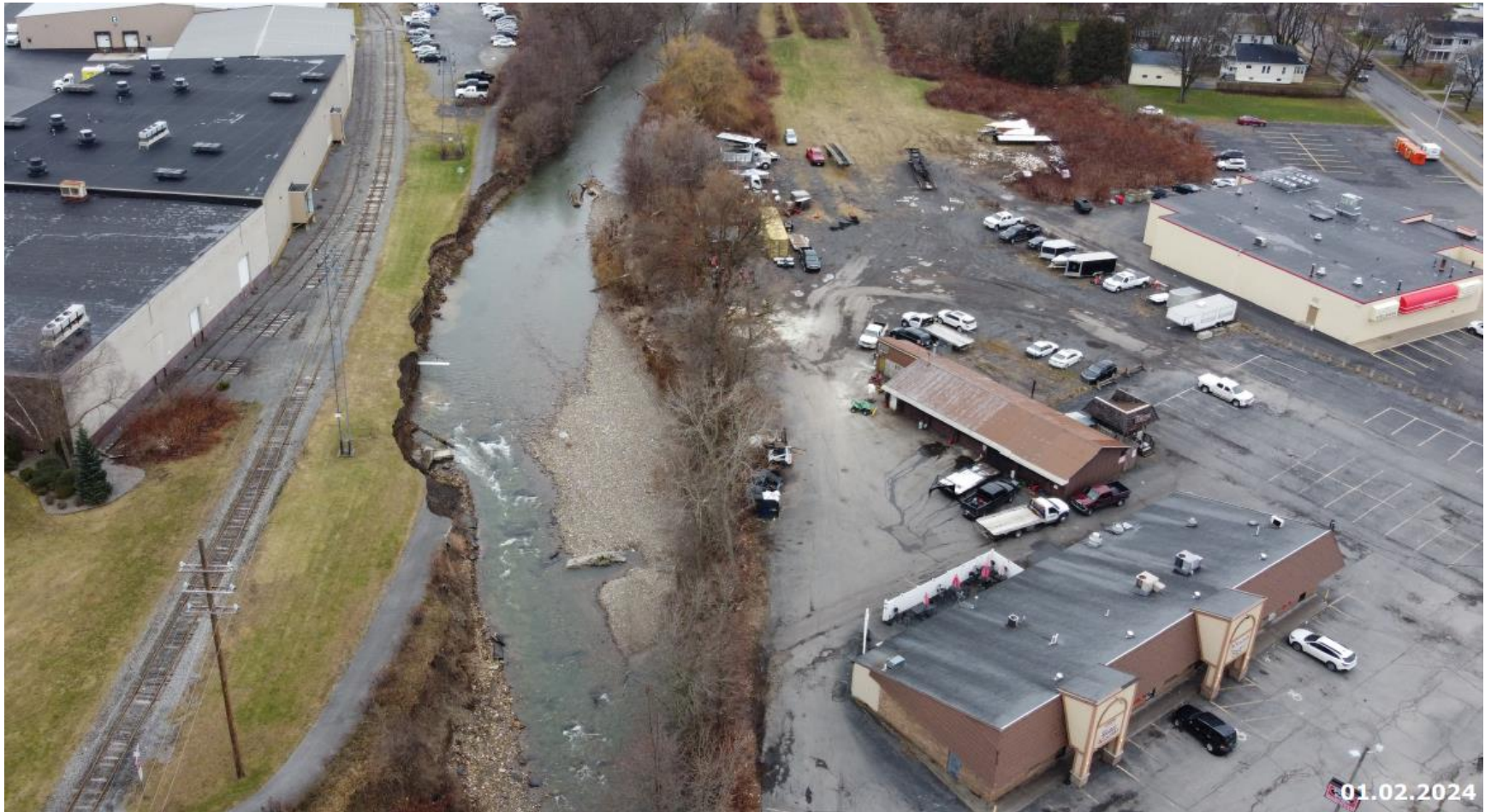
Figure I - January 2024 aerial photo of eroded bank at McCraith Beverages site
