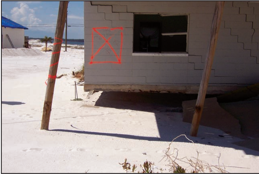
Figure 6-3. NAVARRE BEACH, FLORIDA: Close-up of foundation failure shown in Figure 6-2. (Source: FEMA 489)
