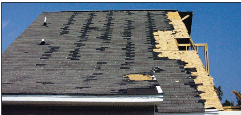
Figure 8-6. Roof failures that resulted from asphalt shingles being installed in a raking fashion. (Source: FEMA 489)
