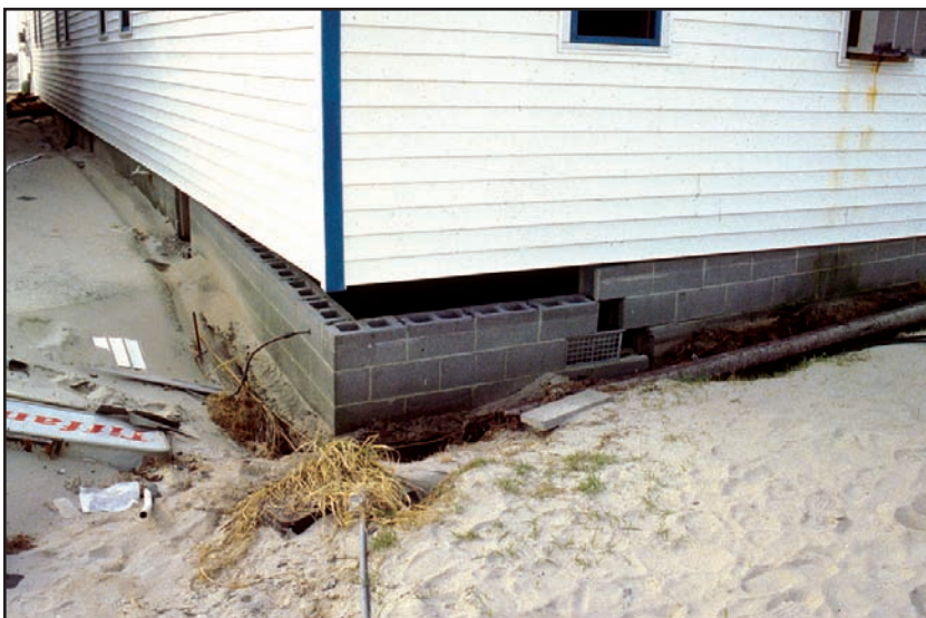
Figure 6-6. Failure of crawlspace foundation undermined by scour. (Source: FEMA 290)
