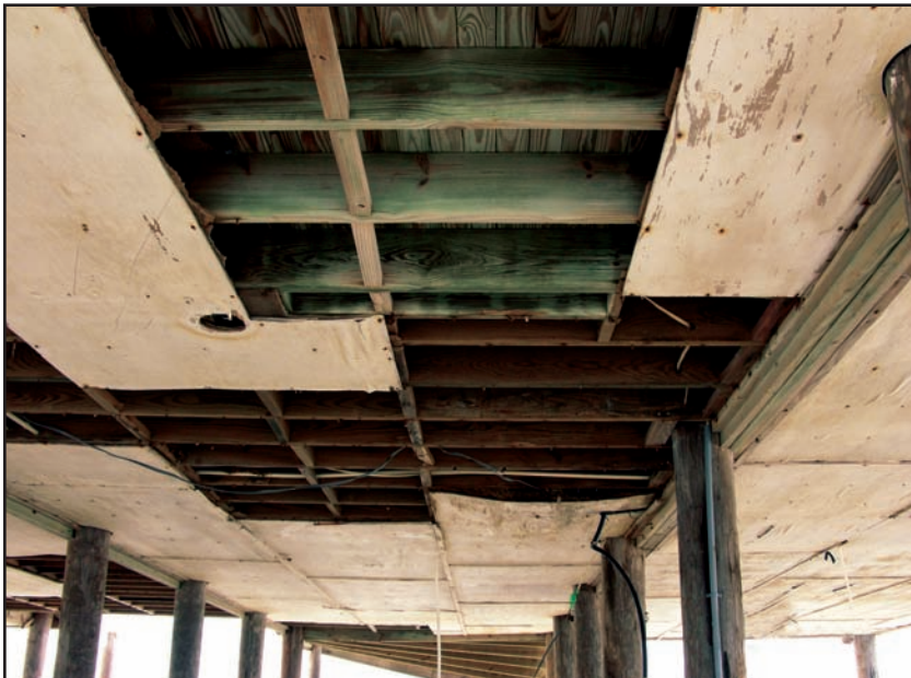
Figure 9-12. Example of an exterior floor covering system damaged by Hurricane Ivan. Note the good condition of the floor joists and flooring, due to their protection from salt spray prior to the storm. (Source: FEMA 489)
