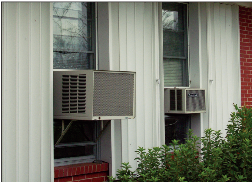
Figure 10-5. PENSACOLA, FLORIDA: Shutters had been attached to this building in order to protect it from windborne debris. However, areas above and below the air conditioning units were left unprotected. (Source: FEMA 489)
