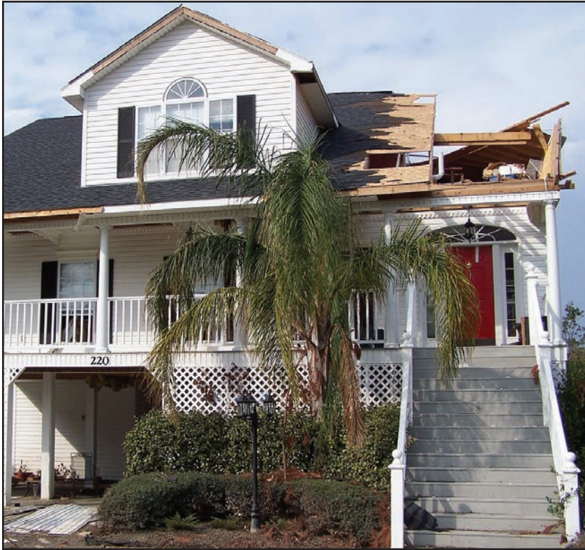
Figure 5-5. PASS CHRISTIAN, MISSISSIPPI: Newer home damaged from internal pressurization and inadequate connections. (Source: FEMA 549)
