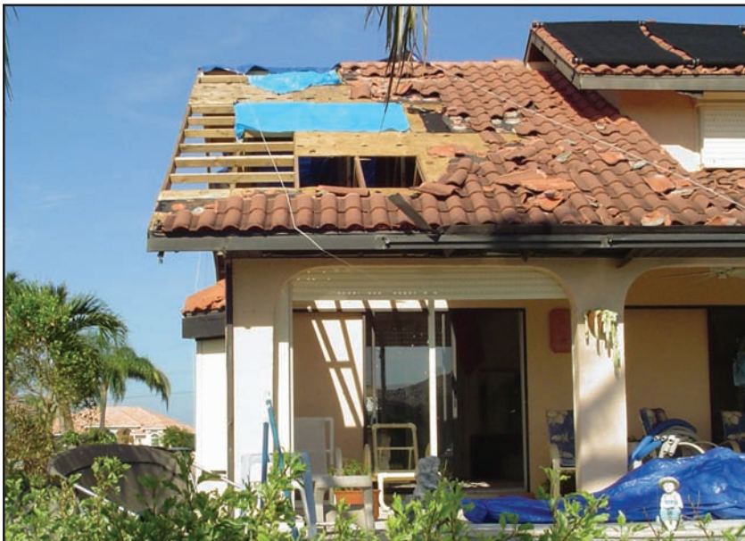
Figure 5-4. PUNTA GORDA, FLORIDA: Load path failure in connections between roof decking and roof framing. (Source: FEMA 488)
