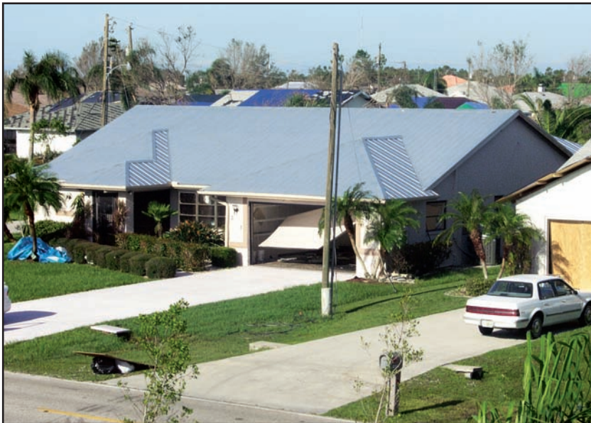
Figure 10-8. Negative pressure failure of garage door. (Source: FEMA 488)
