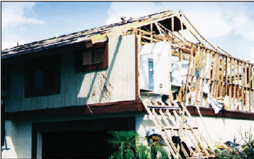
Figure 5-1. DADE COUNTY, FLORIDA, HURRICANE ANDREW (1992): Second-story wood framing (on first-story masonry). Load path failure at end gable. (Source: FEMA 55)
