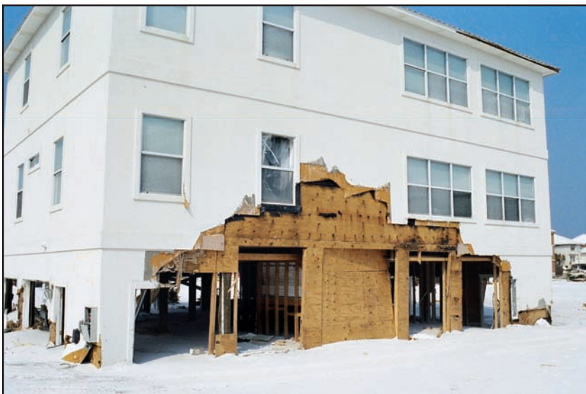
Figure 6-18. Building damages due to the incorrect construction of a breakaway wall. (Source: FEMA 489)
