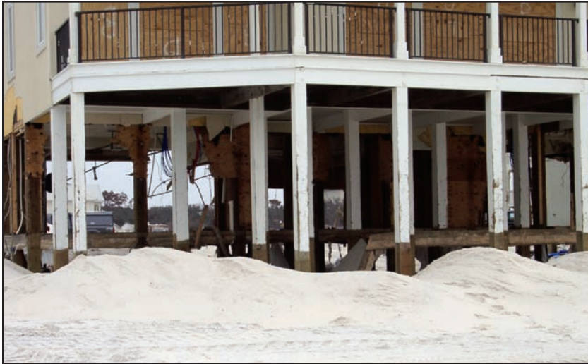
Figure 6-17. Successful use of a breakaway wall. (Source: FEMA 489)
