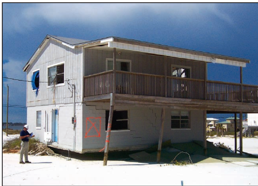
Figure 6-2. NAVARRE BEACH, FLORIDA: Slab-on-grade foundation failure due to erosion and scour undermining. (Source: FEMA 489)
