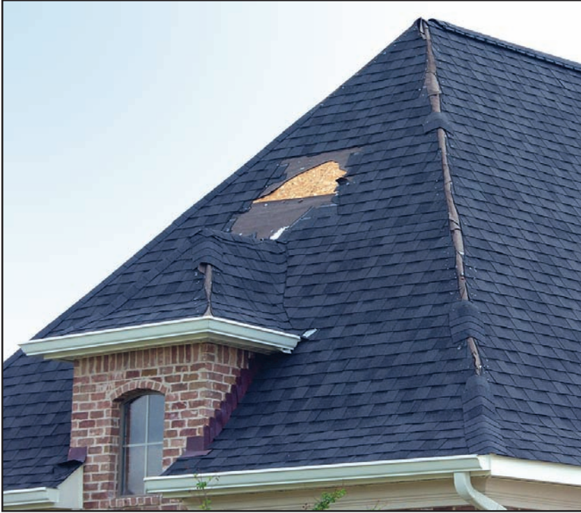
Figure 8-1. Instance where wind pressures exceeded the strength of the asphalt roofing. (Source: FEMA 549)
