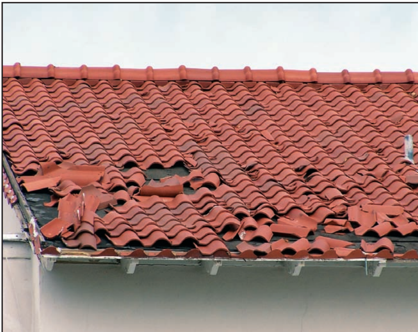
Figure 8-8. Clay tile roof failure. The tiles were dislodged due to inadequate anchorage. (Source: FEMA 549)
