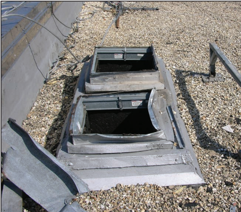
Figure 8-2. GULFPORT, MISSISSIPPI: Winds dislodged roof mounted equipment and created large openings in the roof system. (Source: FEMA 549)
