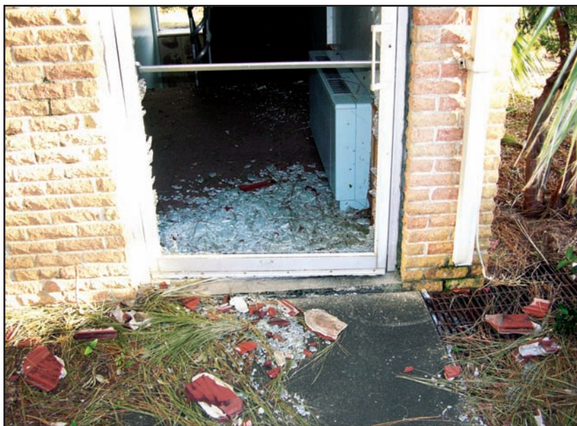
Figure 10-6. PENSACOLA, FLORIDA: Failure of glazing from windborne debris created by dislodged tile roofing. (Source: FEMA 489)
