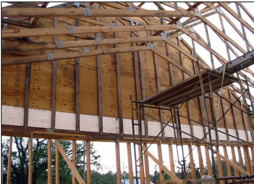
Figure 7-14. Improperly braced gable walls. The ceiling diaphragm (i.e., the bottom chords of the scissor truss) is located several feet above the top of the end wall top plate and no wall-to-truss bracing is provided. (Source: FEMA 549)
