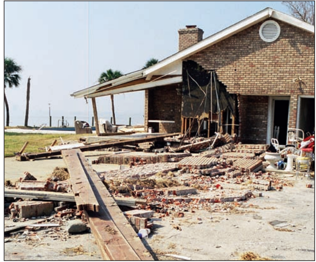
Figure 2-11. Example of surge, wave, and debris damage. (Source: FEMA 489)
