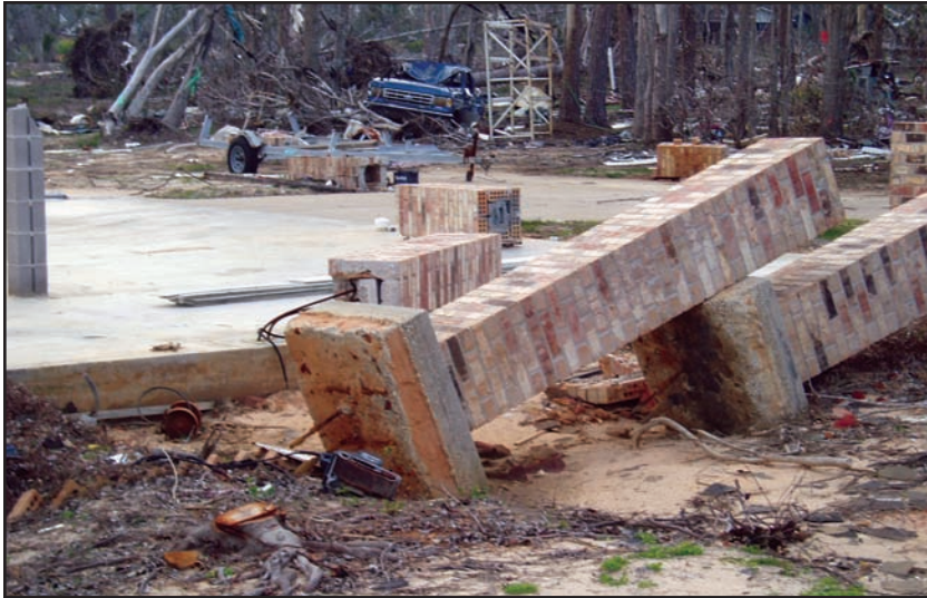
Figure 6-20. PASS CHRISTIAN, MISSISSIPPI: Performance comparison of shallow, open foundations founded on discrete footings (foreground) failed by rotating and overturning, while piers located on more substantial footings—in this case, a concrete mat (background)—survived. (Source: FEMA 549)
