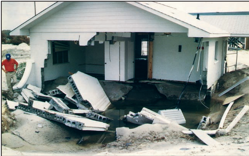
Figure 6-5. Building failure caused by undermining of crawlspace foundation during Hurricane Fran. Breaking waves may also have contributed to foundation failure. (Source: FEMA 290)
