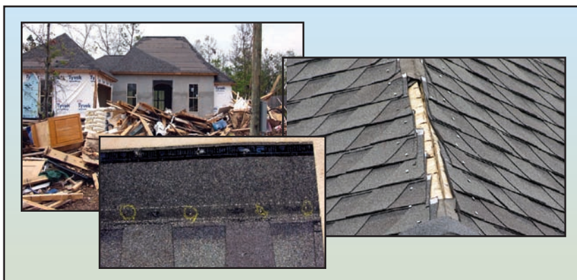
Figure 8-7. Loss of asphalt shingle roofing along hip. Best Practices approaches contained in Technical Fact Sheet No. 20 help prevent this mode of failure. (Source: FEMA 489)
