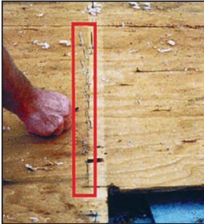
Figures 7-5 and 7-6. Exterior and interior views of connection issues between the roof sheathing and the top chords of the roof truss system. (Source: FEMA 55)
