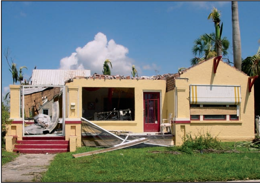
Figure 5-3. PUNTA GORDA, FLORIDA: Roof framing damage and loss due to load path failure at top of wall/roof structure connection. (Source: FEMA 488)
