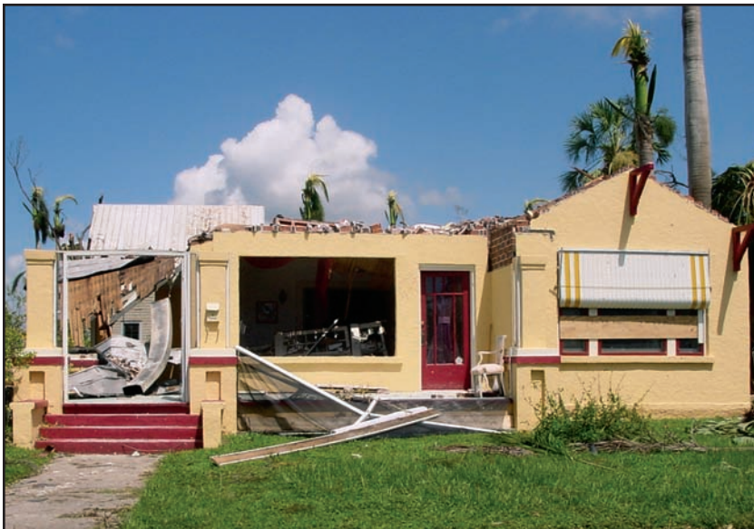
Figure 10-1. PUNTA GORDA, FLORIDA: Failure of a roof structure from pressurization of a house when the window failed on the windward face. (Source: FEMA 488)
