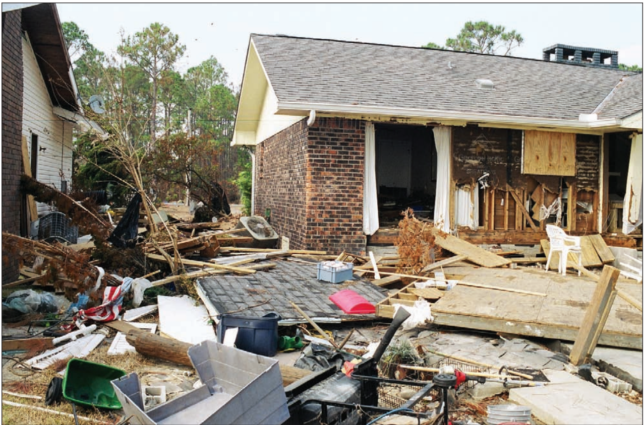
Figure 2-12. BIG LAGOON, ALABAMA: Buildings constructed on piles and elevated several feet above the base flood elevation (BFE) sustained less flood damage than adjacent buildings at lower elevations. (Source: FEMA 489)
