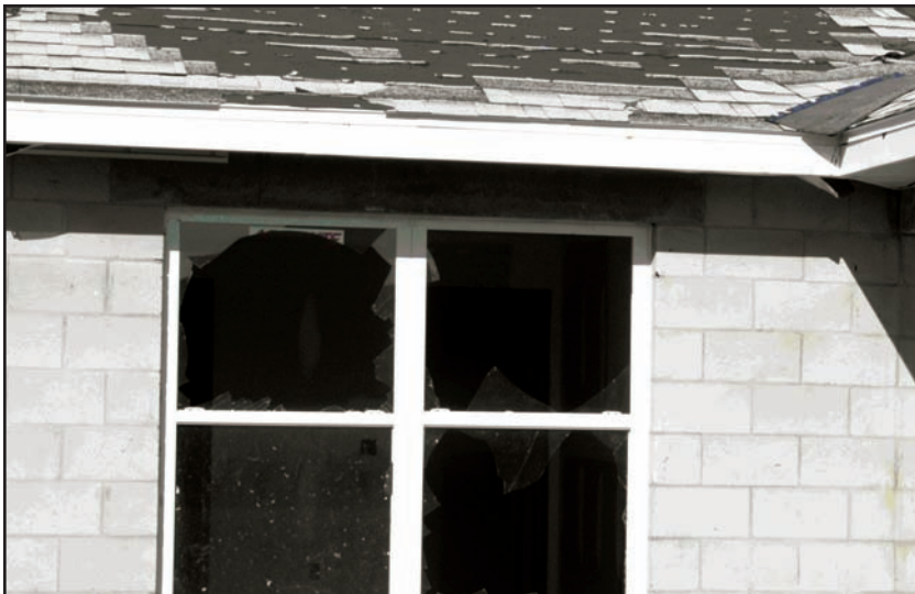
Figure 10-3. PUNTA GORDA, FLORIDA: Glazing failure due to windborne debris from displaced roofing. (Source: FEMA 488)
