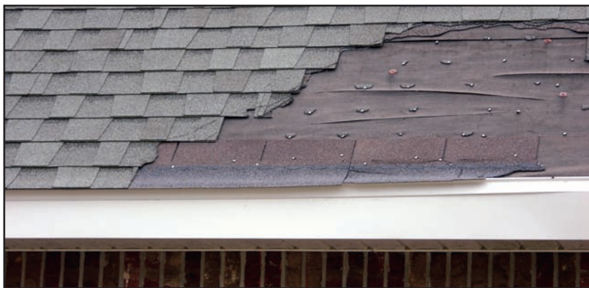
Figure 8-5. Roof failures that resulted from improper starter-strip installation. (Source: FEMA 549)
