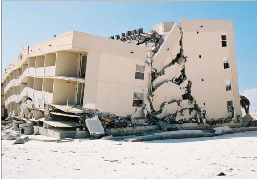
Figures 2-5 and 2-6. ORANGE BEACH, ALABAMA: Collapse of five-story, multi-family buildings on shallow foundations. (Source: FEMA 489)
