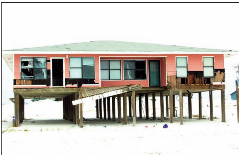
Figure 10-4. Glazing failure due to windborne debris. An oceanfront home damaged during Hurricane Ivan due to windows being broken by windborne debris. (Source: FEMA 489)
