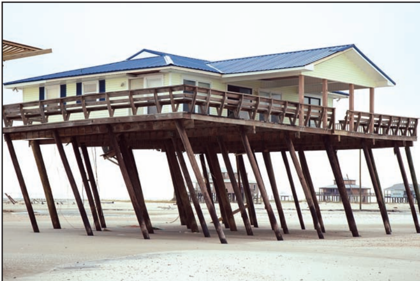
Figure 6-11. DAUPHIN ISLAND, ALABAMA: Structure near collapse due to insufficient pile embedment. (Source: FEMA 549)
