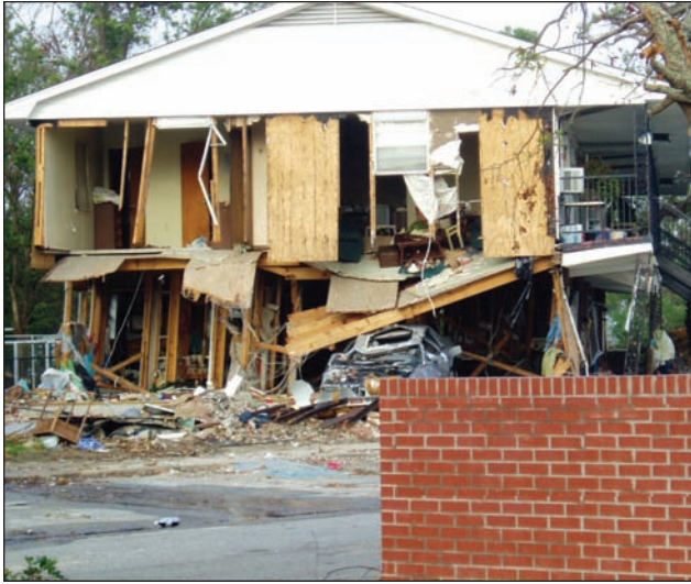
Figure 2-10. Example of surge, wave, and debris damage. (Source: FEMA 549)
