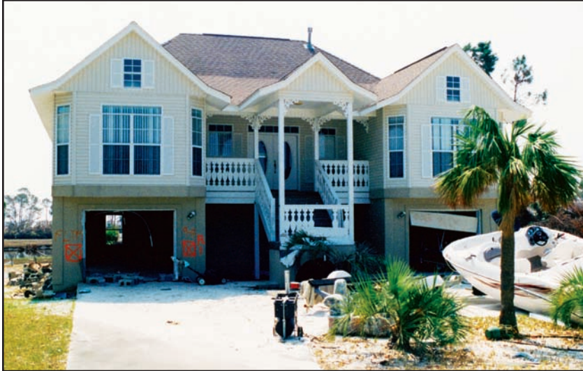
Figure 5-9. BIG LAGOON, FLORIDA: Elevated building (constructed to newer code) that survived Hurricane Ivan. (Source: FEMA 489)
