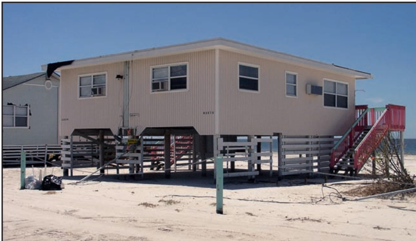
Figure 6-8. FORT MYERS BEACH, FLORIDA: Oceanfront house constructed on an open foundation sustained only minor damage after being exposed to high winds and storm surge. (Source: FEMA 488)
