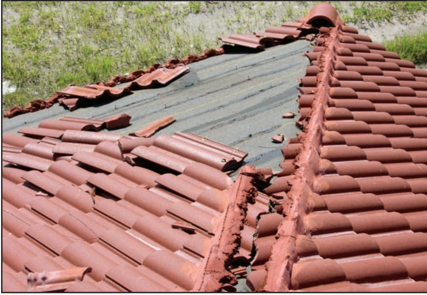
Figure 8-9. Storm damage to a tile roof system. (Source: FEMA 488)
