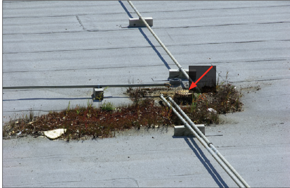
Figure 6-32: Dirt and vegetation surrounded this roof drain (red arrow) and impeded drainage. Roof drains should be checked at least annually and cleaned of debris if found. Drains should also be checked prior to hurricane landfall. Hurricane Ike (Texas, 2008)
