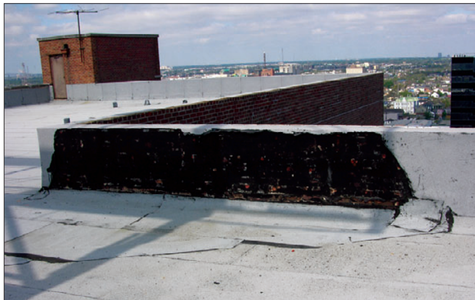
Figure 6-133: Failed base flashing adhered directly to the brick parapet. Estimated wind speed: 105 mph. Hurricane Katrina (Louisiana, 2005)
