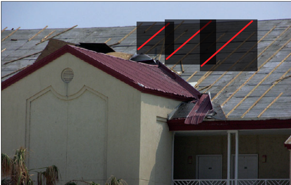
Figure 6-30: In most of the areas on this roof, the connection of the top nailer to the bottom nailer was the weakest link. However, in a few locations, the connection of the bottom nailer to the roof structure was the weak link (three of the blown-off bottom nailers are shown by the red lines).
