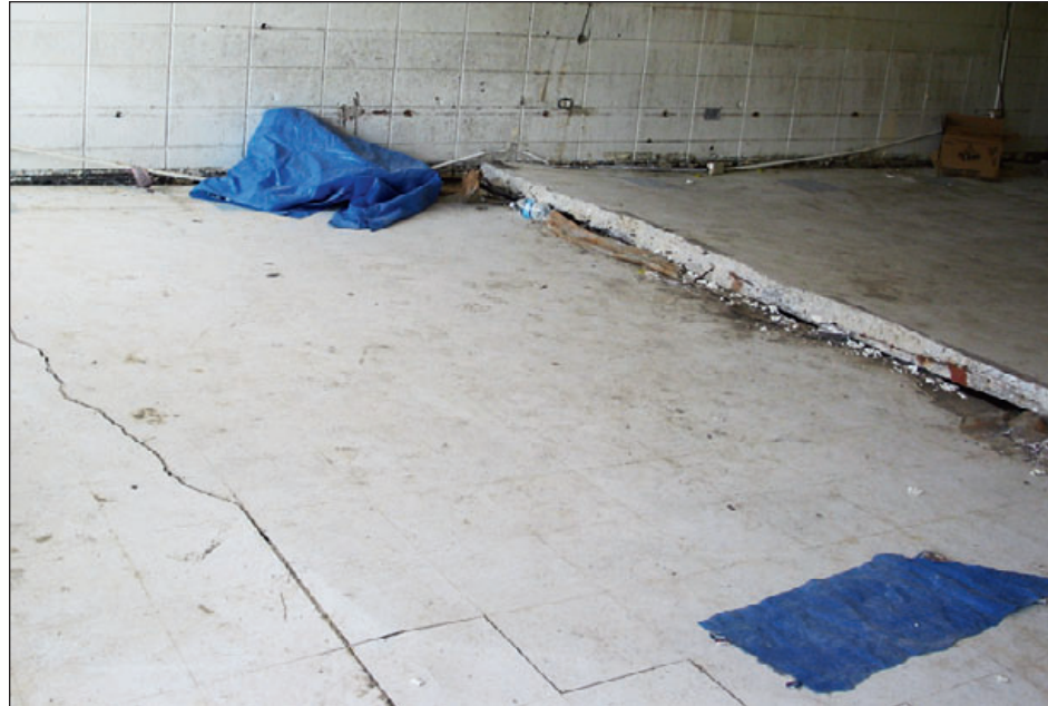
Figure 5-15: Concrete slab ruptured by hydrostatic pressure (buoyancy) induced by the floodwaters of Hurricane Katrina (2005)
