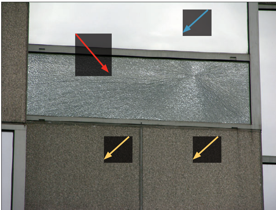
Figure 6-54: The red arrow shows a piece of laminated glass that was broken, but remained in the frame to protect the building's interior. The blue arrow shows unbroken laminated glass. The yellow arrows show granite wall panels. Estimated wind speed: 105 mph. Hurricane Katrina (Louisiana, 2005)
