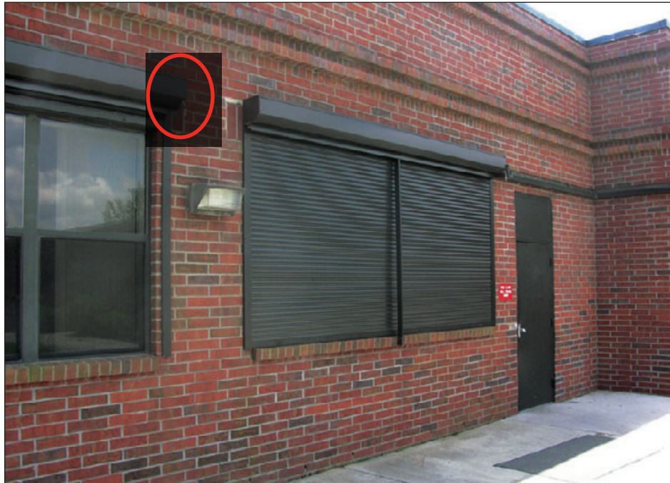
Figure 6-128: This school has roll-down shutters. The toggle in the red circle allows the shutter to be manually raised. Estimated wind speed: 130–140 mph. Hurricane Charley (Florida, 2004)
