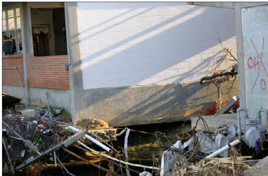
Figure 5-16: Scour undermined the foundation of St. Paul Catholic School, Pass Christian, LA.
