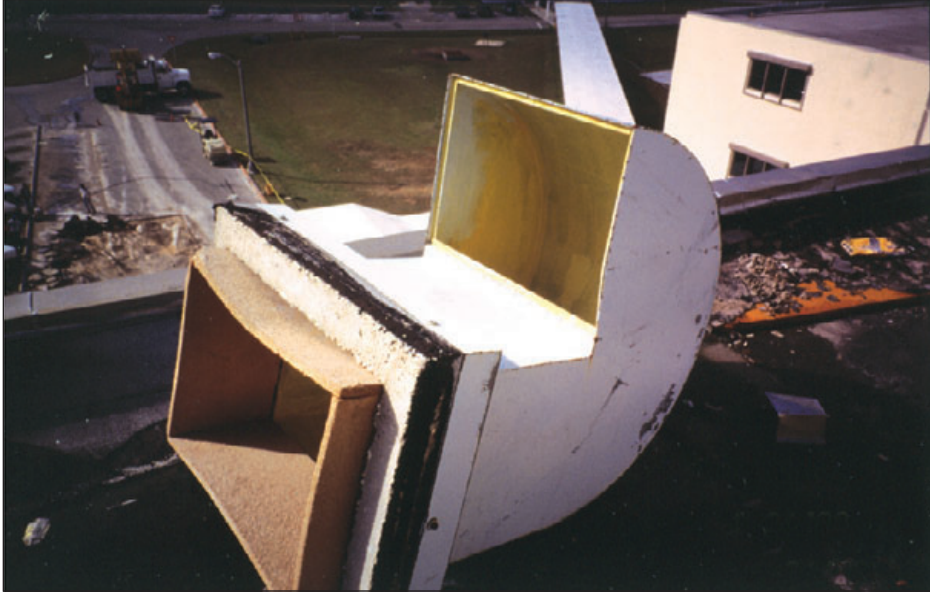
Figure 6-91: The gooseneck on this building remained attached to the curb, but the curb detached from the deck. Typhoon Paka (Guam, 1997)
