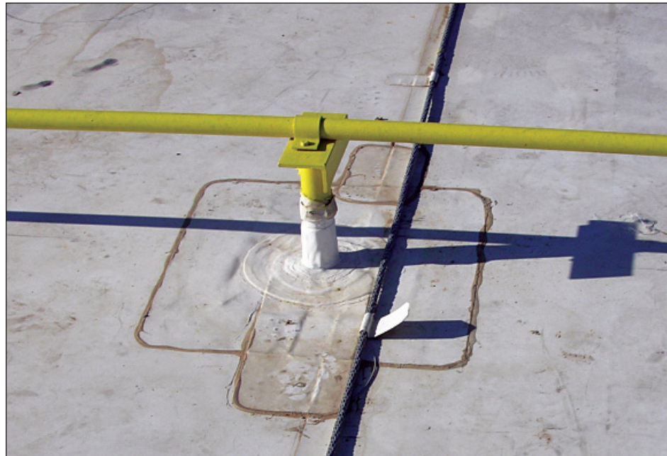
Figure 6-100: At a periodic gas line support on this roof, a steel angle was welded to a pipe that was anchored to the roof deck. A strap looped over the gas line and was bolted to the support angle. Such a connection provides resistance to lateral and uplift loads.
