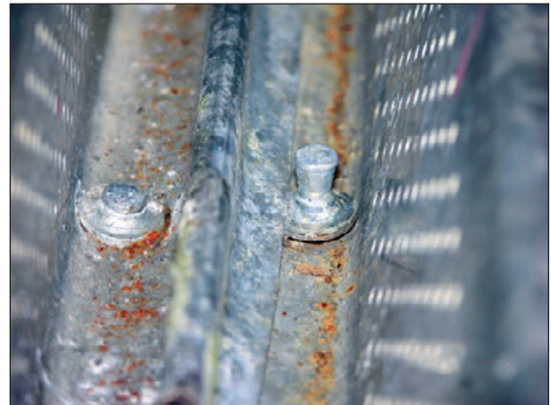
Figure 6-38: View looking along a sidelap of a deck attached with powder-driven pins. The right pin does not provide adequate uplift and shear resistance.
