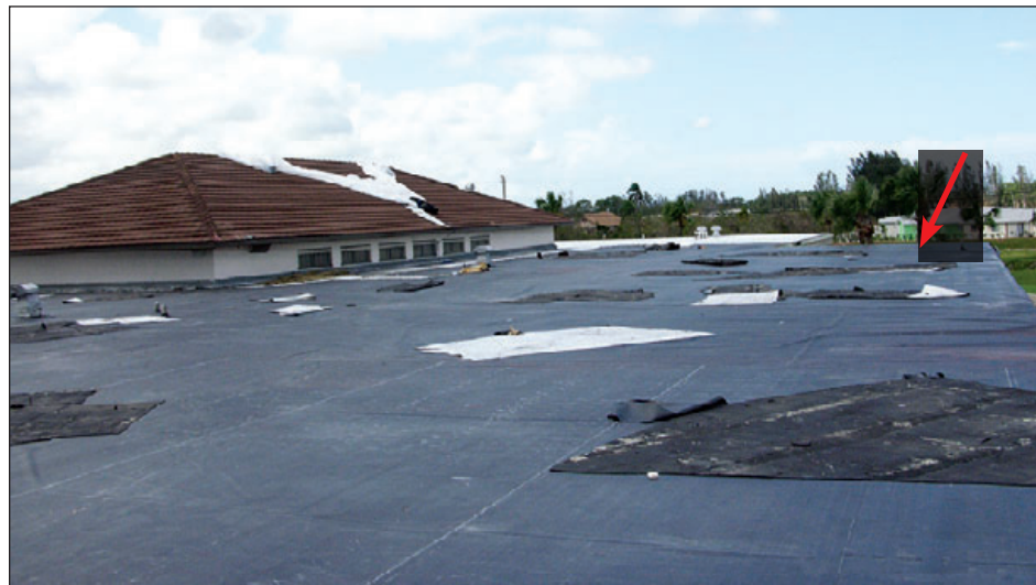
Figure 6-75: The original modified bitumen membrane was blown away after the gutter lifted in the area shown by the red arrow (the black membrane is a temporary roof). Hurricane Francis (Florida, 2004)
