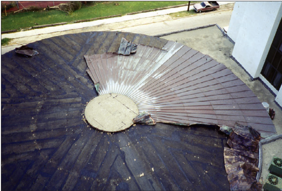
Figure 6-80: The secondary membrane prevented significant leakage into the building after the copper roof blew off. Hurricane Andrew (Florida, 1992)
