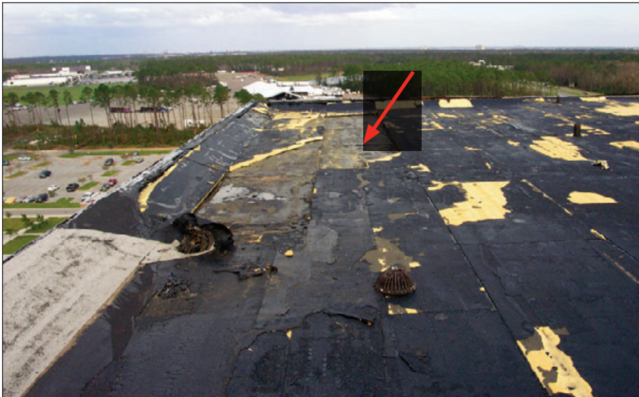
Figure 6-68: The blown off insulation (red arrow) may have initiated blow-off of the roof membrane. Estimated wind speed: 105–115 mph. Hurricane Ivan (Florida, 2004)
