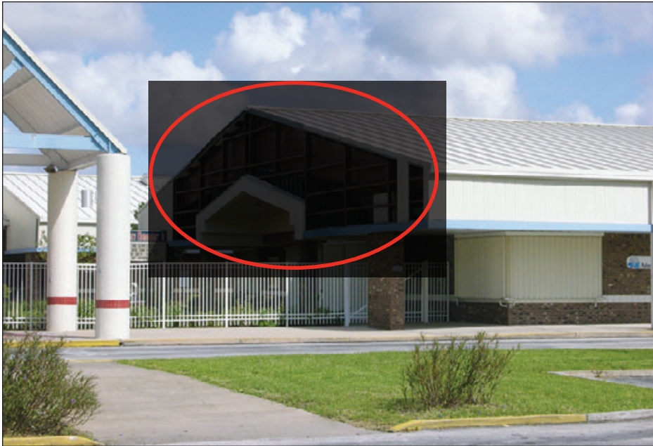
Figure 6-15: Blow-off of metal wall panels allowed wind-driven rain to enter this school. Hurricane Frances (Florida, 2004)
