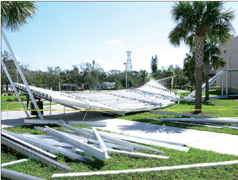
Figure 6-41: The wind speed was sufficient to collapse this school's canopy, but the speed was not high enough to blow the canopy debris very far. Hurricane Francis (Florida, 2004)
