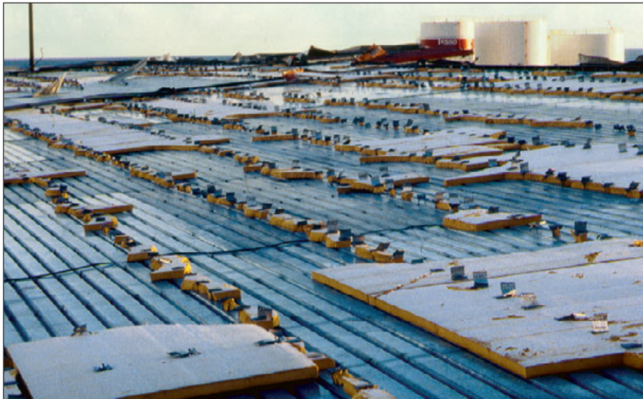
Figure 6-82: Significant interior water damage and facility interruption occurred after the standing seam roof blew off. Hurricane Marilyn (U.S. Virgin Islands, 1995)
