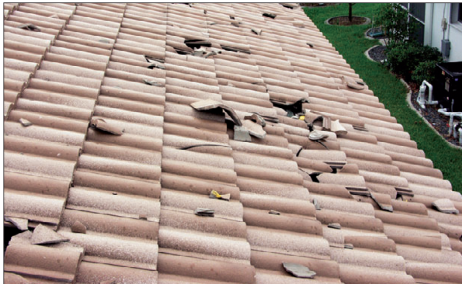
Figure 6-83: Brittle roof coverings, like slate and tile, can be broken by missiles, and tile debris can break other tiles. Estimated wind speed: 140–160 mph. Hurricane Charley (Florida, 2004)
