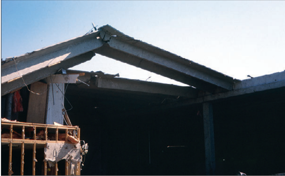
Figure 6-40: Twin-Tee roof panel lifted as a result of the combined effects of wind uplift and pre-tension. Tornado (Missouri, May 2003)
