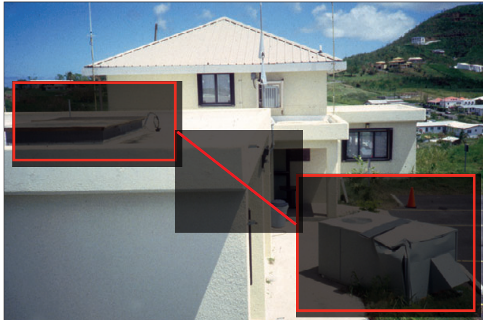
Figure 6-25: Lack of fasteners resulted in blow-off of the HVAC unit, which caused extensive interior water damage and interrupted facility use. Hurricane Marilyn (U.S. Virgin Islands, 1995)
