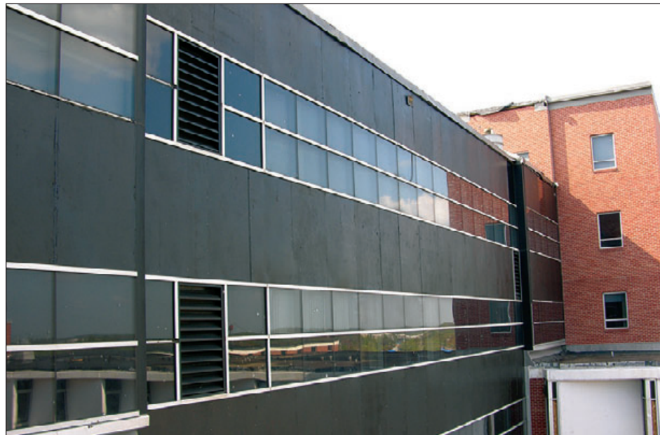
Figure 6-53: Plywood panels (black continuous bands) installed after the glass spandrel panels were broken by roof aggregate. 19 Estimated wind speed: 130 mph. Hurricane Katrina (Mississippi, 2005)
