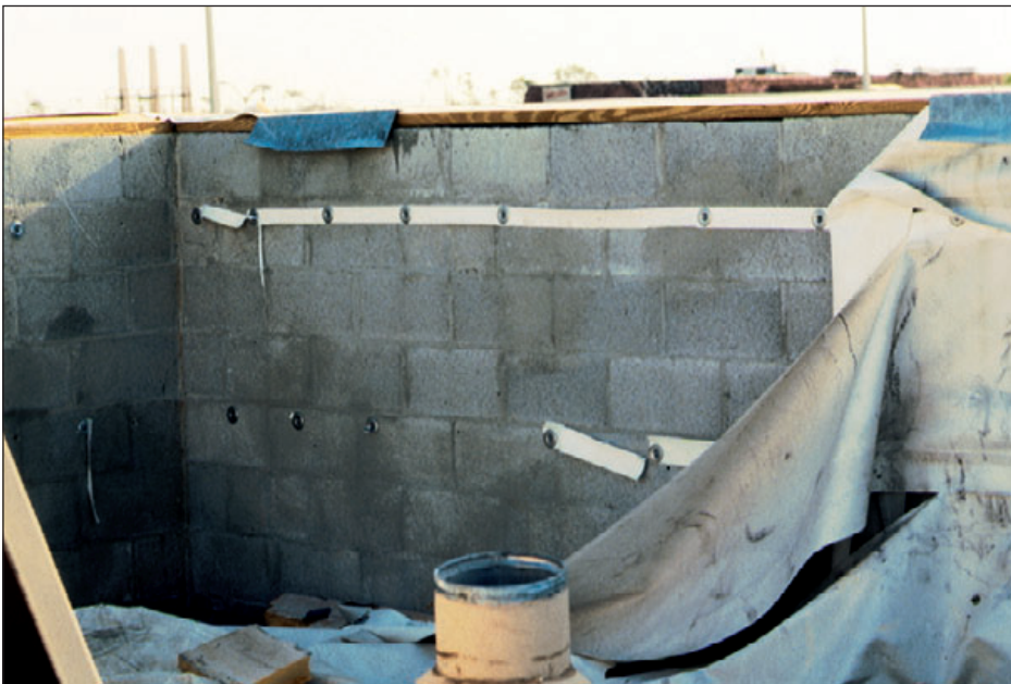
Figure 6-79: If mechanically attached base flashings have an insufficient number of fasteners, the base flashing can be blown away. Hurricane Andrew (Florida, 2004)
