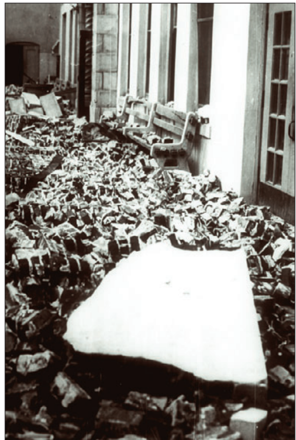
Figure 4-13: Damage to shop building, Compton Junior High School, Long Beach, CA, 1933
