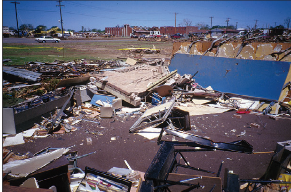
Figure 6-17: The roof and all of the walls of a wing of this elementary school were blown away by a violent tornado. (Oklahoma City, 1999)
