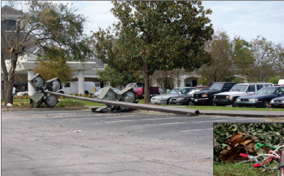
Figure 6-105: Collapsed light fixtures caused by severe corrosion (see inset). Estimated wind speed: 105–115 mph. Hurricane Ivan (Florida, 2004)
