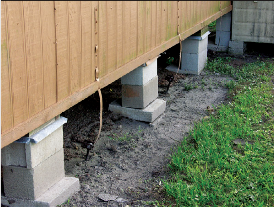
Figure 6-22: The metal straps between this portable classroom and the ground anchors were not taut. This classroom is susceptible to being blown off the piers and to overturning. See Figure 6-27 for a robust anchoring system.
