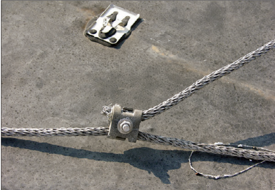
Figure 6-117: Bolted splice connectors are recommended to prevent free ends of connectors from being whipped around by wind. Estimated wind speed: 130 mph. Hurricane Katrina (Mississippi, 2005)
