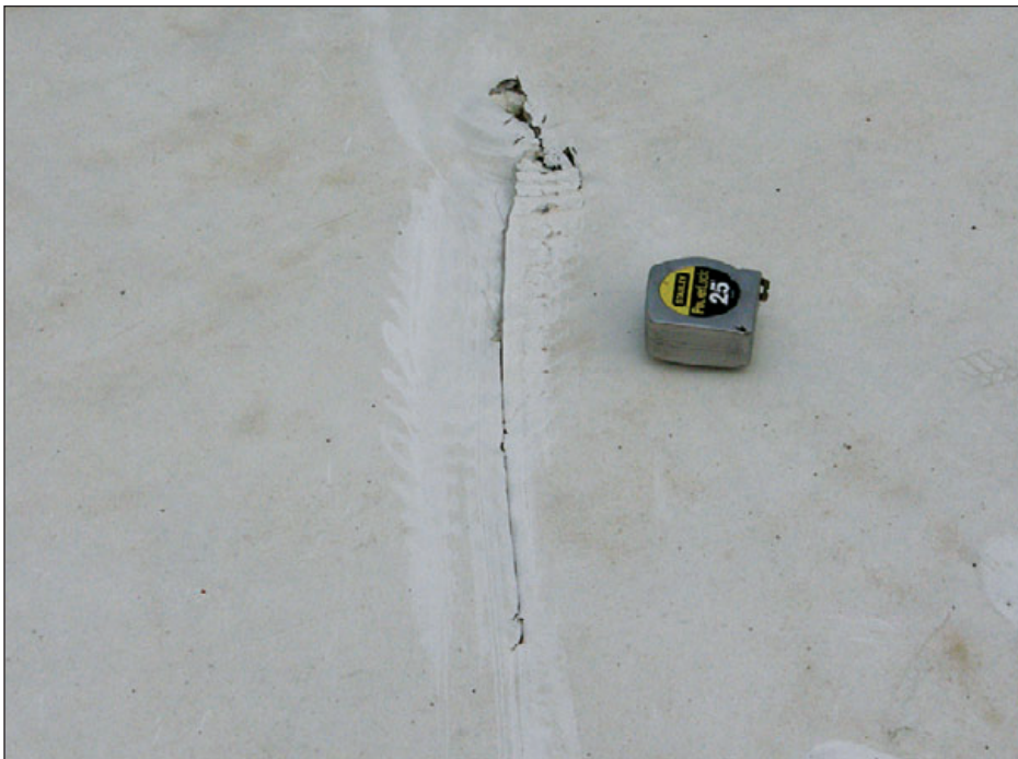
Figure 6-11: The single-ply roof membrane on this school was torn by a missile. The tear was still unprotected 6 days after it was damaged. A substantial amount of water can enter the building through such a tear, unless the deck is water tight (see Figure 6-13) or a secondary roof membrane is used as discussed in Section 6.3.3.7. Estimated wind speed: 105 to 115 mph. Hurricane Ivan (Florida, 2004)
