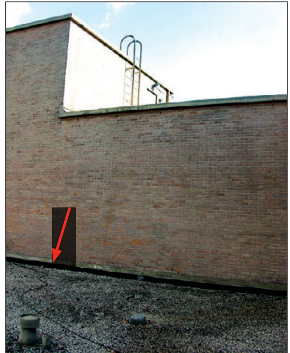
Figure 6-59: Water leaked inside along the base of the brick veneer walls (red arrow). Estimated wind speed: 115 mph. Hurricane Katrina (Louisiana, 2005)
