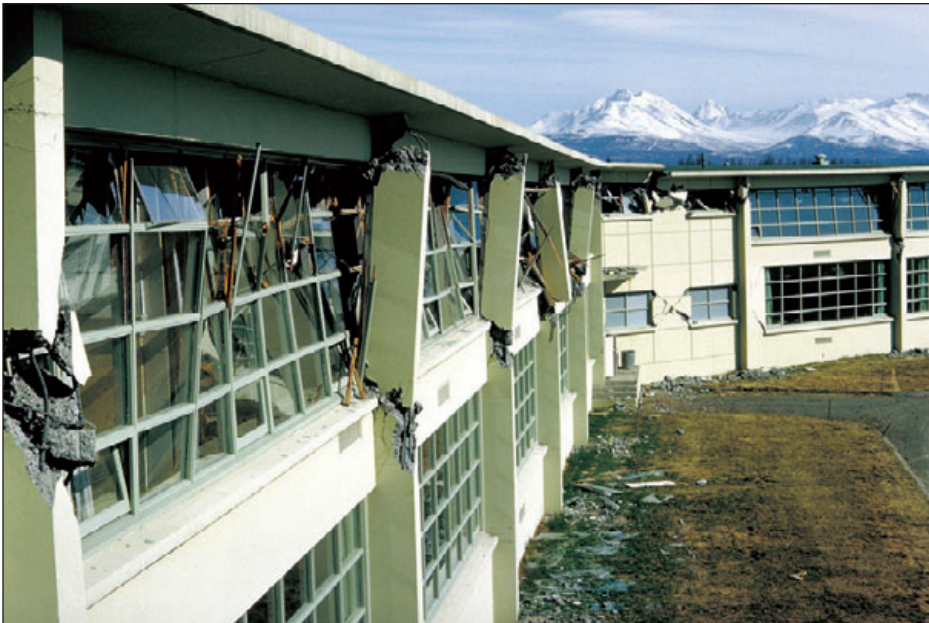
Figure 4-23: Severe structural damage to the West Anchorage High School, Anchorage, AK, 1964
