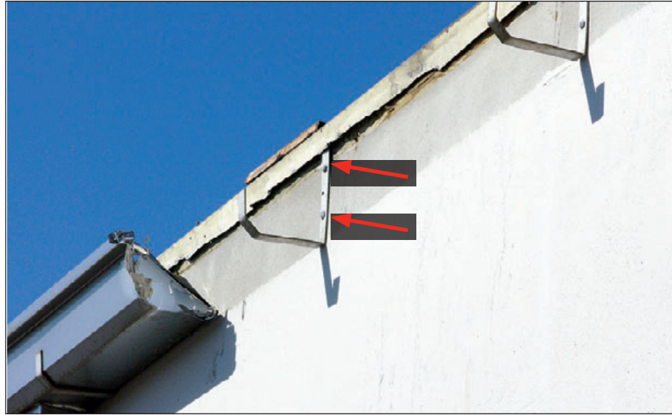
Figure 6-74: Because this gutter was not attached to the bracket, wind lifted the gutter along with the metal edge flashing that lapped into the gutter. Bracket fasteners are indicated by the red arrows. Hurricane Francis (Florida, 2004)
