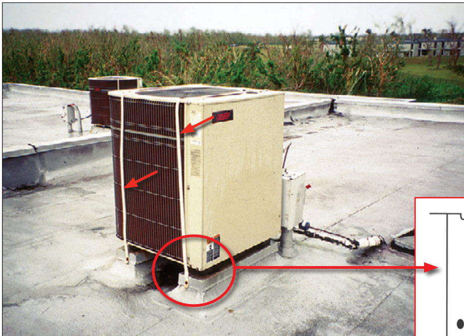
Figure 6-95: This condenser had supplemental attachment straps (see red arrows). Typhoon Paka (Guam, 1997)
