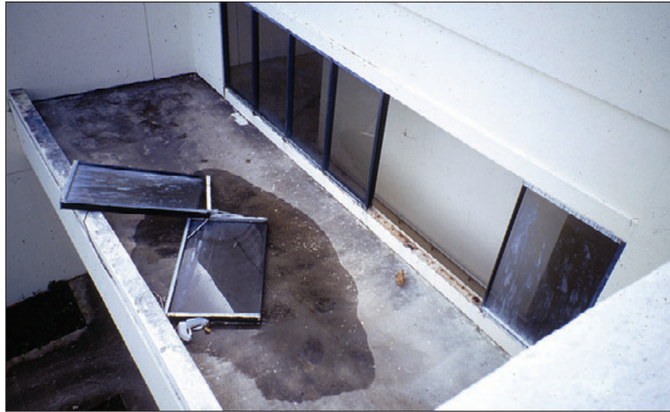
Figure 6-50: Two complete windows, including frames, blew out as a result of an inadequate number of fasteners. Typhoon Paka (Guam, 1997)
