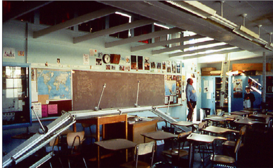
Figure 4-27: Line of suspended light fixtures fallen on teacher's station, Northridge, CA, 1994
