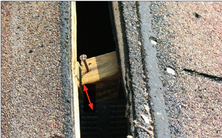
Figure 6-134: During a reroofing project a slot was cut in the plywood deck in order to allow air to flow from the attic to a new continuous ridge vent. The cutting depth of the saw was not adjusted for the thickness of the deck. The top 1½ inch of each truss and a portion of the metal nailing plate was inadvertently cut.
