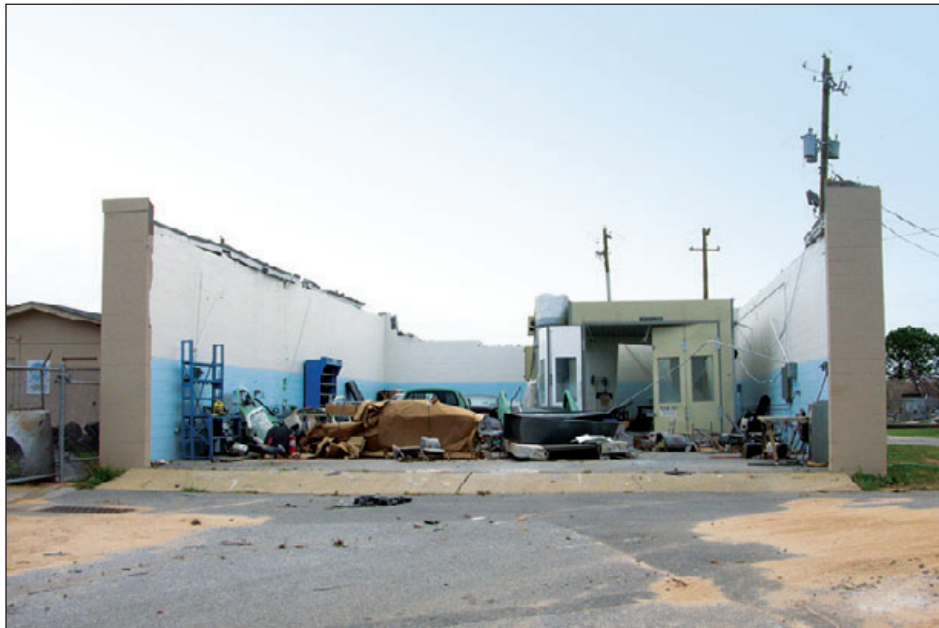
Figure 6-21: The entire metal deck and steel joist roof structure at this school's auto shop blew off. Estimated wind speed: 105 to 115 mph. Hurricane Ivan (Florida, 2004)
