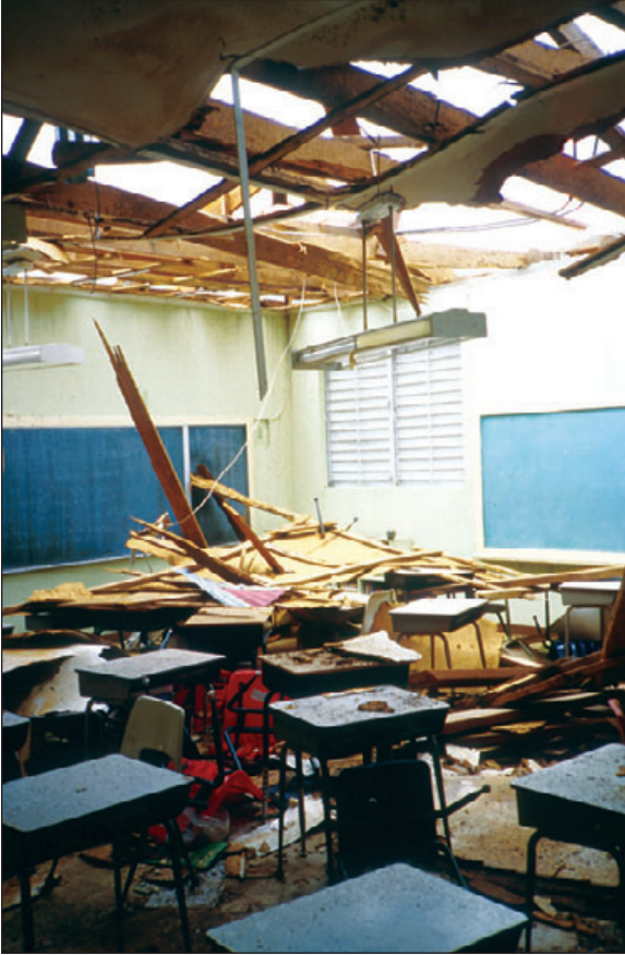
Figure 6-24: A portion of the roof structure blew off this school, and a portion of it collapsed into classrooms. Extensive water damage can cause such a school to be out of operation for a considerable period of time. Hurricane Marilyn (U.S. Virgin Islands, 1995)
