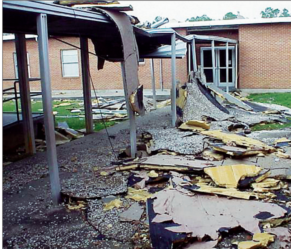
Figure 6:33: Open walkways do not provide protection from wind-borne debris. Hurricane Katrina (Mississippi, 2005).
