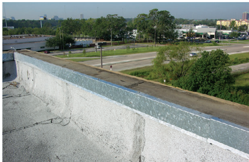
Figure 6-72: The coping blew off because of inadequate attachment of the cleats. Estimated wind speed: 92 mph. Hurricane Ike (Texas, 2008)
