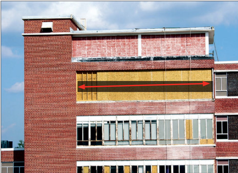
Figure 6-123: Wind pressure caused the window frames on the upper floors to fail (red arrow). Estimated wind speed: 130 mph. Hurricane Katrina (Mississippi, 2005)
