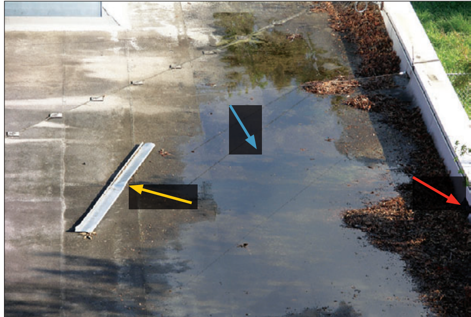
Figure 6-104: Leaf debris and ponding near a scupper (red and blue arrows). The yellow arrow indicates a piece of coping that blew off an upper roof shown in Figure 6-72. Estimated wind speed: 92 mph. Hurricane Ike (Texas, 2008)
