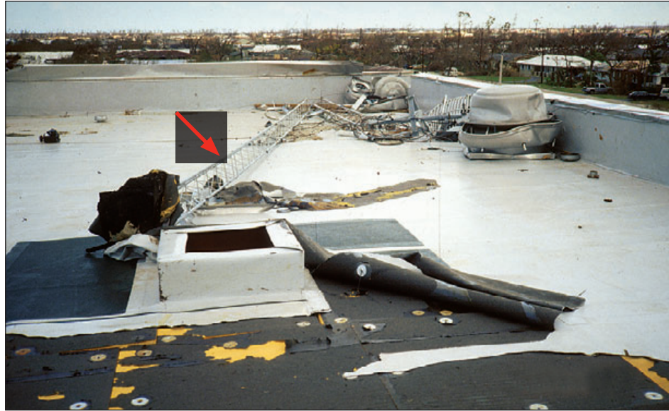
Figure 6-106: The collapse of the antenna tower at this school caused progressive peeling of the roof membrane. Also note that the exhaust fan blew off the curb, but the high parapet kept it from blowing off the roof. Hurricane Andrew (Florida, 1992)
