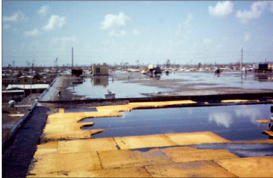
Figure 6-13: Extensive roof covering and rooftop equipment damage occurred on this school. However, the cast-in-place concrete deck kept most of the water from entering the school. Hurricane Andrew (Florida, 1992)
