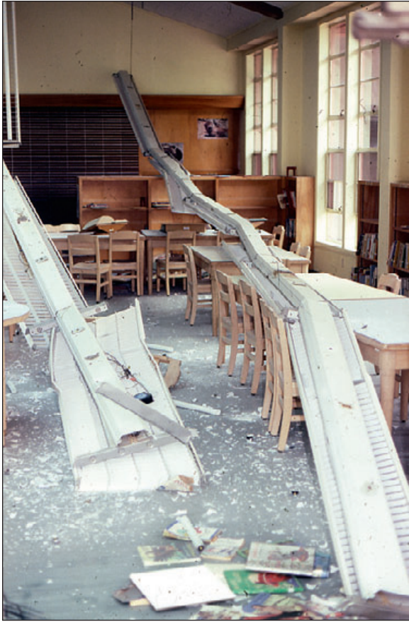
Figure 4-10: Fallen light fixtures, library, Coalinga, CA, 1983
