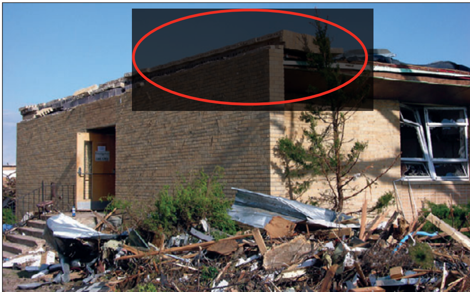
Figure 6-129: Collapsed unreinforced masonry parapet. Greensburg Tornado (Kansas, 2007)
