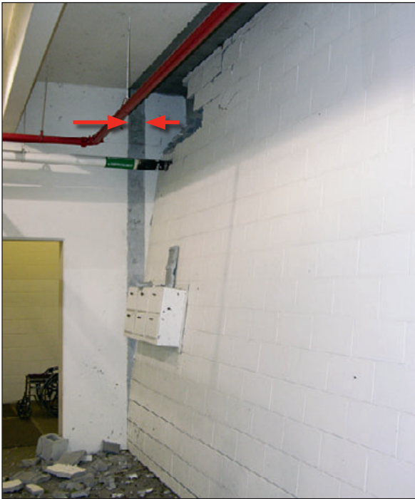
Figure 6-56: The red arrows show the original location of a CMU wall that nearly collapsed following a rolling door failure. Estimated wind speed: 140–160 mph. Hurricane Charley (Florida, 2004)
