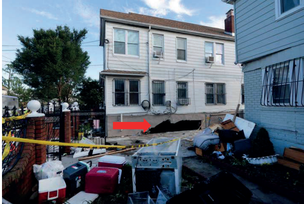
Figure 10. Failure of unreinforced masonry foundation wall at single-family home in Queens. Arrows point to a large opening in the foundation wall, as seen from the outside and inside of the building.
