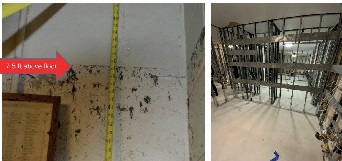
Figure 8. Water-damaged interior surfaces and interior walls in basements
