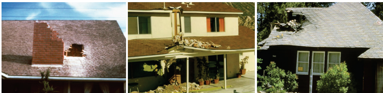
Figure 11-20 Earthquake damage to existing masonry chimneys (from R. Gallagher, National Geophysical Data Center).
