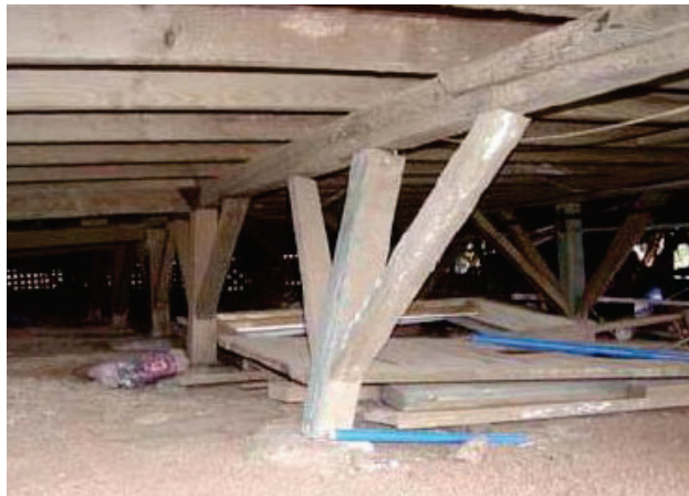
Figure 11-14 Earthquake damaged post and pier foundation (from FEMA P-530).
