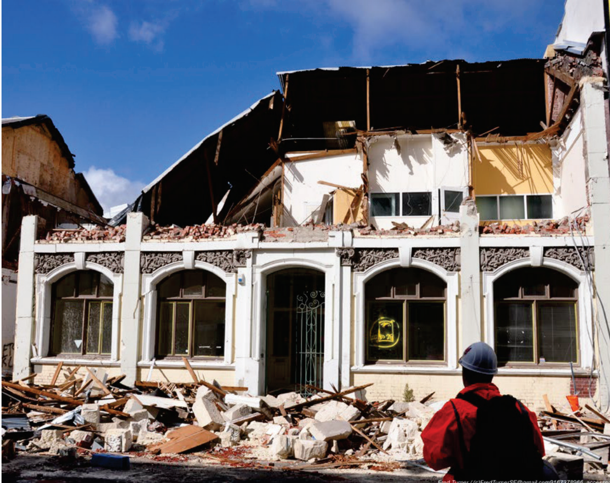
Figure 6-13 Earthquake-damaged unreinforced masonry wall structure in Christchurch, New Zealand (from Fred Turner).
