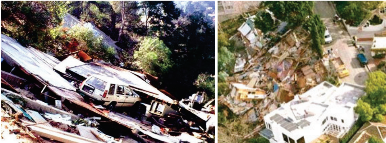
Figure 11-6 Dwellings located on hillside sites and damaged during the Northridge, California, earthquake (from FEMA P-530).
