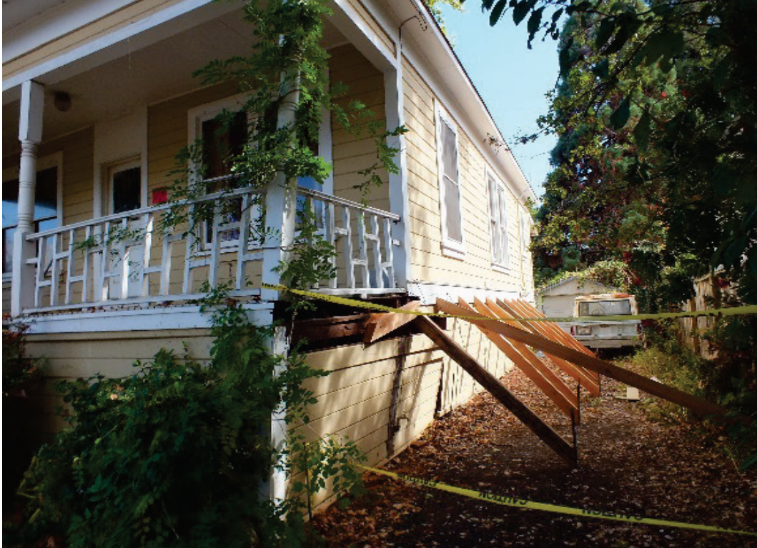
Figure 2-22 Cripple wall failure in the 2014 South Napa Earthquake (from FEMA P-1024).
