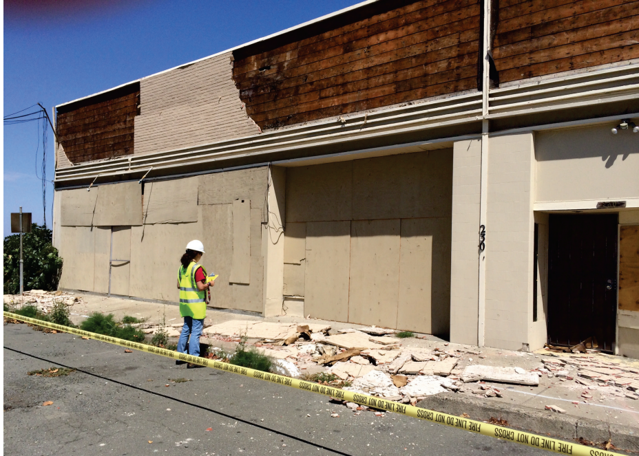
Figure 7-3 Veneer damage in the 2014 South Napa Earthquake (from L Whitehurst, EERI Learning From Earthquakes).
