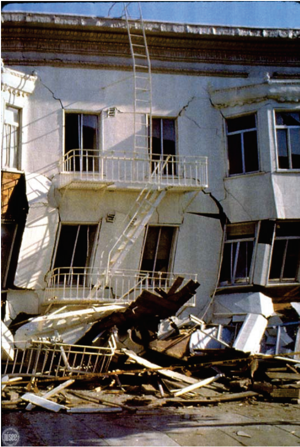
Figure 2-21 Multi-family housing with soft story failure in the 1989 Loma Prieta Earthquake (from NISEE).
