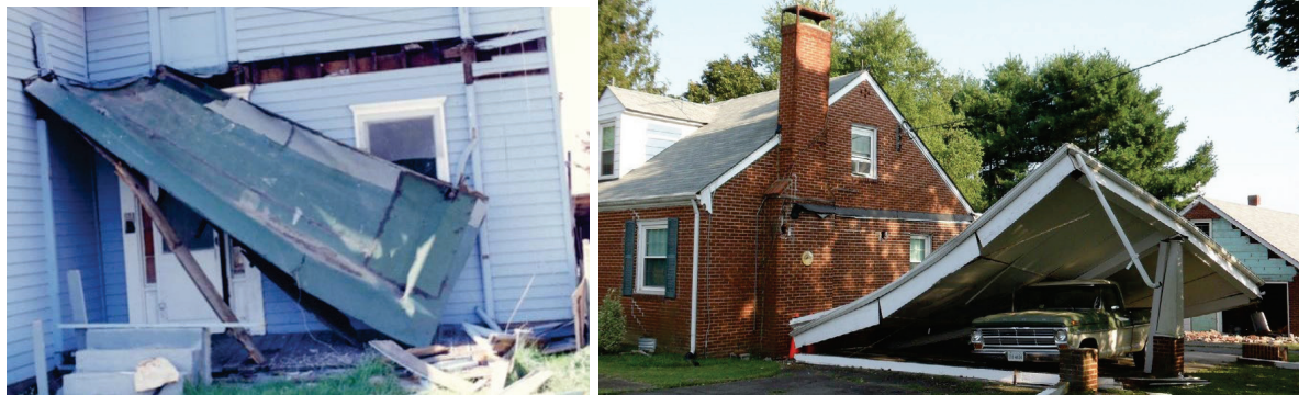
Figure 11-22 Earthquake damage to elevated decks and carports (from R. Gallagher, R. Green).
