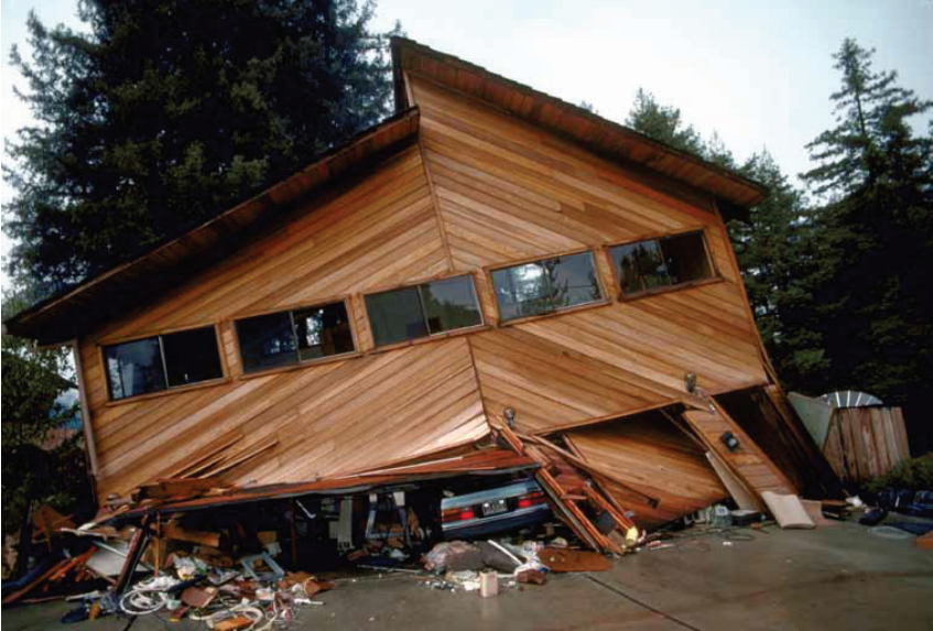
Figure 2-20 House experiencing soft- and weak-story behavior in the 1989 Loma Prieta Earthquake (from USGS).
