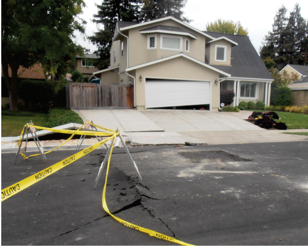
Figure 2-5 A dwelling damaged due to fault movement in the 2014 South Napa Earthquake. (from Geotechnical Extreme Events Reconnaissance, GEER).
