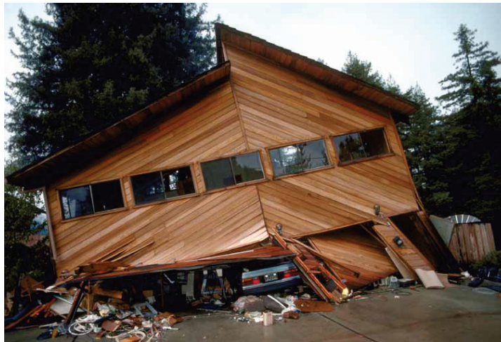
Figure 11-10 Damage to living-space-over-garage dwellings in the 1989 Loma Prieta Earthquake (from USGS).
