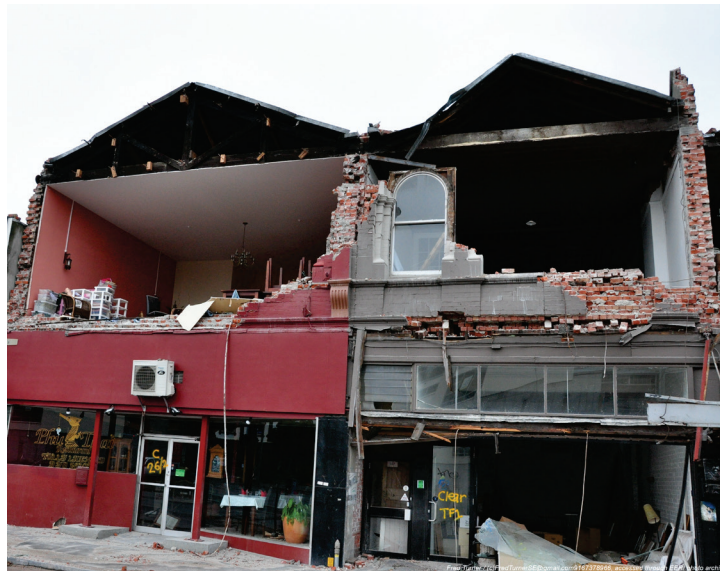
Figure 11-16 Earthquake-damaged unreinforced masonry wall structure in Christchurch, New Zealand (from Fred Turner, EERI Learning From Earthquakes).
