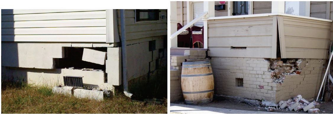
Figure 11-18 Earthquake damage to unreinforced masonry foundations in the 2011 Mineral, Virginia Earthquake (left) and 1994 Northridge Earthquake (right) (from FEMA P-530).
