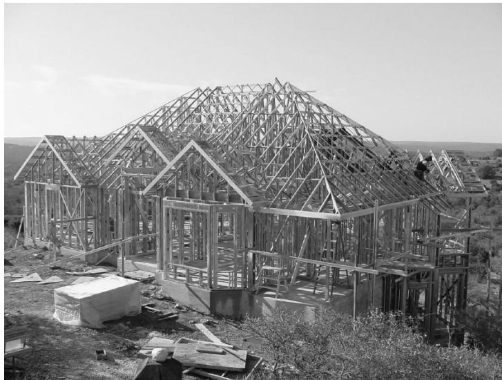
Figure 6-11 Cold-formed steel house under construction (from Dietrich Metal Framing – a Worthington Industries Company).
