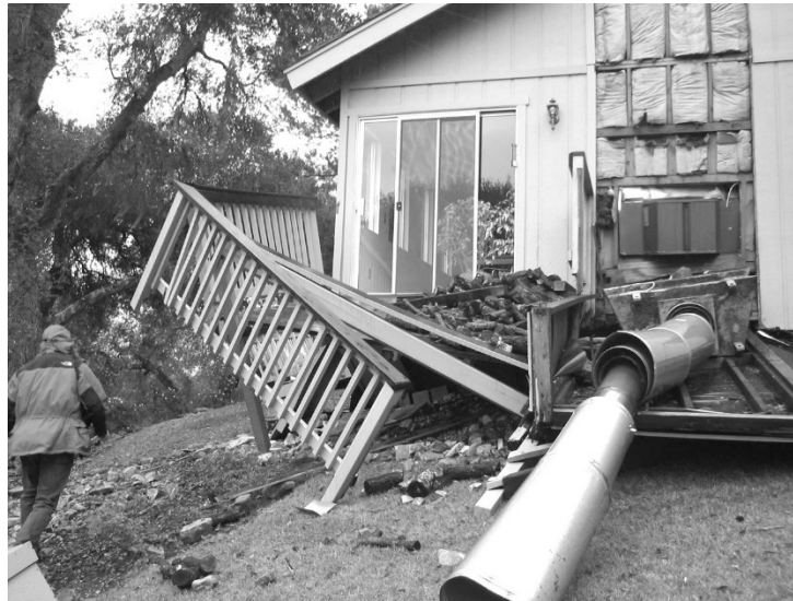
Figure 9-7 Collapsed factory-built chimney, light-frame enclosure, and deck after the San Simeon Earthquake (from J. Marrow).
