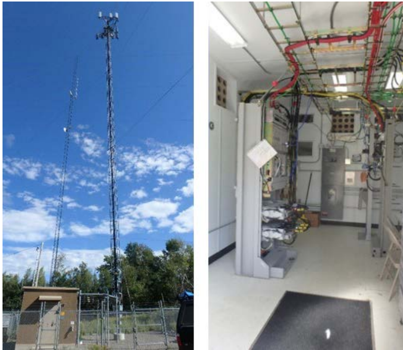
Figure 4.4.4. Exterior and interior of an equipment shelter.
