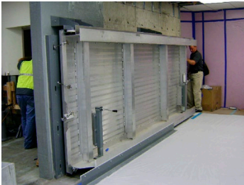
A flood door is an example of dry floodproofing a building.
