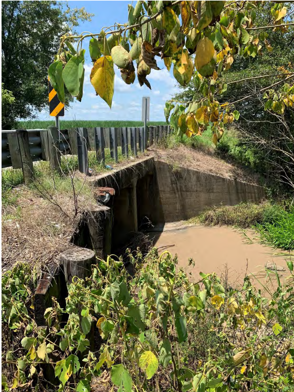
Figure 6. North detail of the bridge at the LA Hwy 983 (West Bueche Road) crossing where slope stabilization measures will be applied.
