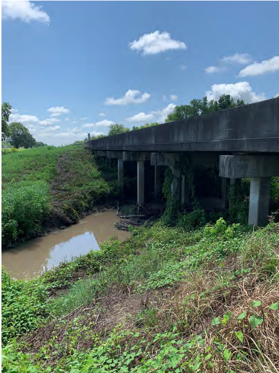
Figure 10. North detail of the bridge at the US Hwy 190 crossing where slope stabilization measures will be applied.
