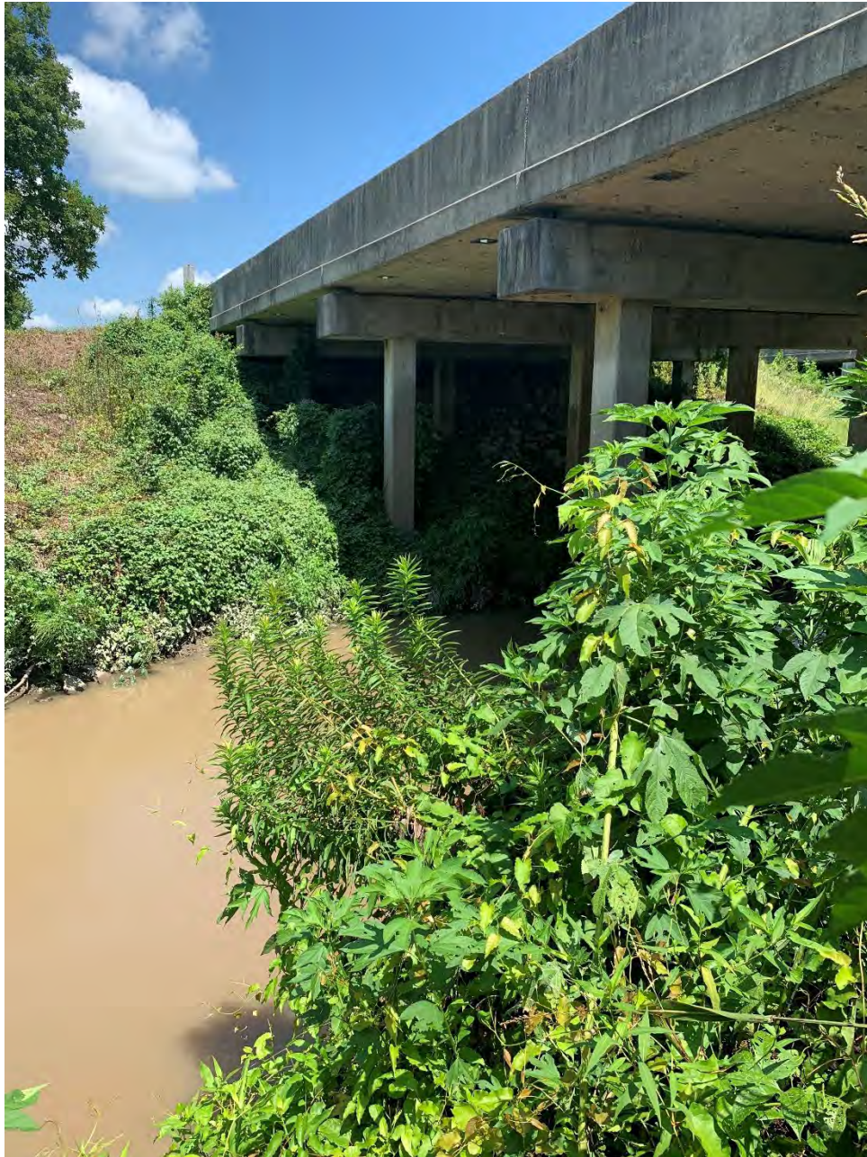
Figure 11. South detail of the bridge at the US Hwy 190 crossing where slope stabilization measures will be applied.
