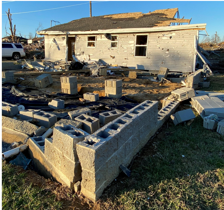
Figure 1. Failure of load path, building envelope components (roof shingles, soffits, and siding) and windows observed in Dawson Springs, Kentucky (December 2021)
