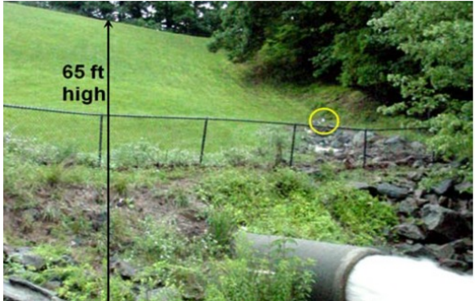
Lake Needwood Dam Seepage Incident
