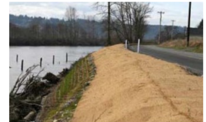
Figure 1. A photo of a soil stabilization project along a riverbank below a roadway.
