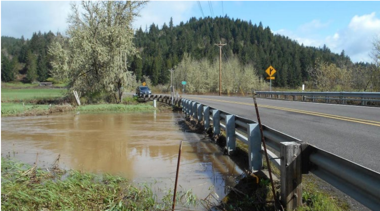
Figure 5: View of the existing north bridge (04057A) that traverses Coyote Creek during a flood event in April 2019
