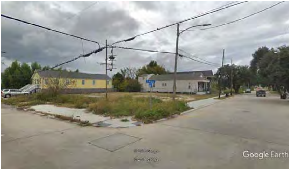
Figure 10. View of Stormwater Lot 2, 3200 Jackson Ave. (Google Street View 11/2018), looking northwest. Scope of work includes demolition/replacement of concrete sidewalk and curb; excavation of property; construction of surface retention ponds, new catch basins, two concrete runnels and footbridges; and installation of plant material. This area is not within an a NRHP listed/eligible historic district.
