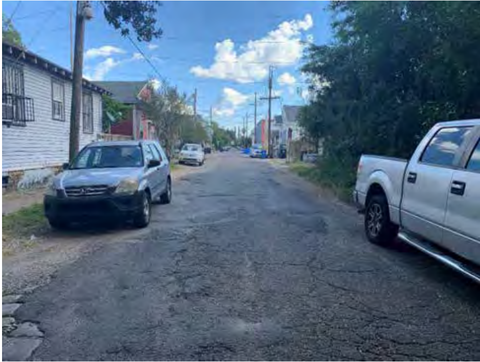
Figure 19: Typical conditions of Saint Thomas Street, as seen from its intersection with Washington Street, where the road reconstruction with bioswales is proposed
