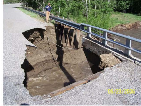
Damage to bridge from flood.
