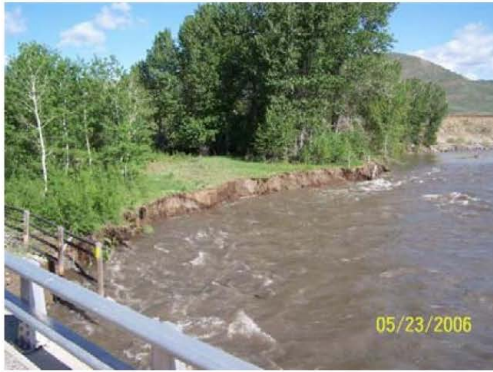
Flooding along west bank, looking north of bridge.
