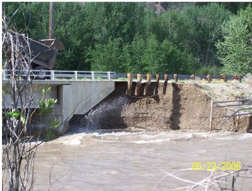
Looking south towards bridge. Hanging guardrails mark damaged section of bridge (see top right photograph).
