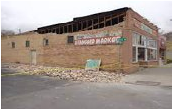
Earthquake Damage from Unreinforced Masonry
