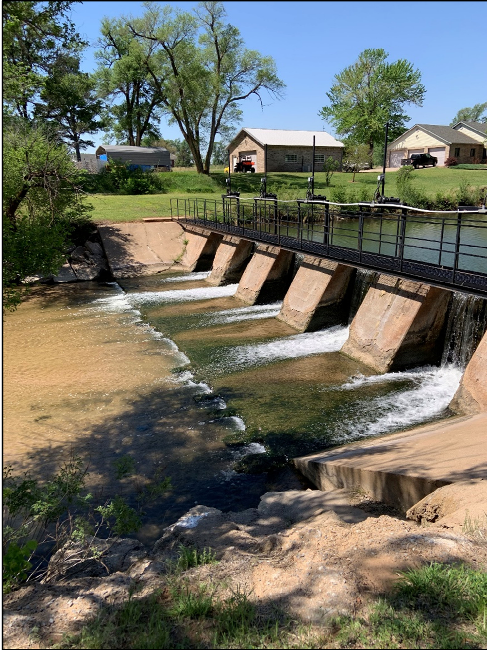
Mill Race Dam (ca.1933) view to southwest Image date: 9 May 2022 FEMA EHP staff photograph
