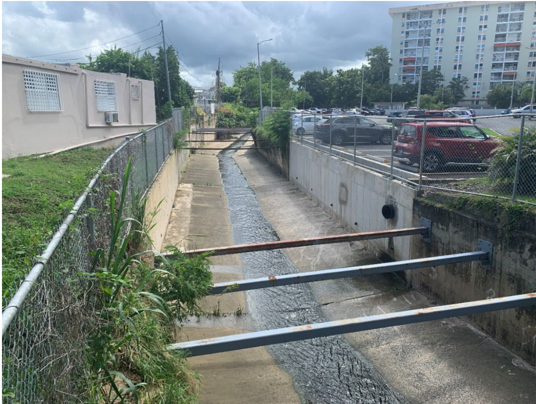
Figure 1-3: Trapezoidal channel concrete walls failing along the Quebrada Buena Vista Stream, between the Jardines Metropolitanos residential building complex and the Ramón Nevarez community in San Juan. (2023).
