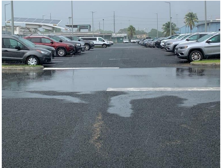
Figure 2-7. Permeable parking lot at the GSA Guaynabo Center after an afternoon rain, showing the water slowly infiltrating into the pavement, recharging the groundwater and reducing runoff at the site. Wet area corresponds to standard pavement placed to sustain more intense traffic, while the remaining parking lot was covered with permeable pavement.
