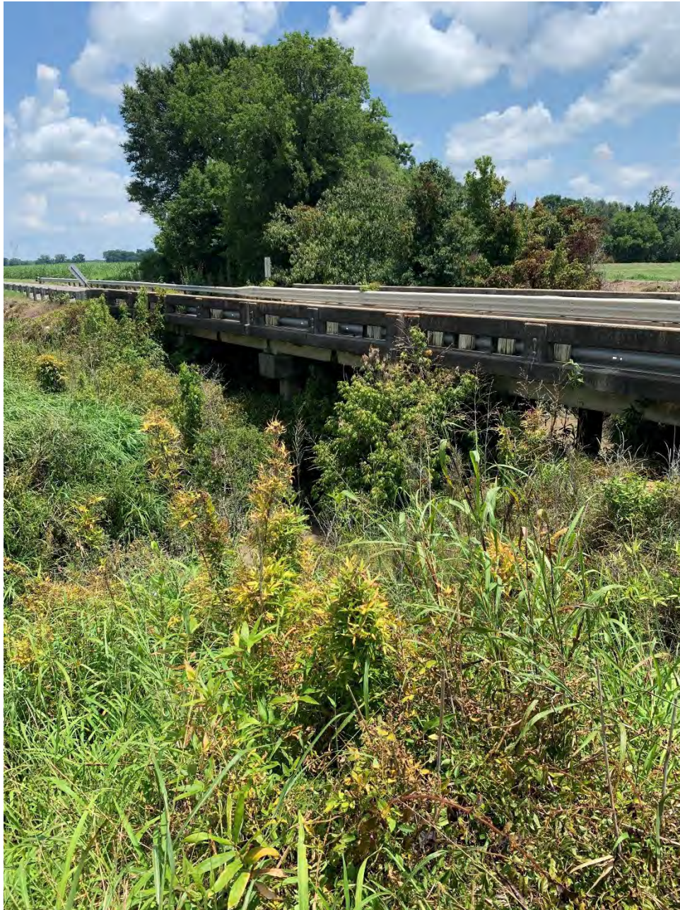
Figure 8. West detail of the bridge at the LA Hwy 984 (Rougon Road) crossing where slope stabilization measures will be applied.
