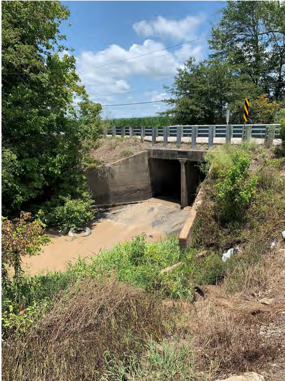
Figure 7. South detail of the bridge at the LA Hwy 983 (West Bueche Road) crossing where slope stabilization measures will be applied.
