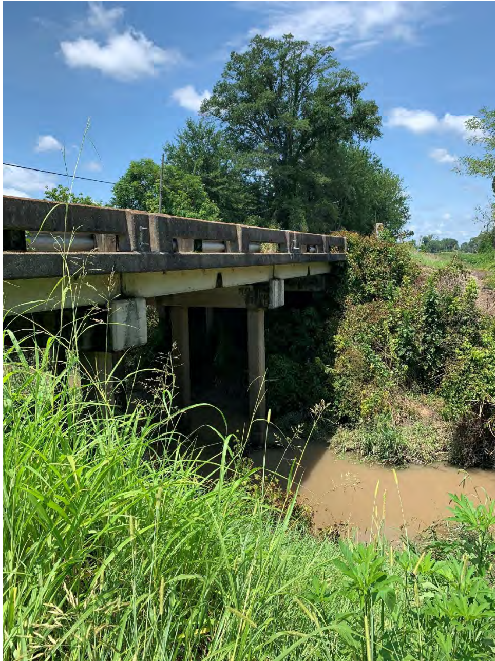
Figure 9. North detail of the bridge at the LA Hwy 620 (Section Road) crossing where slope stabilization measures will be applied.
