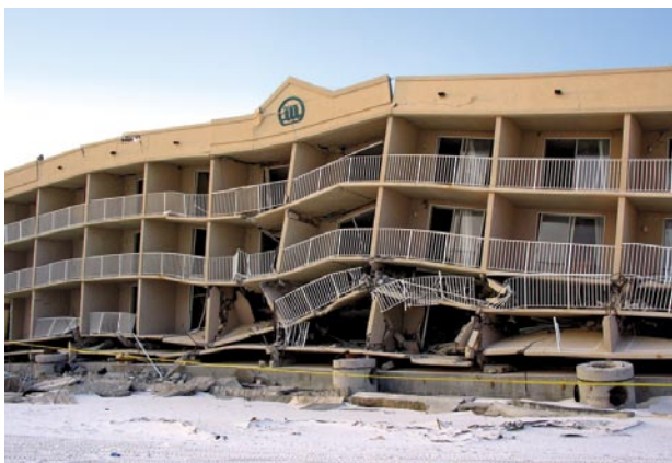
A multi-family condominium collapsed after Hurricane Ivan due to erosion of supporting soil under the shallow foundation.
