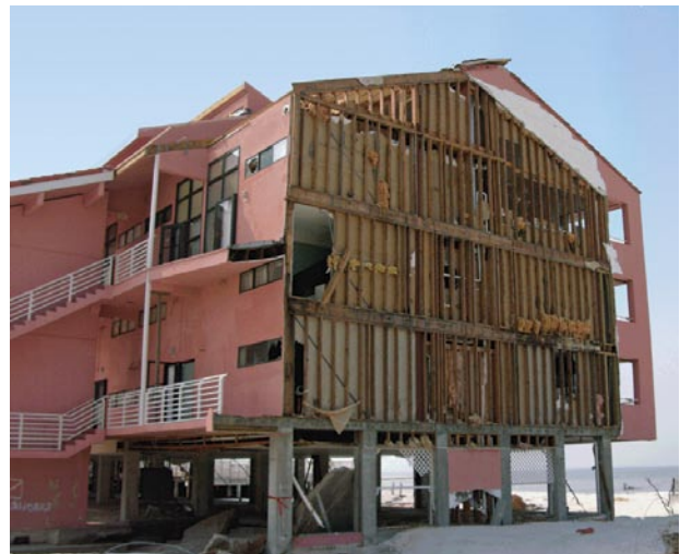
Example of wall cladding failure. The building had synthetic stucco installed over molded, expanded polystyrene insulation and gypsum board. The gypsum board blew off during Hurricane Ivan.
