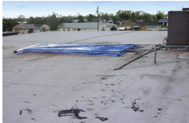
A large HVAC package unit was blown off this curb during Hurricane Charley. Note the loose LPS conductors this side of the curb. This school had significant damage from several pieces of rooftop equipment that blew off the building roof. (Port Charlotte Middle School)
