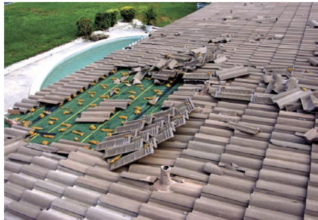
In addition to the damage shown in this photo, this one-story roof lost virtually all of the hip and ridge tiles during Hurricane Charley. (Punta Gorda Isles)
