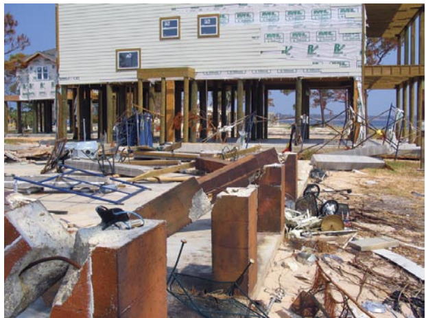
High flood levels during Hurricane Ivan and lack of structural capacity to withstand waves and debris loads caused this reinforced pier foundation to fail.
