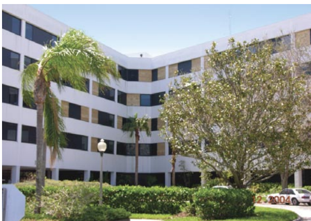
Aggregate from the Indian River Memorial Hospital's roof (Vero Beach) broke several of the patient room windows (which were covered with plywood after Hurricane Frances).
