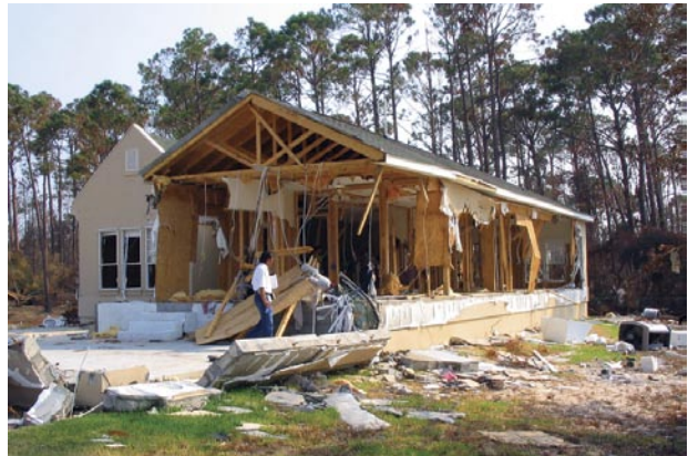
Flood water from Hurricane Ivan exceeded the required elevation of the top of the lowest floor supported by the stem wall foundation for this house leading to severe damage caused by waves and debris impact.
