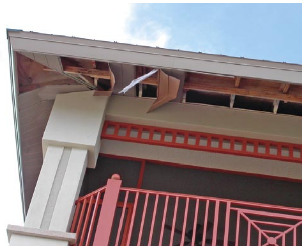
Soffit damage on the third story of a multi-family building. (Captiva Island)
