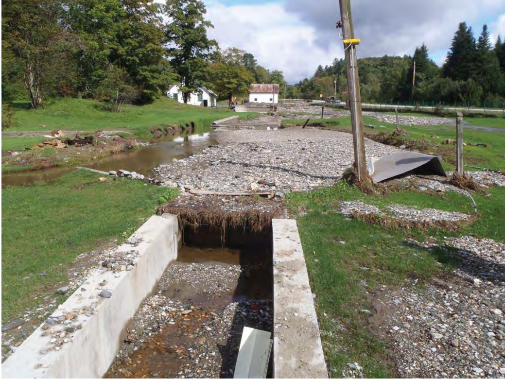
The Raceway and Pond #4 (looking north) immediately after Tropical Storm Irene
