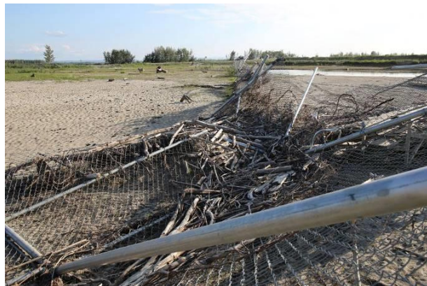
Figure 2. The fence running along the Galena ball field sits ruined after the floodwaters receded.
