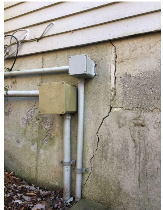
Figure 1. A crack in a home's foundation caused by pyrrhotite in the concrete.
