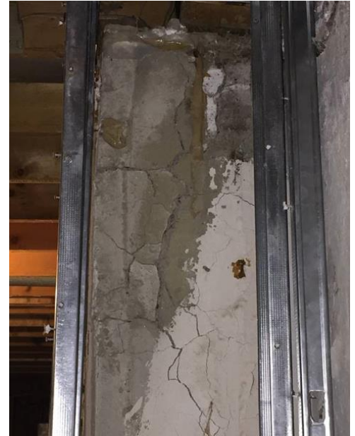
Figure 3. A crumbling foundation caused by the presence of pyrrhotite.
