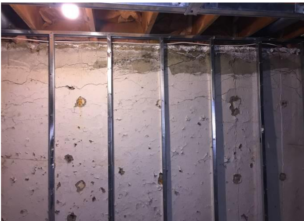
Figure 2. A crumbling foundation due to pyrrhotite in the concrete.
