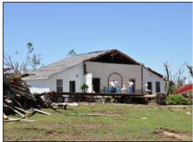
Figure 6: Remaining Portion of Ebenezer Baptist Church, Holmes County, MS, EF-3, 145 mph
