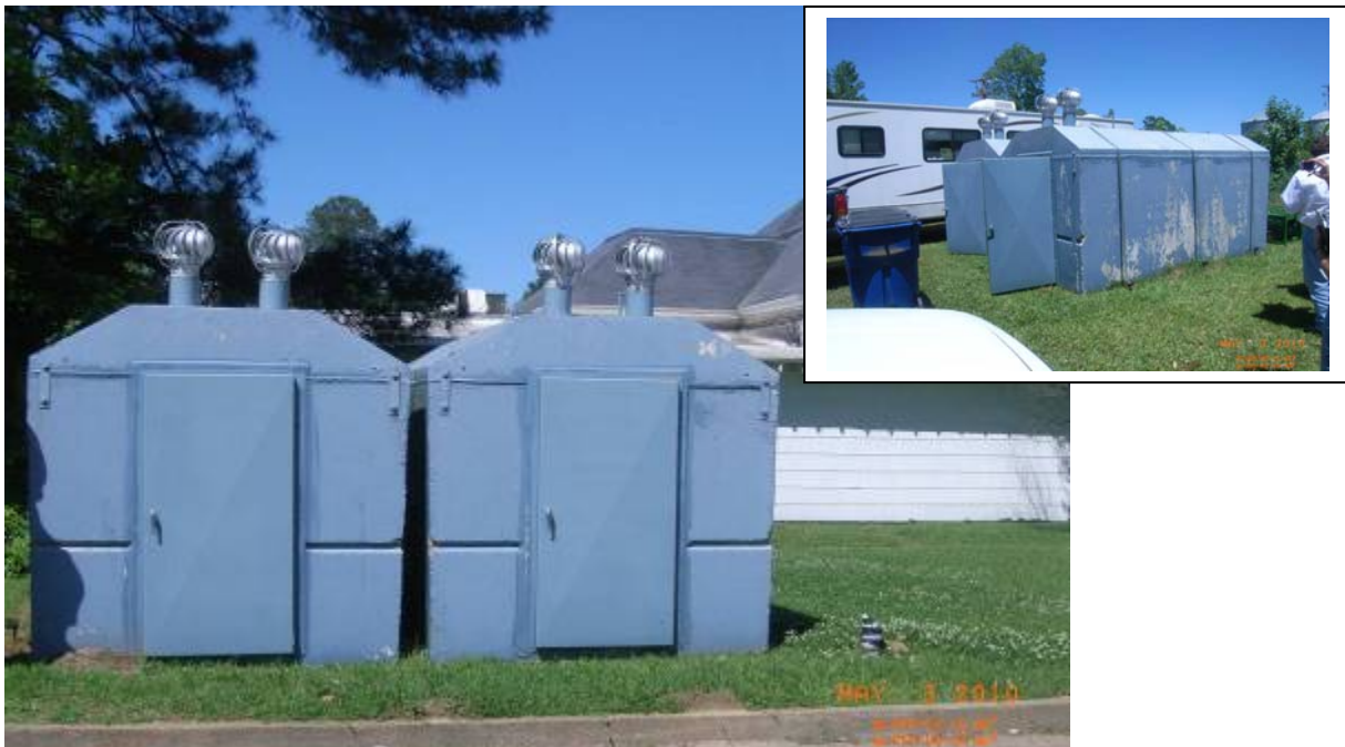
Figure 21: Durant Police Station (Left) and Ebenezer Fire Department (Top Right), Holmes County, FEMA 361 Community Safe Rooms
