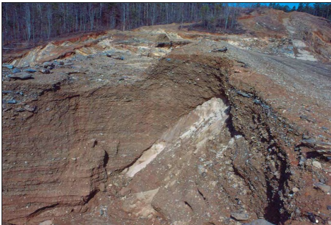
Figure E-4. View toward right abutment showing remnant of chimney filter/drain in cross-sectional view. Chimney filter/drain was 3 ft wide.
