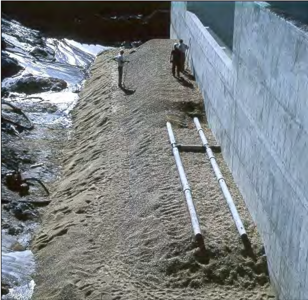
Figure 2-7. Filter and drainage zones to provide pressure relief and drainage of backfill next to training wall for a spillway chute. One individual is standing on top of the sand layer (Photo courtesy of NRCS, Texas).
