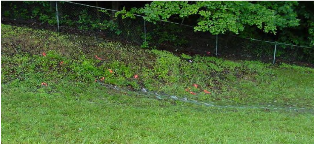
Figure L-26-1. Water discharging in the groin area downstream of an embankment during higher than normal reservoir storage. Seepage was through bedrock in the foundation that was not grouted. A gravel drainage layer was placed over the seepage to provide a controlled outlet. The seepage was not carrying fines, which would have been problematic to deal with because a fine filter would be required to block the fines but a coarse filter was required for capacity. In this case, the gravel layer provided a collector mechanism, with no filtering being required.
