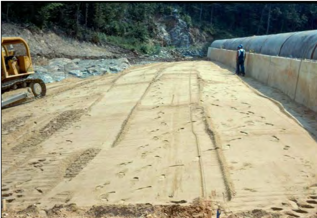
Figure 2-11. Fine filter placed over gravel blanket drain shown in Figure 2-10. (Photo courtesy of NRCS, Alabama.)
