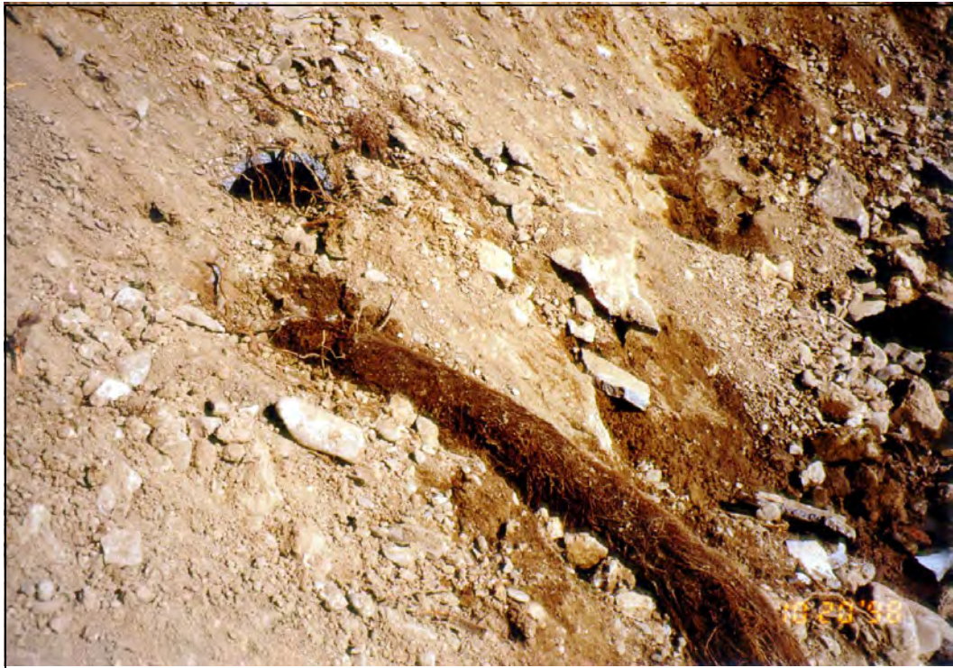
Figure 2-19. During modification of a dam, this toe drain pipe was exposed during excavation. The pipe was completely clogged with the root ball shown in the foreground. It was noted that a tree was growing over the toe drain, and the drain was probably the water source in this arid region of central Oregon.
