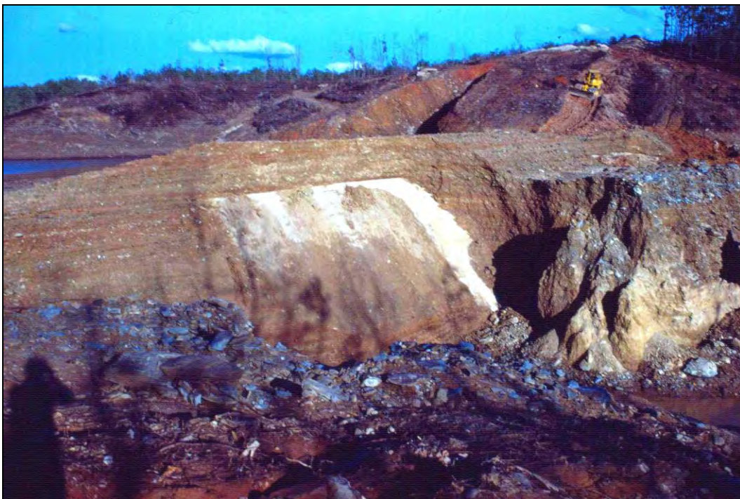
Figure E-6. Breached portion of dike in left abutment viewed upstream. The lighter color is remnant of a chimney filter.
