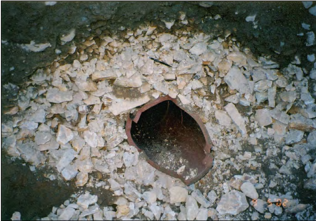
Figure 2-16. Clay tile pipe surrounded by gravel-size material. Note mechanical pencil for scale. Surrounding the gravel is a mixture of silt and sand backfill that does not meet filter criteria for the gravel. Seepage enters the pipe through joints between pipe segments. The silt and sand can erode through the gravel backfill and enter the pipe through the joints.
