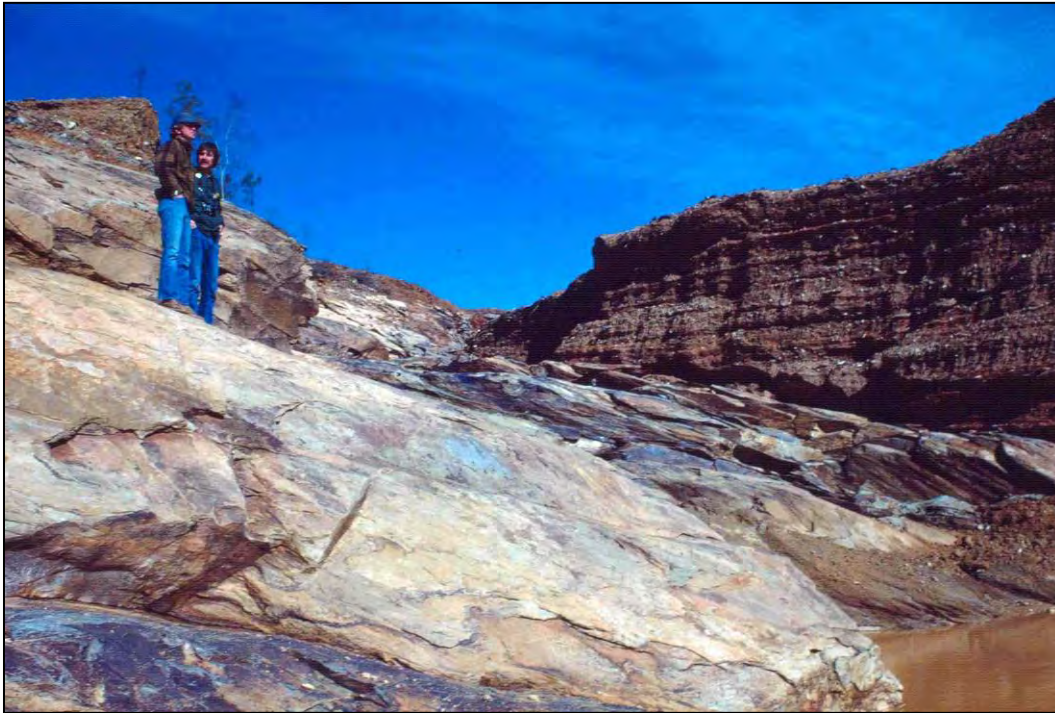
Figure E-5. Closeup of right abutment viewed upstream. Bedrock was cleaned by erosion from overtopping flow. Embankment is in top right of photograph.
