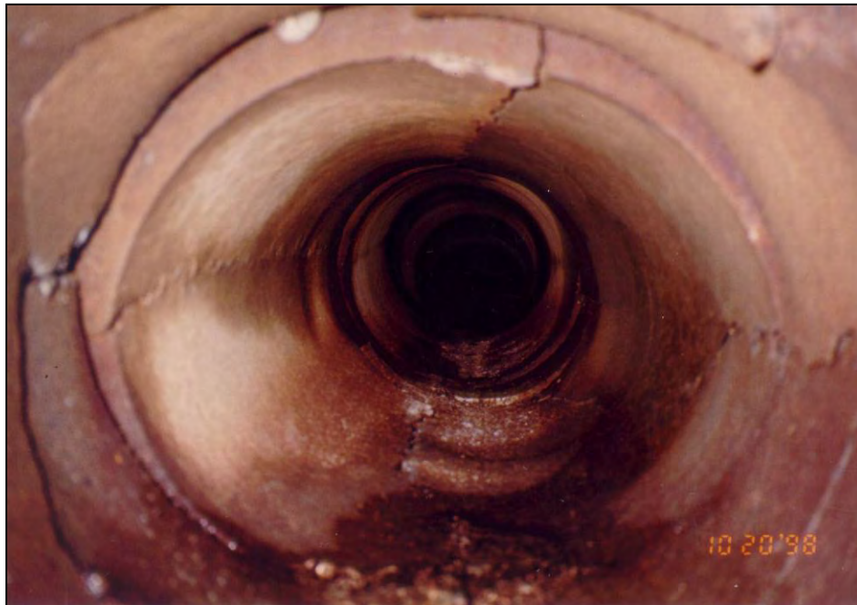
Figure 2-17. Interior view of a reinforced concrete pipe from the 1950s. Note that the pipe is overstressed, and cracks have formed at the crown and spring line. The pipe has also deformed to an oval shape. In the foreground, a joint can be seen and sand that passed through the joint.
