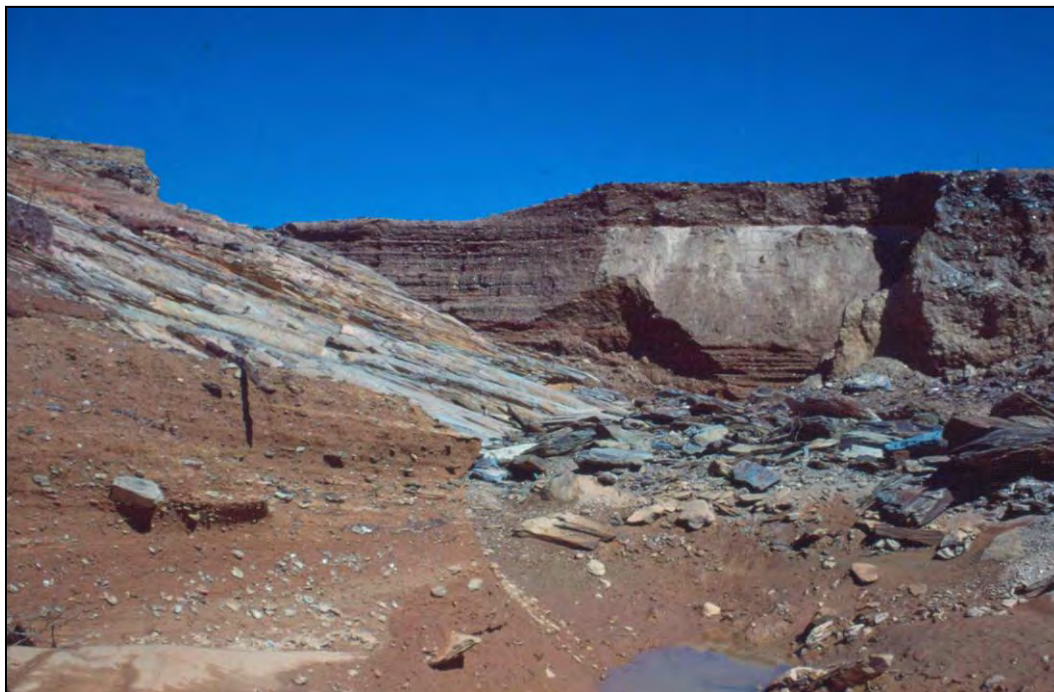
Figure E-3. Breach in left abutment viewed in upstream direction. Right abutment is to left foreground. Overtopping flow washed the embankment and overburden down to clean rock.
