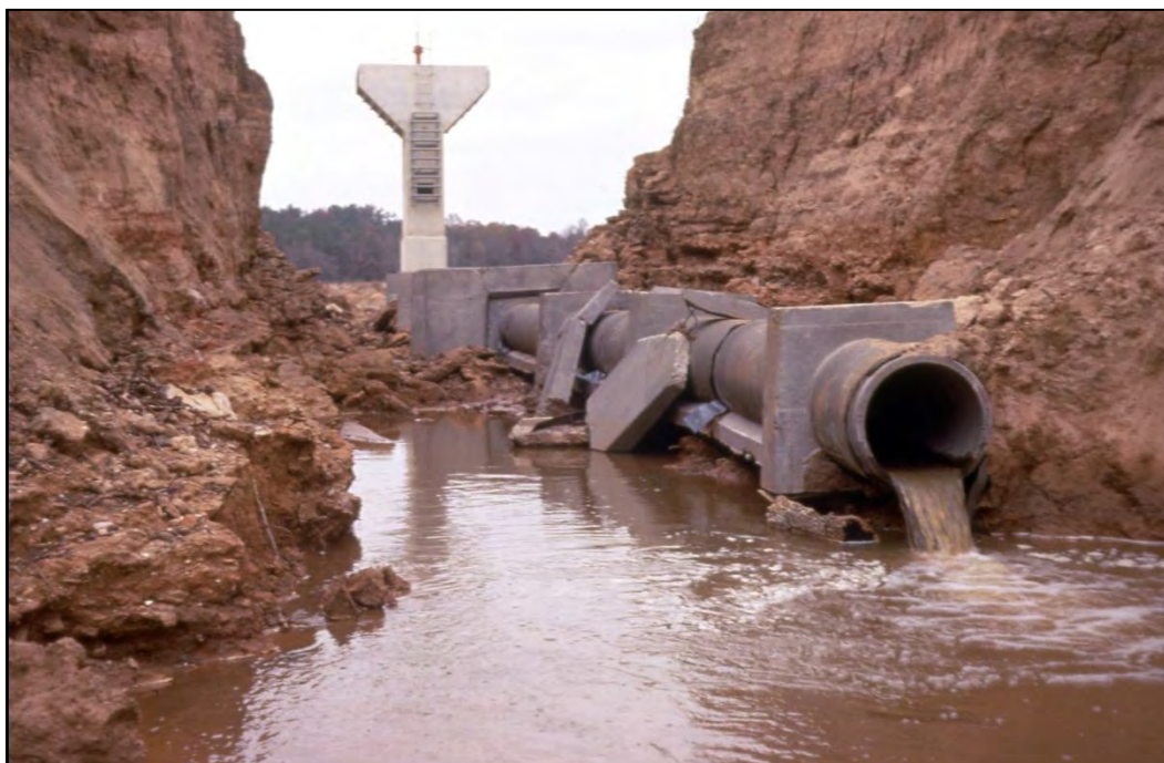
Figure 2-5. Embankment dam breached after piping along the conduit. The view is upstream. Note pre-cast concrete pipe placed on a concrete cradle and the use of seepage collars (Photo credit NRCS).
