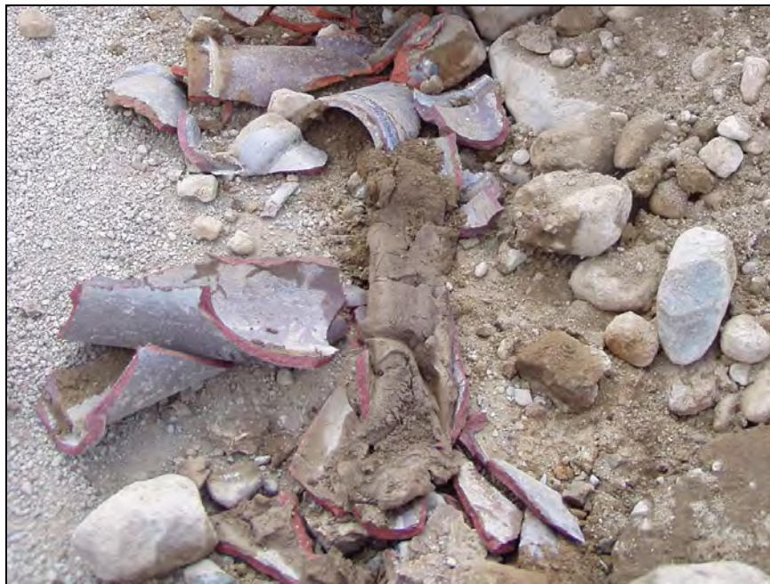
Figure 2-18. Clay tile pipe from 1916 as it was exposed during excavation. Note that the pipe was completely clogged with silt and sand.
