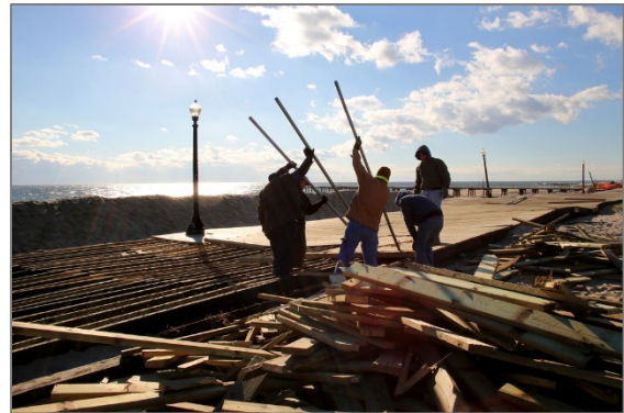
The Calvary Chapel Relief volunteers, an organization, works tirelessly to remove damaged boards from the Asbury Park boardwalk after Hurricane Sandy.
