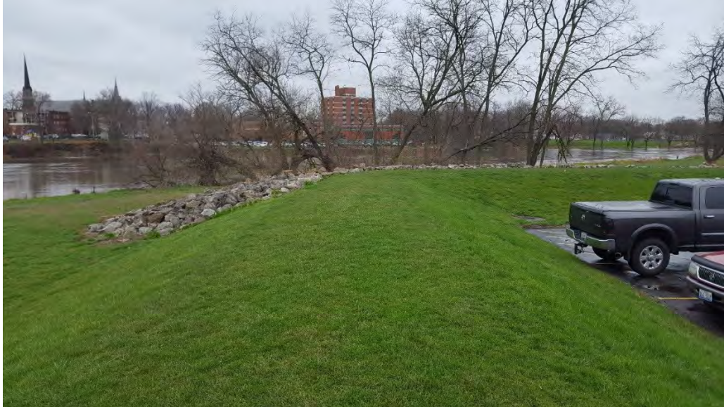
Photo 7: View Northwest toward the Fox River along existing levee and riprap adjacent to the OTHS parking lot north of Main Street.
