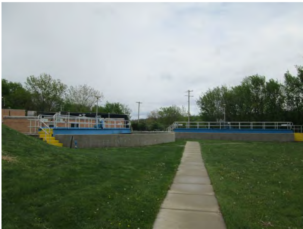
Photo 24: View southeast to c. 1974 Secondary Clarifiers.
