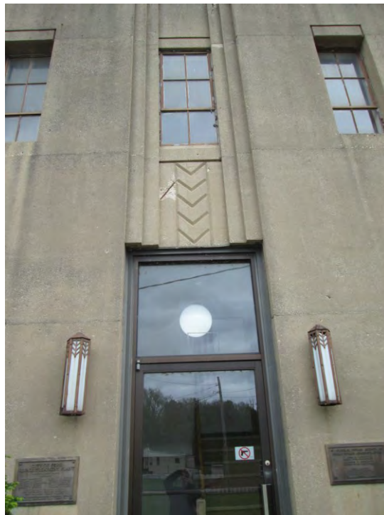
Photo 12: Detail of steel windows and incised detailing above entry on north elevation of Control Building.
