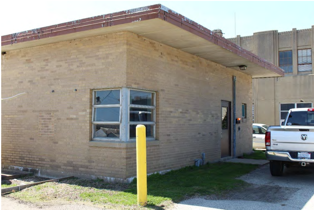
Photo 15: View southwest to east and north elevations of the Storm Building/Excess Flow.
