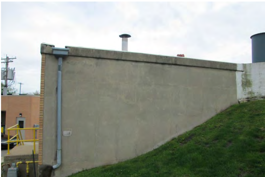
Photo 12: View south-southeast to northwest elevation of Boiler Room Building; Raw Sewage Screen Bar Building at rear left.
