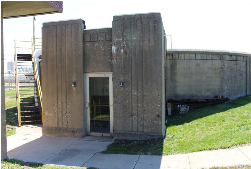
Photo 25: View south to building attached to north side of Secondary Digester Tank.
