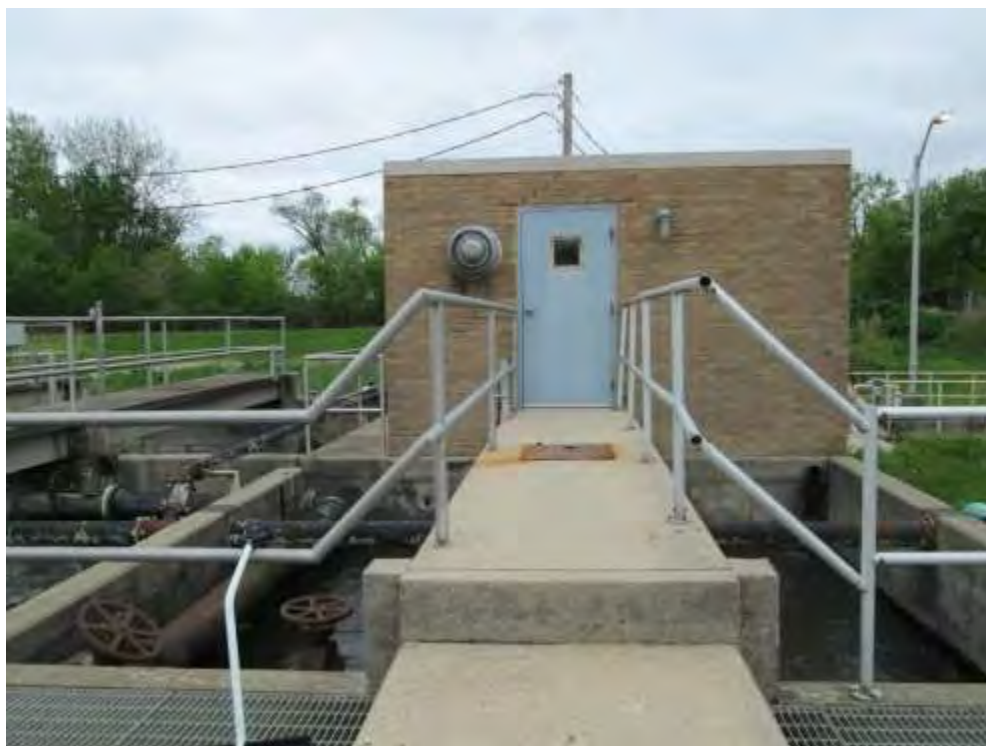
Photo 7: East elevation of Lab and Pump Building with secondary aerator/digester/clarifier in foreground.
