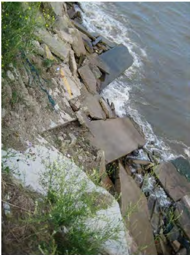
Bluff with unpermitted rubble fill (August 2009)
