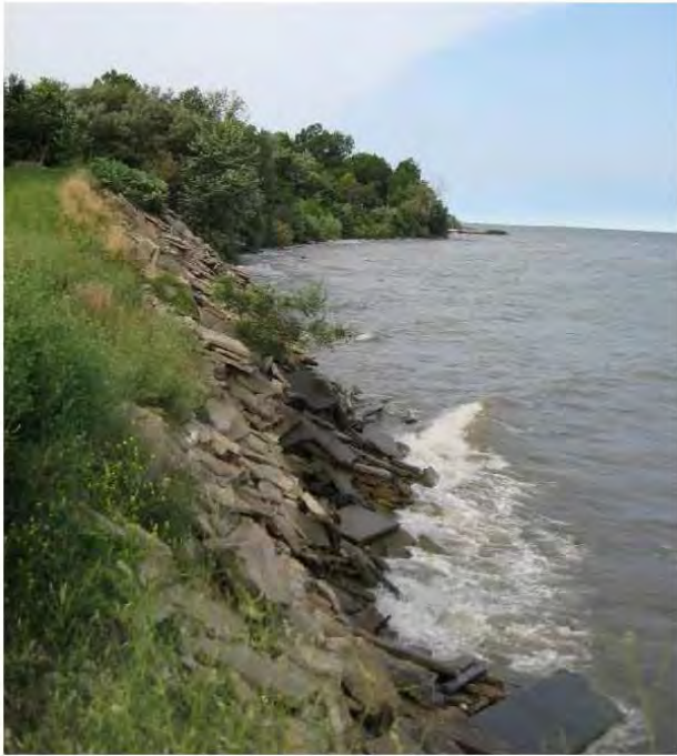
Bluff with unpermitted rubble fill (August 2009)
