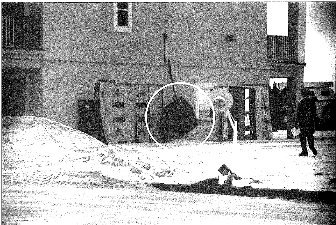
Figure 2-14 These breakaway panels functioned as designed. Note the loss of the air conditioning unit platform.
