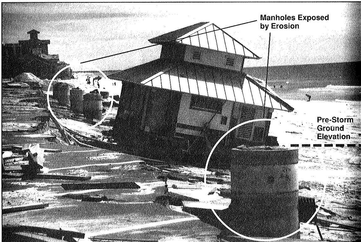
Figure 2-2 Beach erosion caused major damage to structures, as well as roads and utilities.
