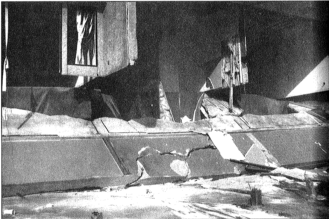
Figure 2-6 Undermining of concrete decks and floor slabs caused the failure of many unreinforced concrete structures.
