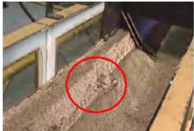
Figure 12. Bank erosion resulting from intermittent block failure
