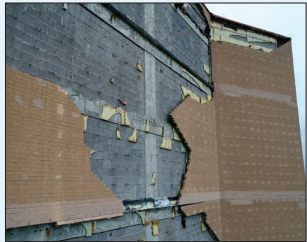
Photo 2: Drone image of brick veneer failure at a mid-rise building.
