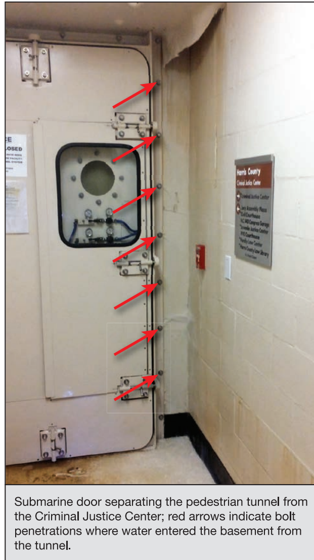
Figure 3-39: Floodwater seepage at submarine door
