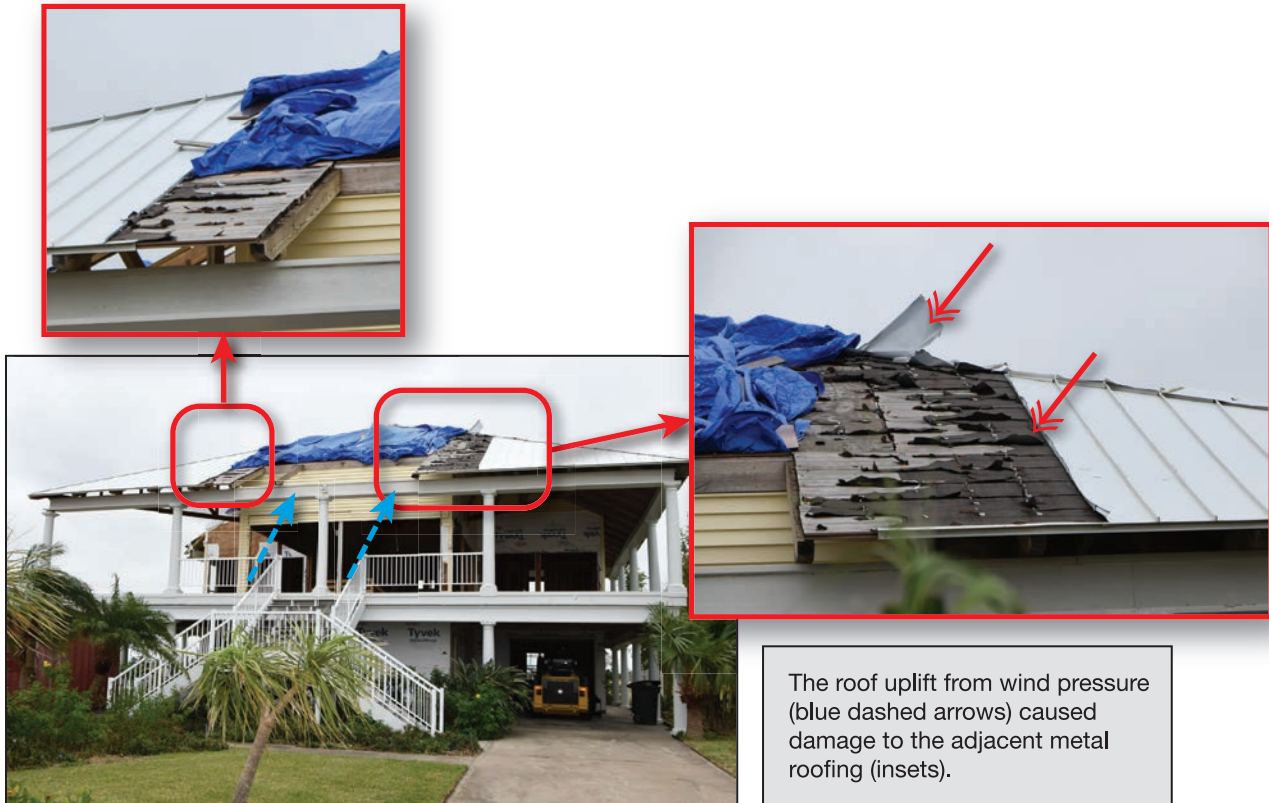
Figure 4-39: Home damaged by wind pressure (130 mph, Exposure C) (Cape Valero)
