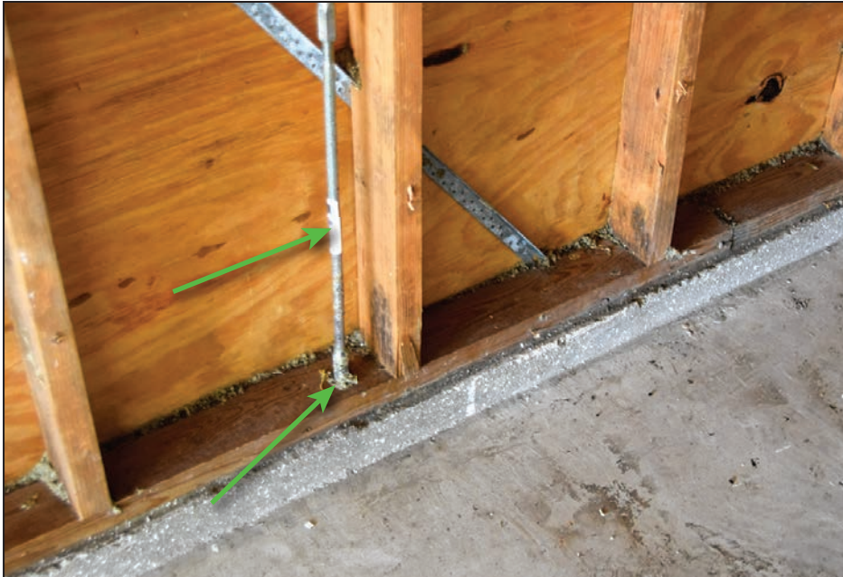
The bottom plate and coupling are shown with green arrows. Same building as Figure 4-1.
