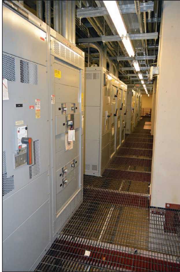
Figure 3-40: Floodwater did not reach critical equipment that was elevated after Tropical Storm Allison
