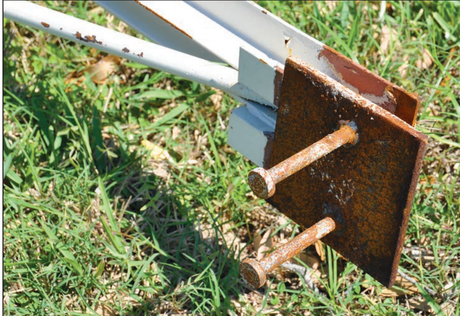
Figure 4-80: Bearing plate studs that were not grouted into the bearing wall and provided no uplift resistance. This condition was observed at many of the joists
