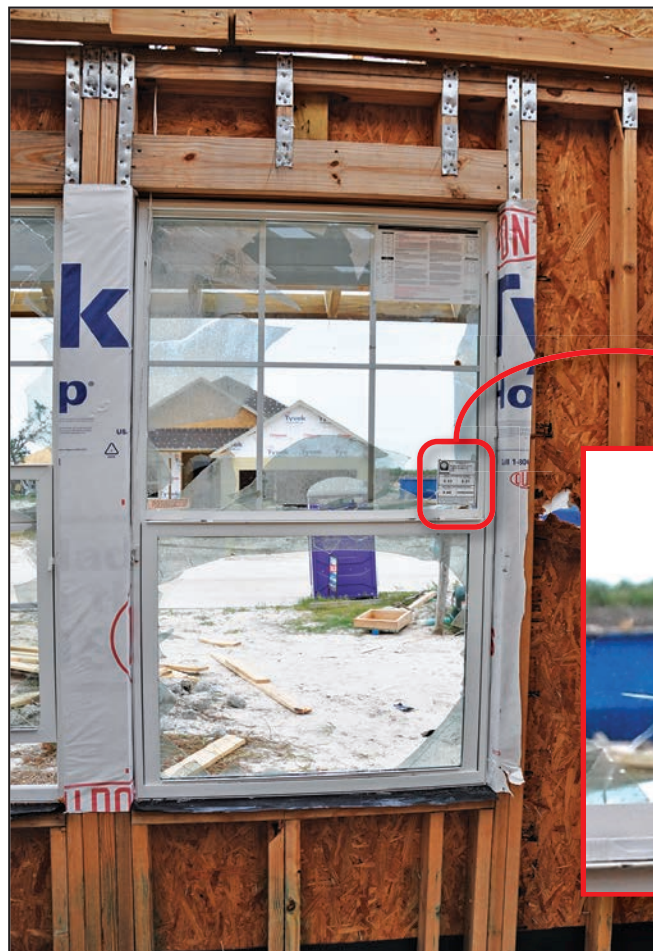
Figure 4-50: Newly installed impact-rated window in new construction to replace a window where all the panes were broken by debris impact (120 mph, Exposure B) (Estes)
