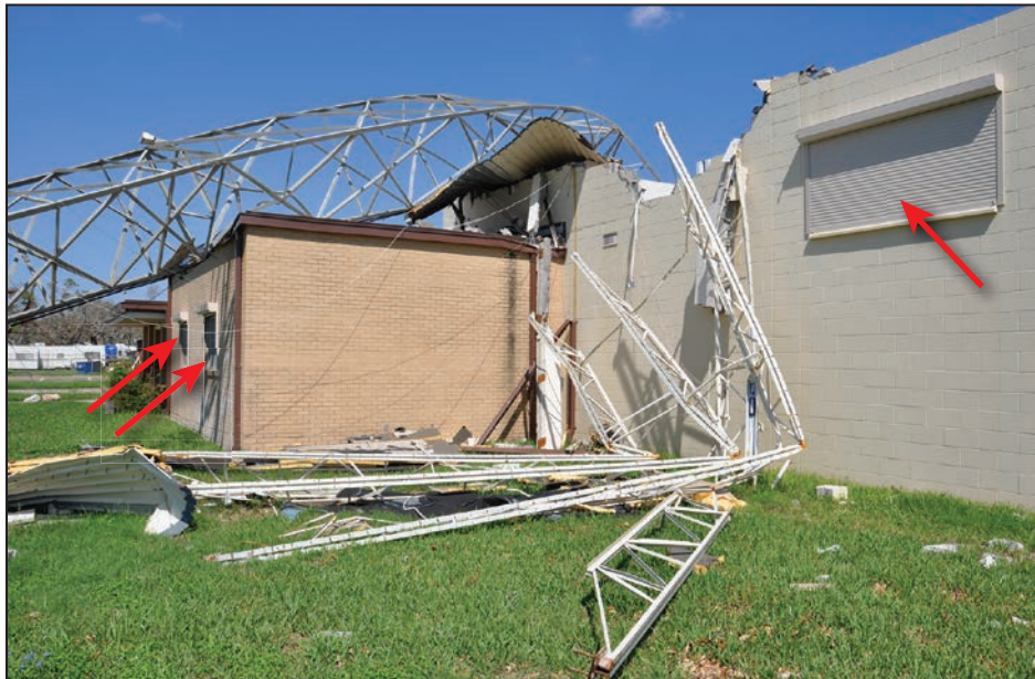
Figure 4-81: Although the exterior windows were protected with shutters (red arrows), the roof structure failure nullified their effectiveness
