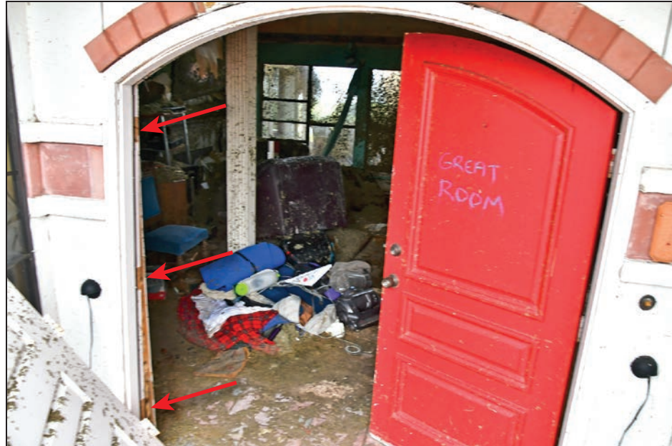
Figure 4-48: The inactive leaf of the door to this residence failed when wind and debris tore the door from its hinges (red arrows) (120 mph, Exposure C) (Rockport)
