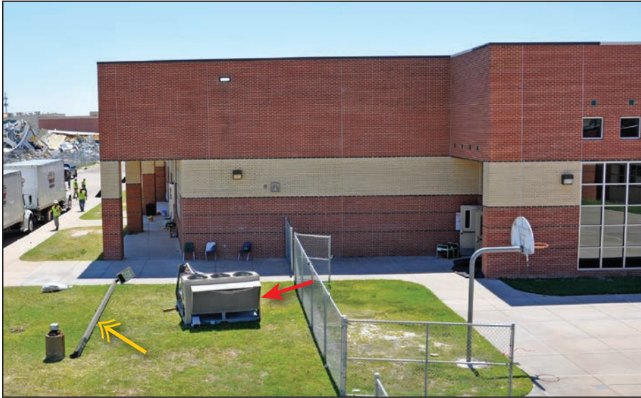
Figure 4-103: HVAC unit (red arrow) that blew off the roof and a collapsed light fixture next to the school (yellow double arrow; see Figure 4-104)
