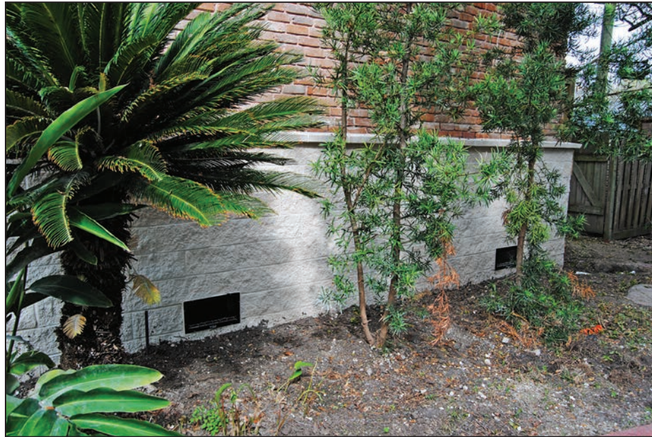
Figure 3-19: Exterior of new masonry perimeter foundation wall adjacent to piers supporting the elevated slab [Zone AE]
