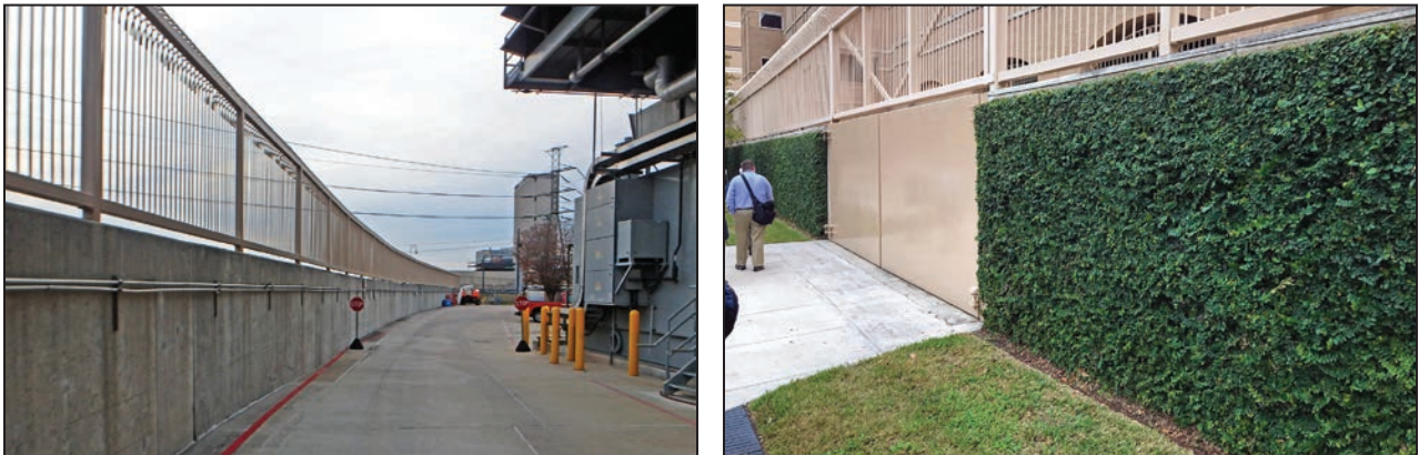
Figure 3-122: TECO floodwall adjacent to Brays Bayou (left image) and along Pressler Street (behind ivy in right image)
