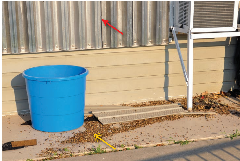
Figure 4-98: The red arrow indicates metal storm shutters. The yellow double arrow indicates aggregate blown from the roof shown in Figures 4-96 and 4-97
