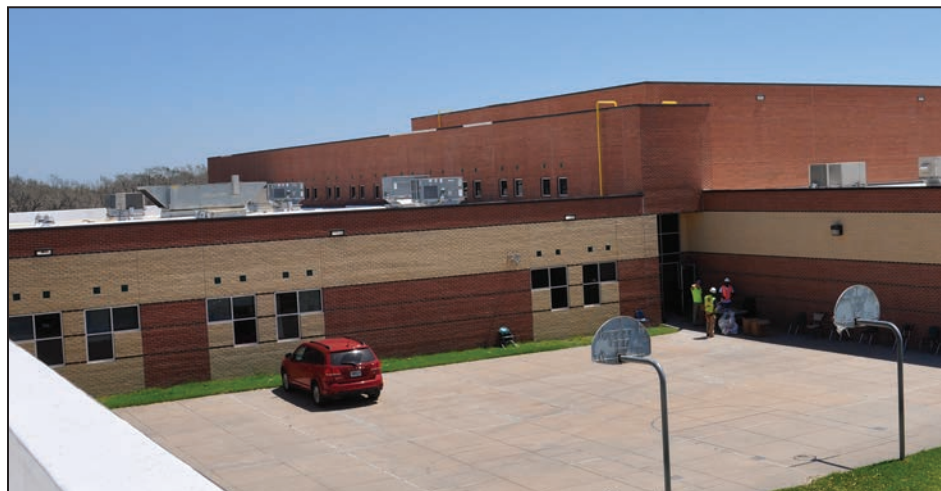
Figure 4-99: Rockport-Fulton Middle School. The HVAC units from the roof that were damaged had been moved to the ground after the storm and are shown in the foreground (Rockport)
