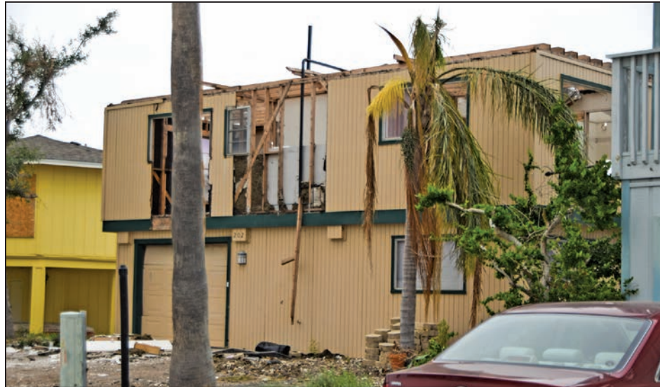
Figure 4-5: Older home with roof failure due to poor connection of the rafters to the joists (120 mph, Exposure B) (Rockport)
