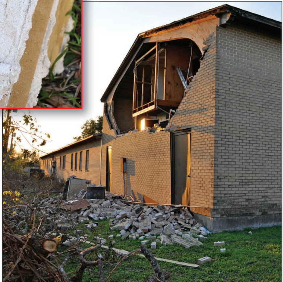
Figure 4-134: Brick veneer failure (Refugio)
