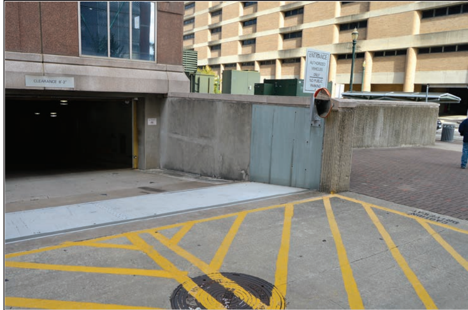
Figure 3-47: Automatic floodgate at ramp to basement parking garage
