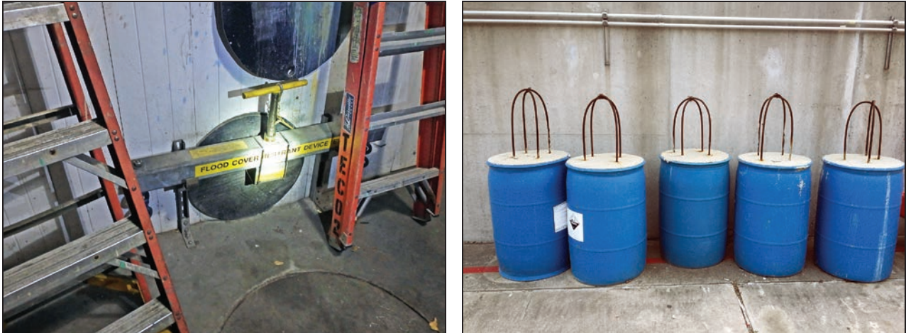
Figure 3-125: Vault flood cover restraining device (left) and barrels used as manhole cover restraining devices (right)
