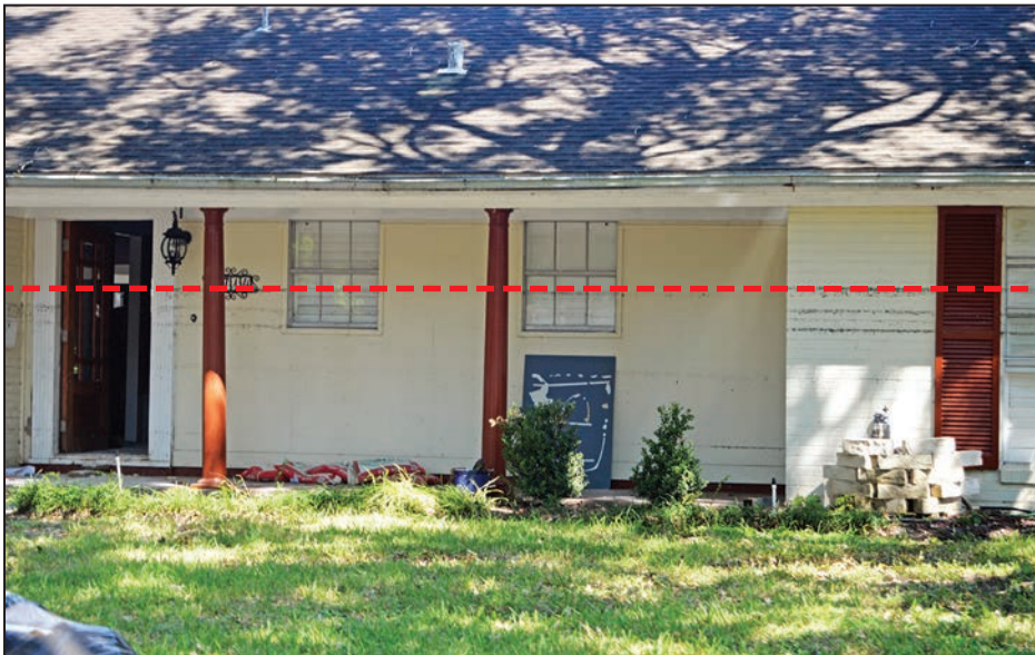
Figure 3-2: An approximately 5-foot-high HWM (shown as the dotted red line) observed by the MAT while assessing residential buildings on September 9 in Harris County [Zone AE]
