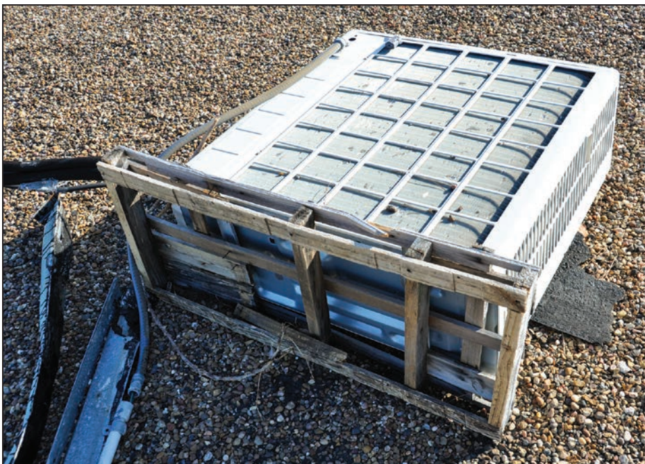
Figure 4-89: Inadequate attachment of rooftop condenser
