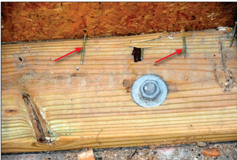
Same building as Figure 4-1.
