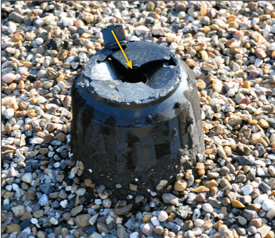
Figure 4-88: Unprotected vent opening
