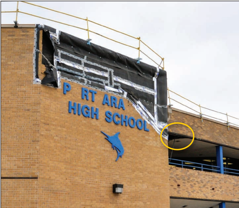
Figure 4-121: Signage, brick veneer, and soffit (yellow oval) failure
