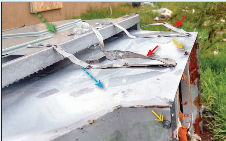
The green dotted arrow indicates the unit. The blue dashed arrow indicates the curb adaptor. The red arrows indicate straps that were supposed to attach the unit, curb adaptor, and curb. The yellow double arrows indicate screws between the adaptor and the curb (which was still on the roof).
