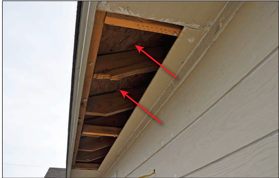
Figure 4-45: Ventilating fiber-cement board removed by the storm, exposing the attic (red arrows) (120 mph, Exposure B) (Holiday Beach)
