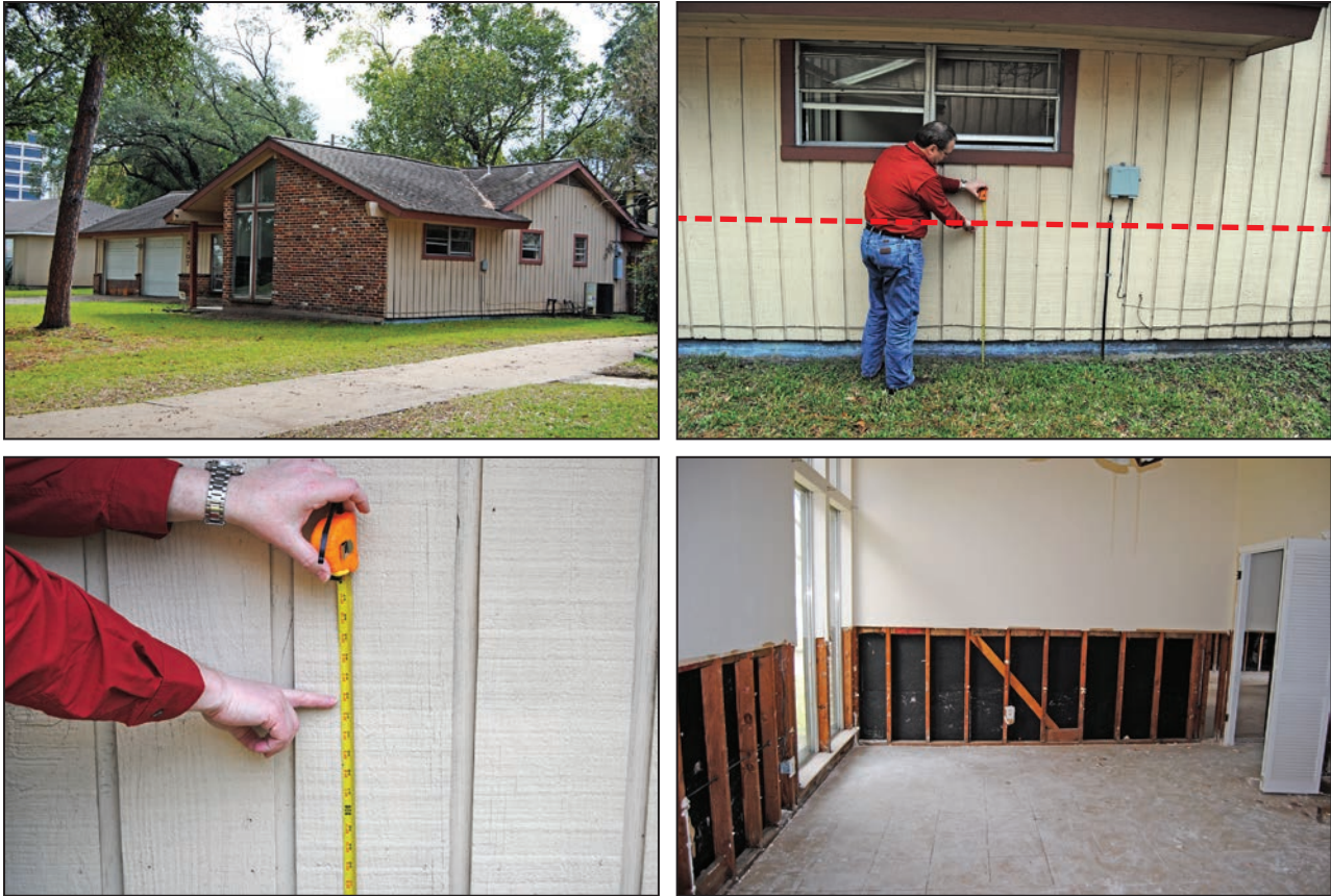
The interior damage shown in the image on bottom right is representative of typical damage observed by the MAT for single-family residences.
