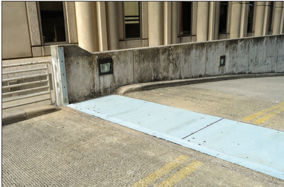
Figure 3-36: Flood shield that automatically deploys as waters rise at ramp to underground parking garage
