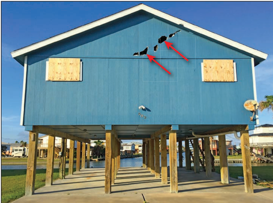
Figure 4-70: Multiple debris impacts on hardboard siding (red arrows) (120 mph, Exposure C) (Holiday Beach)
