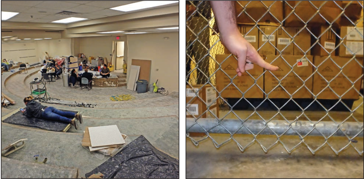
Figure 3-112: Basement auditorium used as water retention area (left) and reported water level in subbasement indicated by staff member (right)
