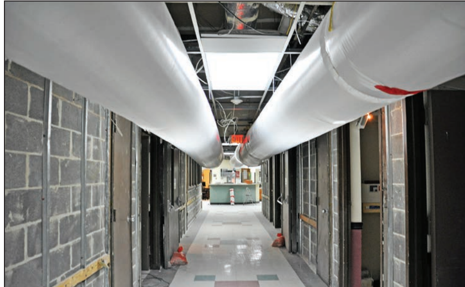
At the time of the MAT visit, the ceiling boards and gypsum wallboard had been removed, and temporary ventilation ducts had been installed.
