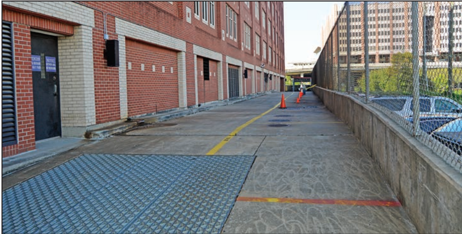
Figure 3-32: At-grade ventilation grill on north side of the building that was not inundated
