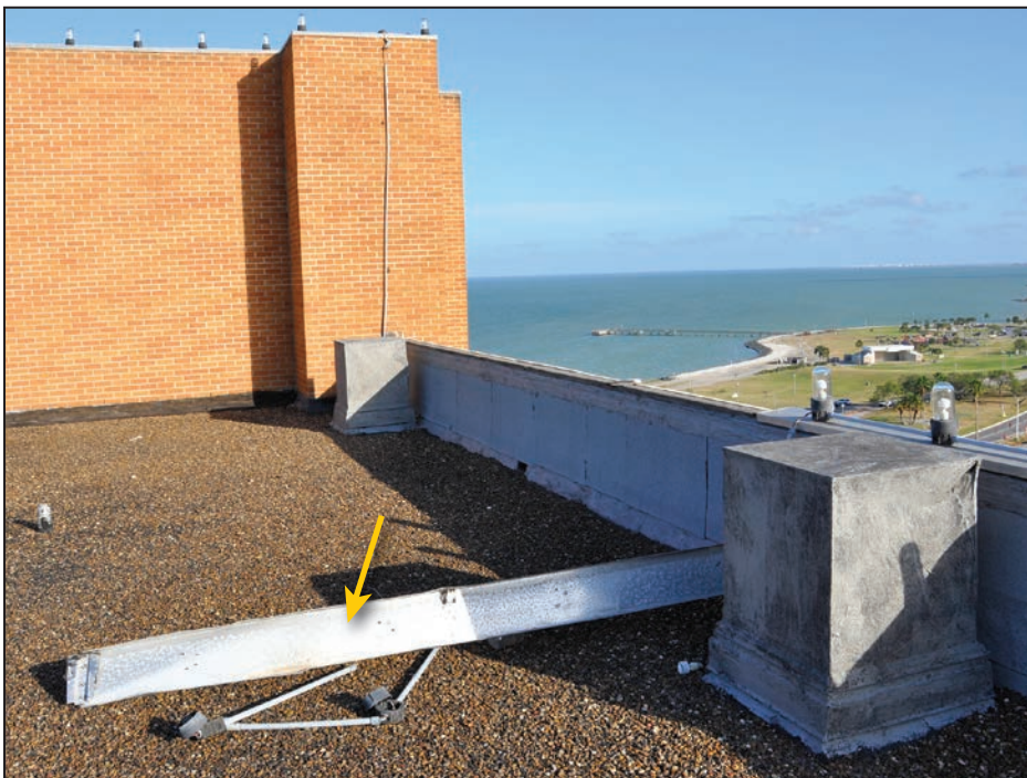
Figure 4-145: Sections of coping blew off at various locations along the parapet
