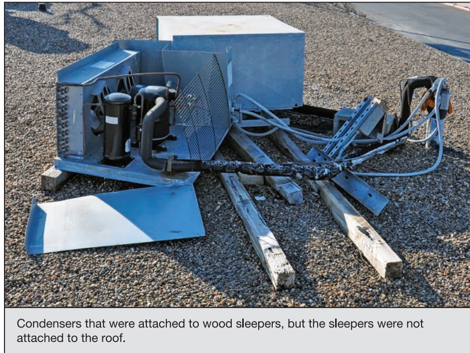
Figure 4-90: Inadequate attachment of rooftop condensers
