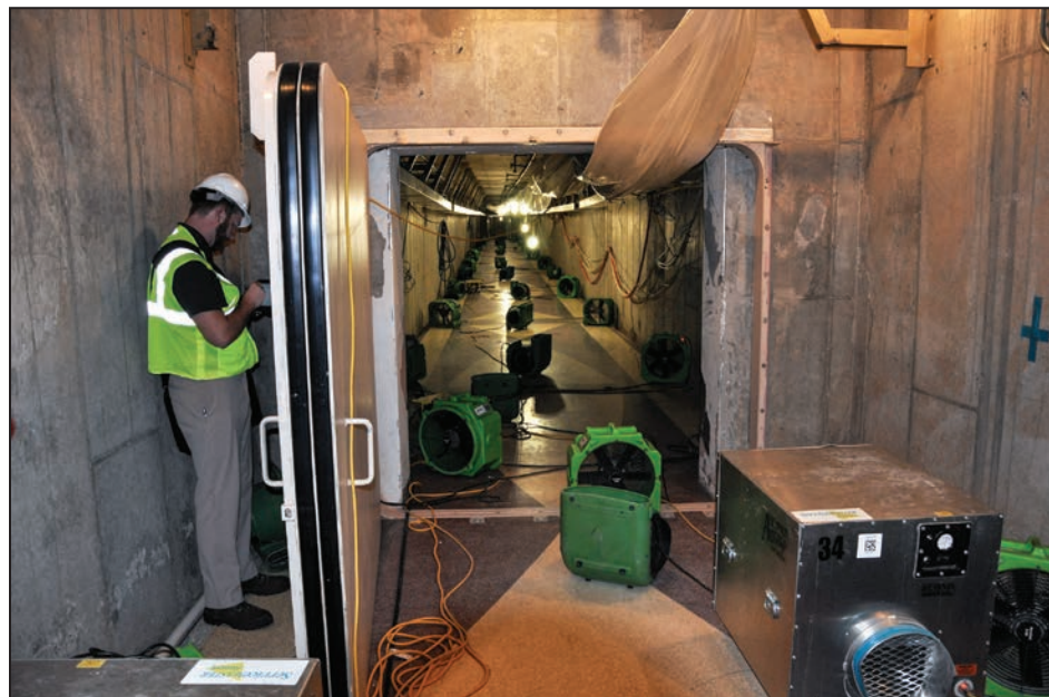
Figure 3-65: Submarine door that isolates the Wortham Theater from the Green Parking Garage
