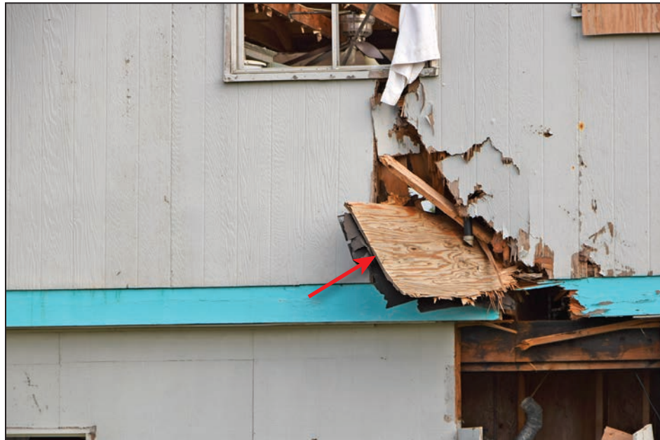
Figure 4-68: Plywood debris impact on hardboard siding (red arrow) (120 mph, Exposure C) (Port Aransas)
