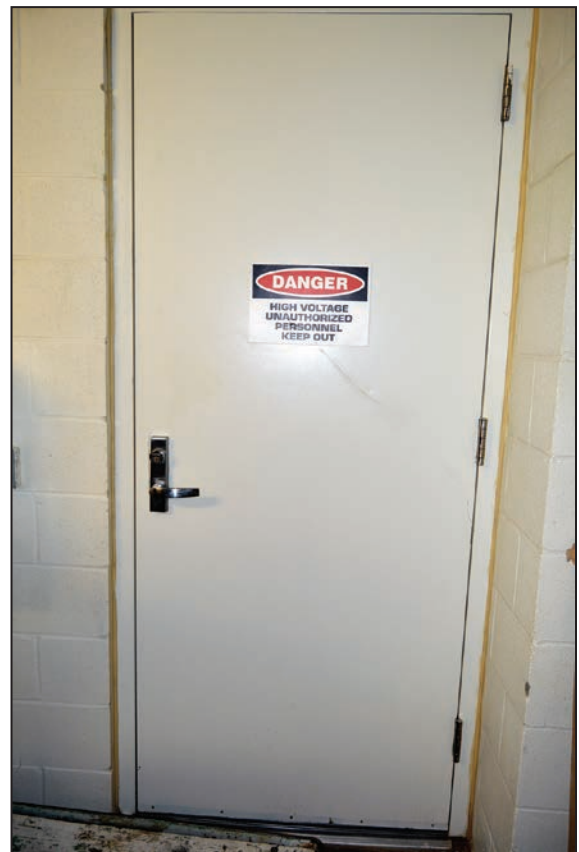
Figure 3-43: Door to the electrical utility vault, which is not designed to prevent floodwater entry
