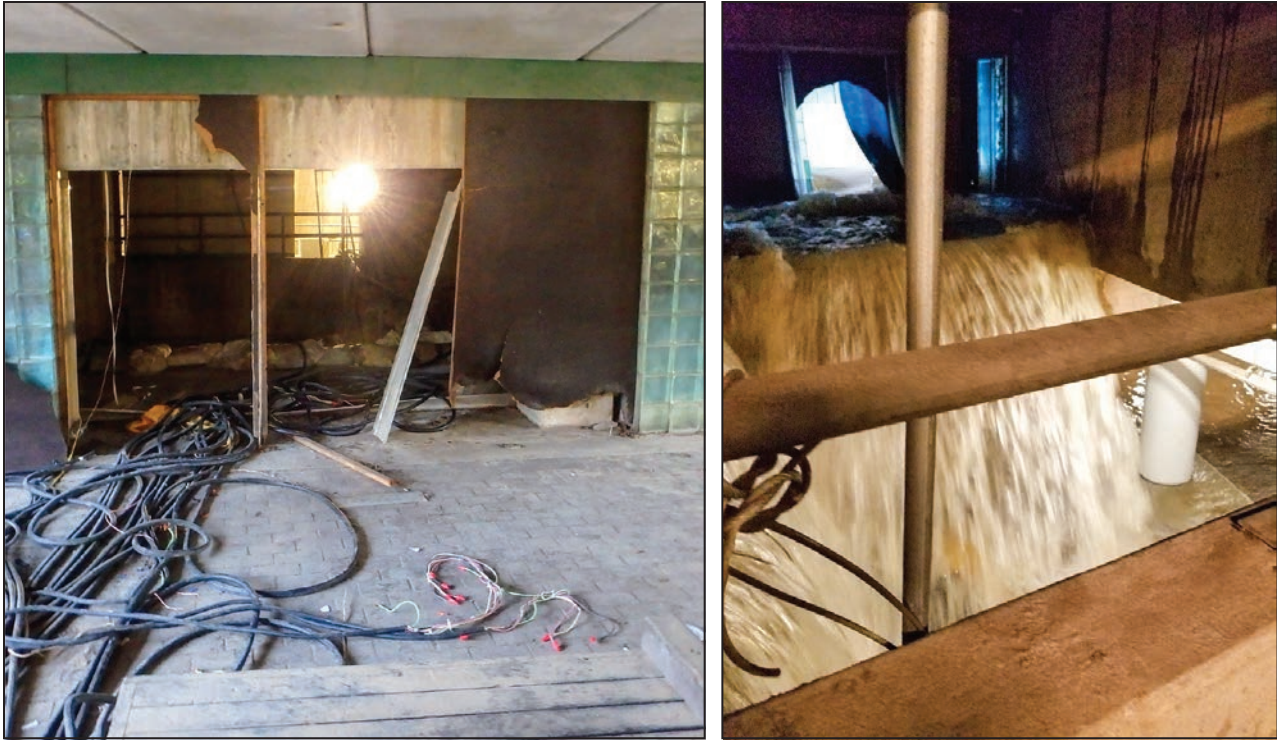
Figure 3-60: Glass block wall that failed when exposed to floodwater pressures (left); floodwater entering through Breach No. 3 (right)
