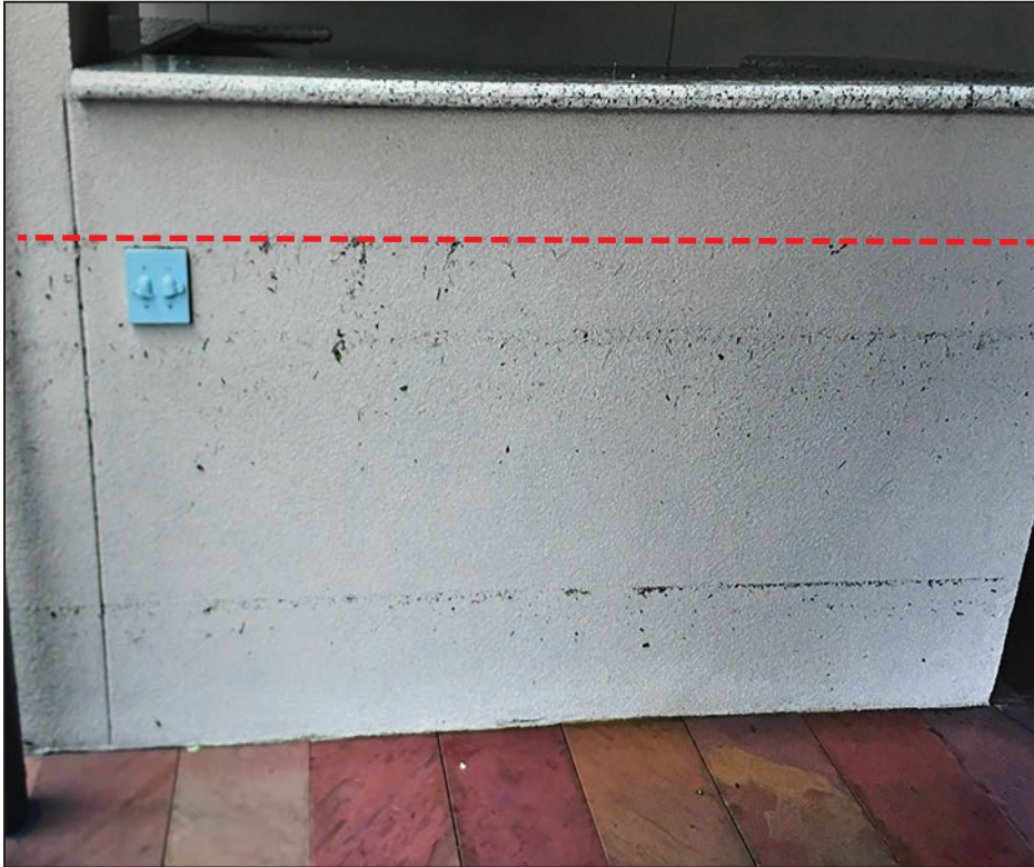
Figure 3-87: HWM near the swimming pool at the Four Leaf Towers condominium complex
