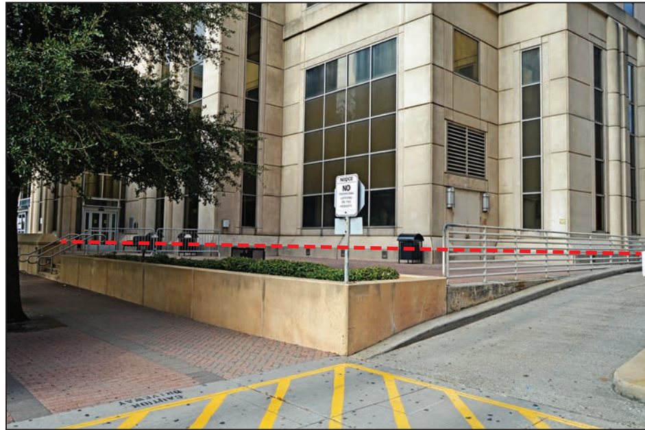
Figure 3-38: View of the Criminal Justice Center from the southeast with approximate depth of flooding indicated by dotted red line
