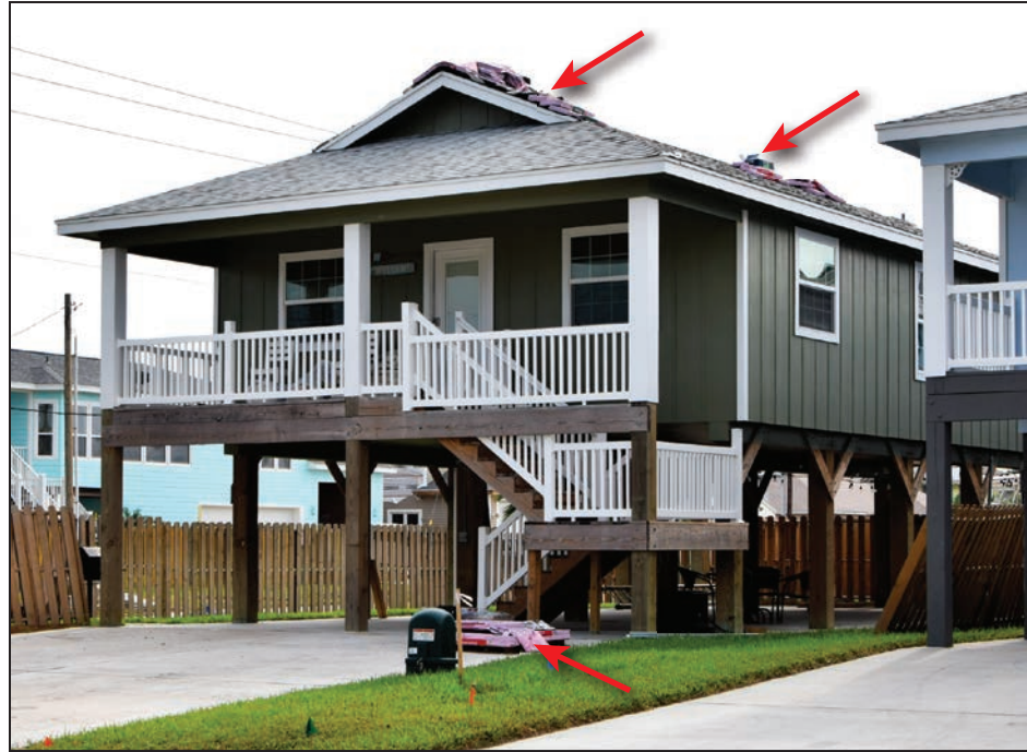
Figure 4-33: Home being reroofed with Class F shingles (see red arrows) (Port Aransas)
