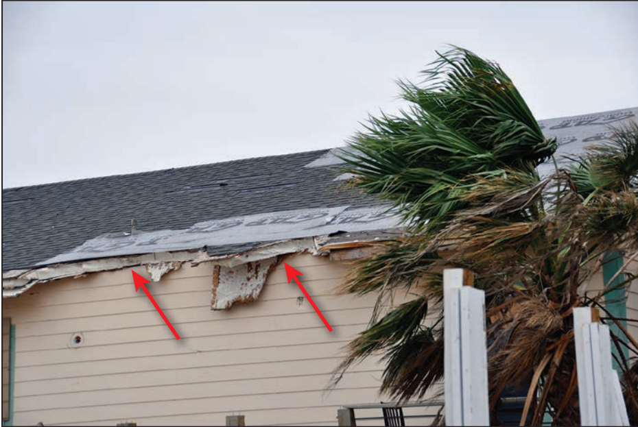
Figure 4-43: Roof overhang that snapped off (red arrows); image is a different view of home shown in Figure 4-42 (120 mph, Exposure C) (Copano Village)
