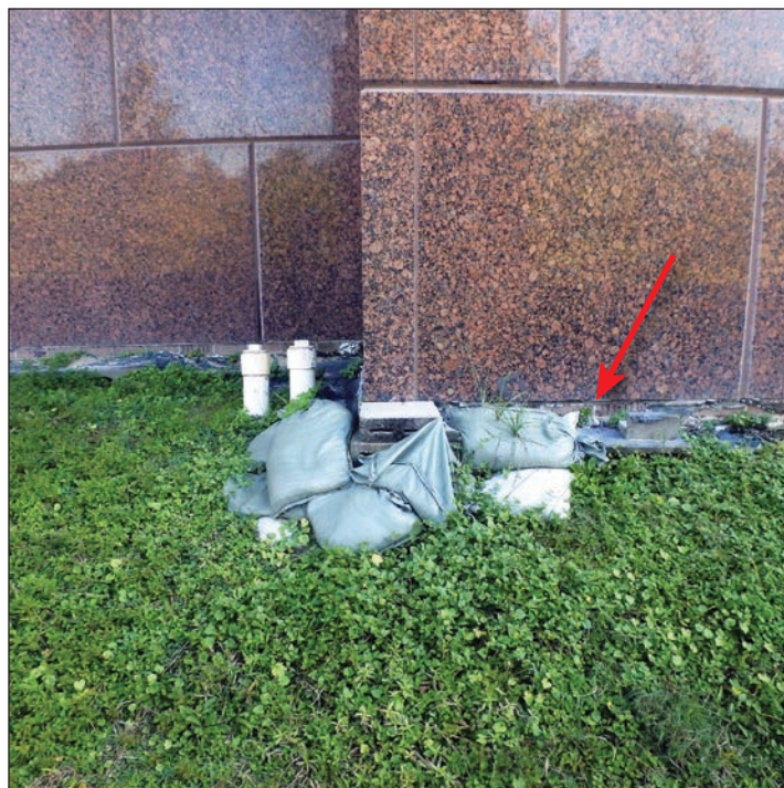
Figure 6: Unsealed joint (red arrow) between concrete foundation wall and a reinforced masonry wall with granite facing panel
