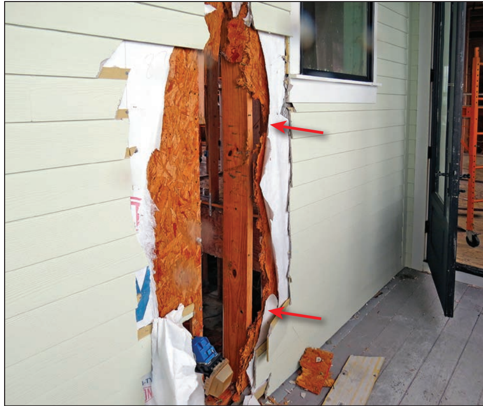
Figure 4-71: Large impact on fiber cement wall on the backside of the same residence as shown in Figure 4-66 (red arrows) (140 mph, Exposure C) (Key Allegro)
