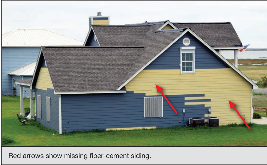
Figure 4-13: Fiber-cement siding damage to a residence (130 mph, Exposure C) (Copano Village)
