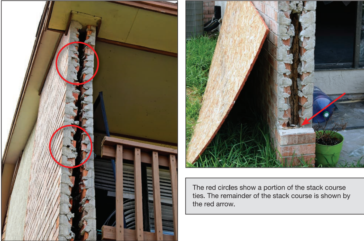
Figure 4-23: Double-wythe brick wing-wall that lost its brick stacked course (130 mph, Exposure B) (Port Aransas)
