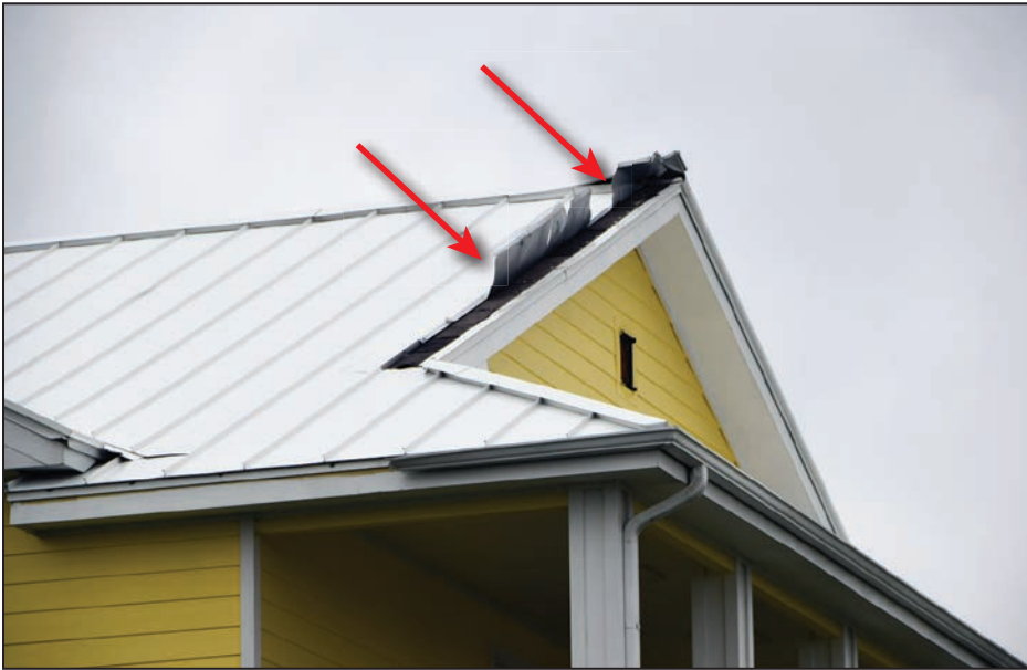
Figure 4-37: Residence with failed rake edge with loss of metal roofing edge trim (red arrows) (130 mph, Exposure B) (Copano Village)
