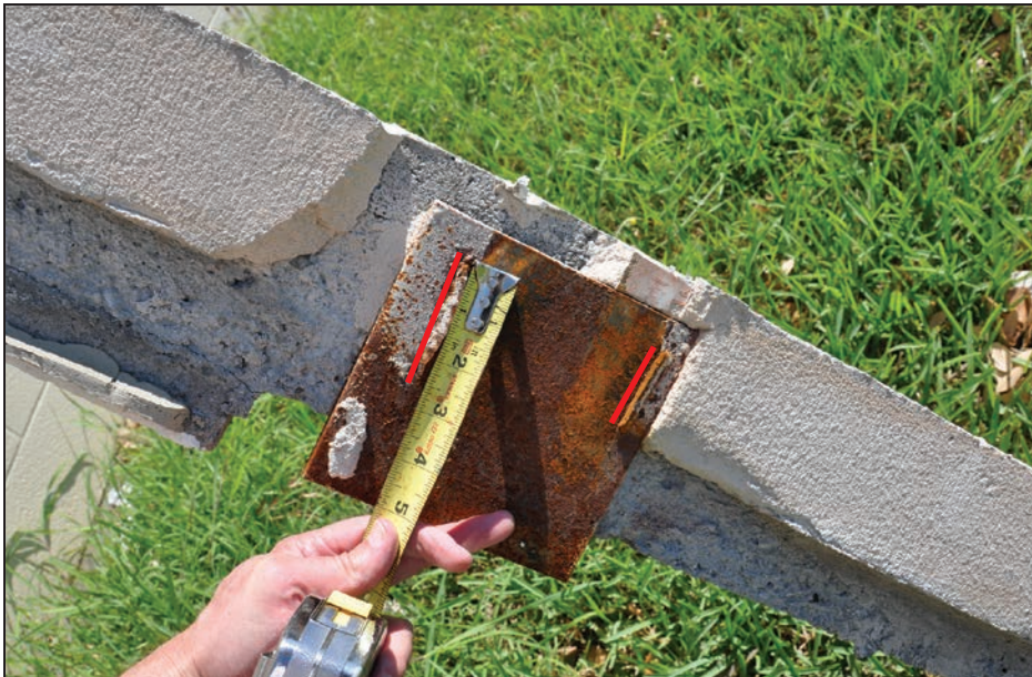
Figure 4-79: Joist bearing plate that is still attached to a bond beam that blew off
