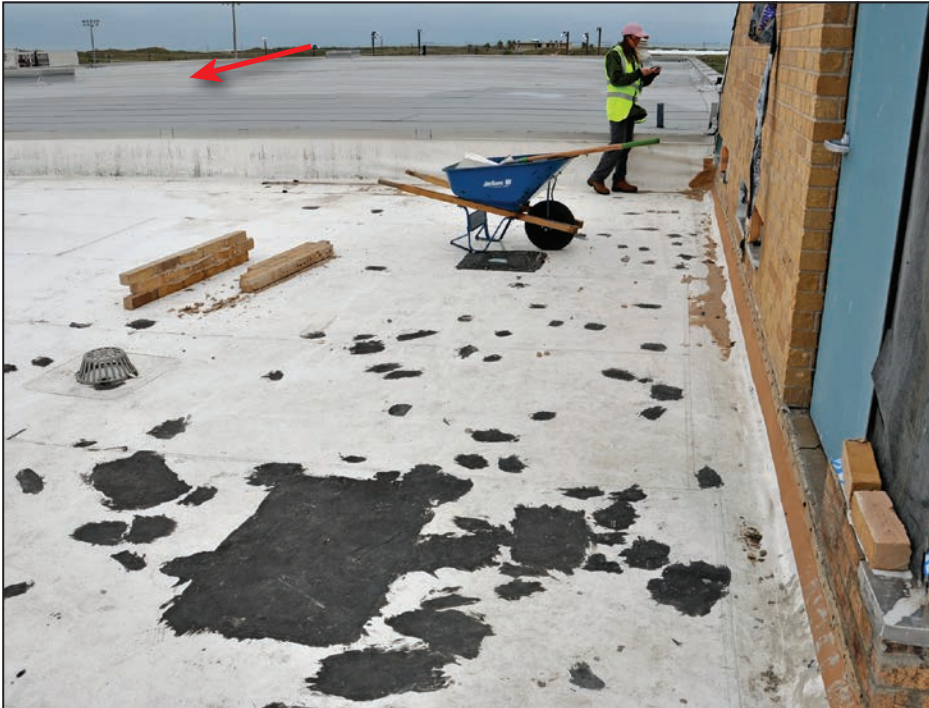
Figure 4-120: Brick veneer failure at a stair tower
