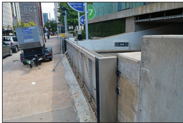
Floodgate protecting vehicle access to the underground Green Parking Garage.
