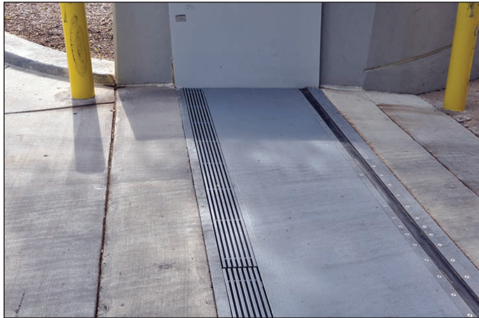
Figure 3-79: Passive floodgate located at the top of the loading dock ramp
