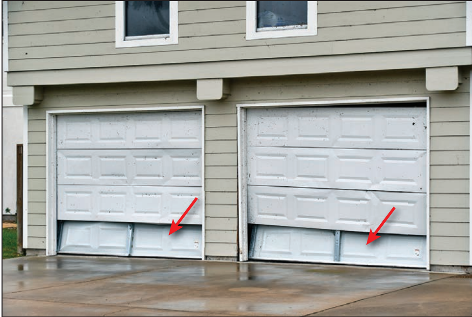
Figure 4-62: Home with insulated unreinforced garage door with loss of the lower exterior panel (red arrows) (Estes)
