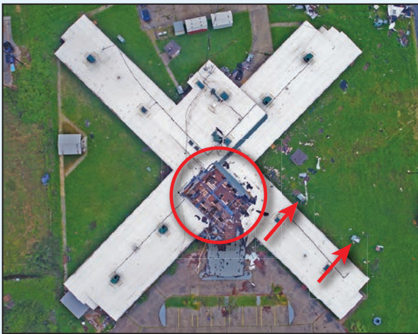
Photo 1: Drone image of a nursing home. The red arrows indicate rooftop heating, ventilation, and air conditioning (HVAC) units that blew off the roof. The roof deck blew off the area within the red circle. See Section 4.2 for further discussion of this facility.
