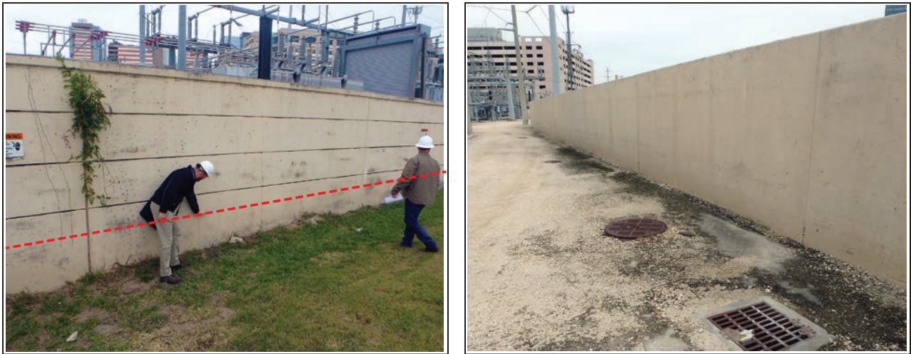
Figure 3-119: Exterior substation floodwall with water height shown (left) and interior wall surface (right)
