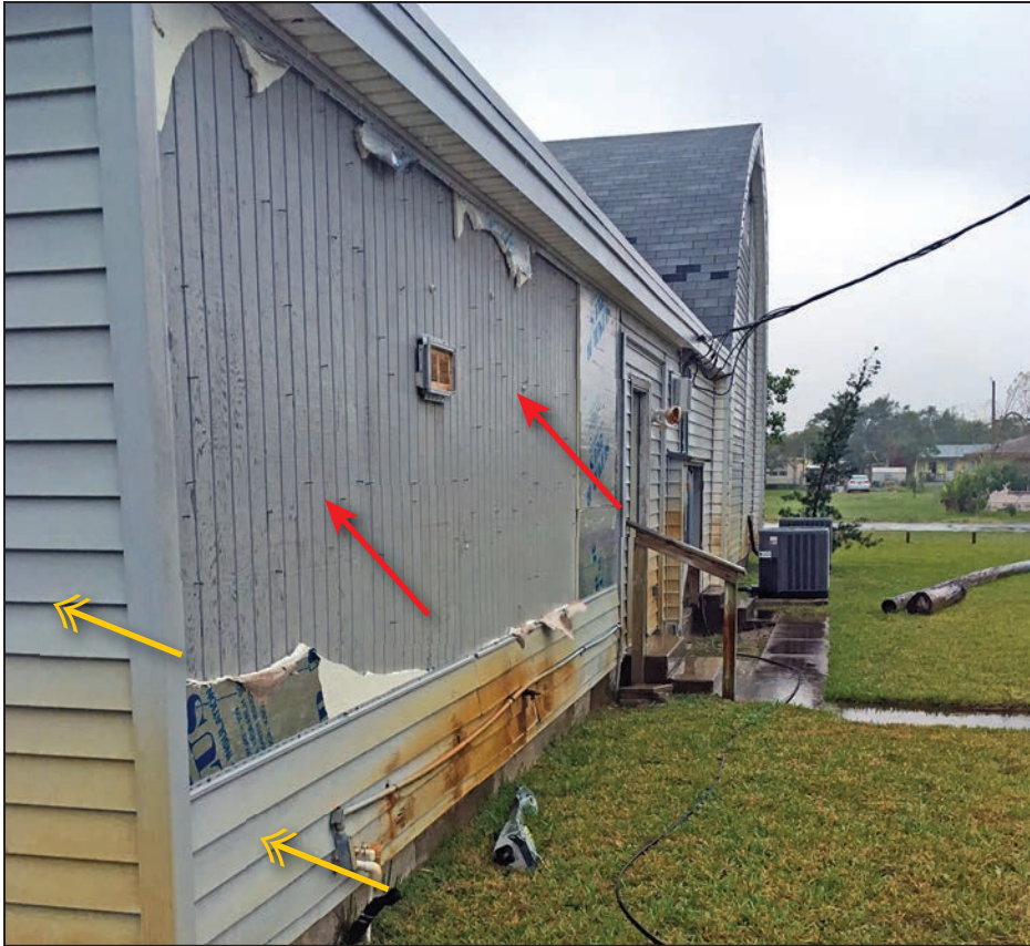
Figure 4-30: Older residence previously sided with hardboard vertical siding (red arrows) that had been re-sided with foam board and vinyl siding (yellow double arrows) (120 mph wind, Exposure B) (Rockport)
