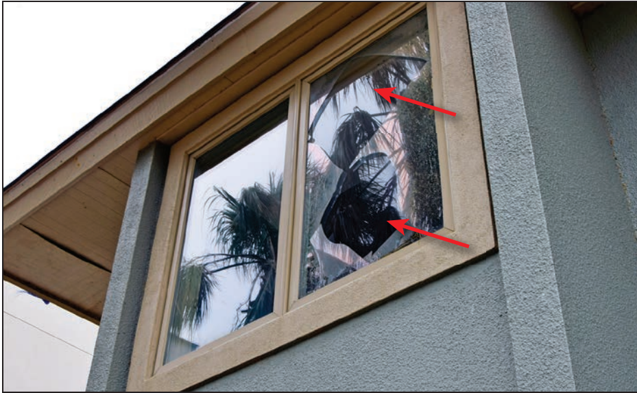
Figure 4-49: Outside layer of glazing sacrificed by the impact of wind-blown debris (Key Allegro)
