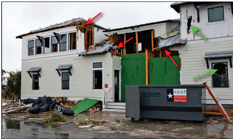
Figure 4-7: Intracoastal Waterway home that experienced a design-level wind event (130 mph, Exposure C) (Rockport)
