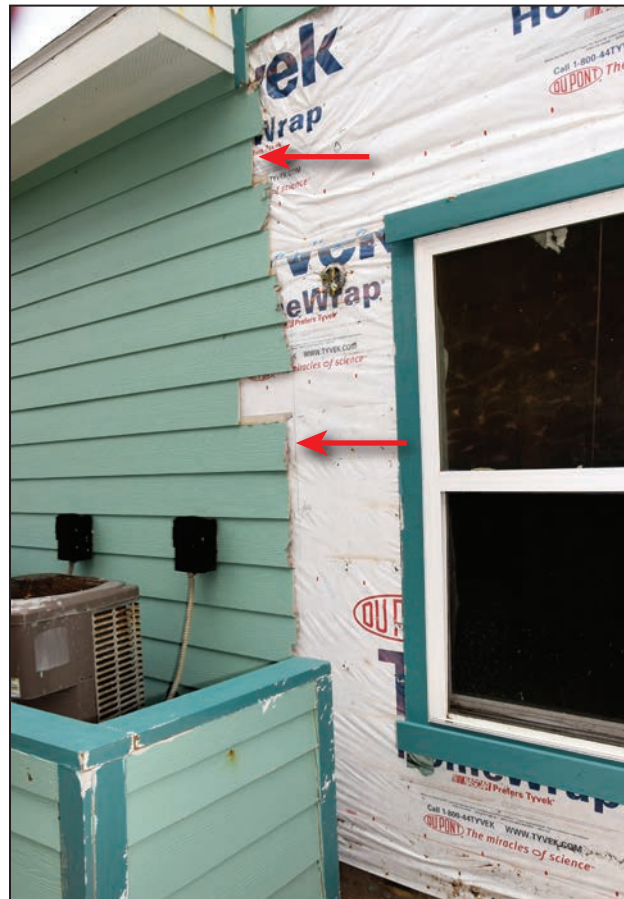
Figure 4-14: Fiber-cement siding ripped from walls (red arrows) (130 mph, Exposure C) (Port Aransas)
