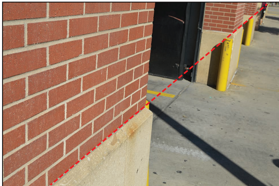
Figure 3-27: View of east wall of jail along N. San Jacinto Street where water levels reached the top of the concrete wainscot (red line)
