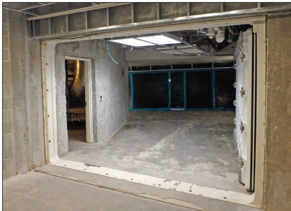
Figure 3-44: Submarine door separating the Jury Assembly Building from the underground pedestrian tunnel
