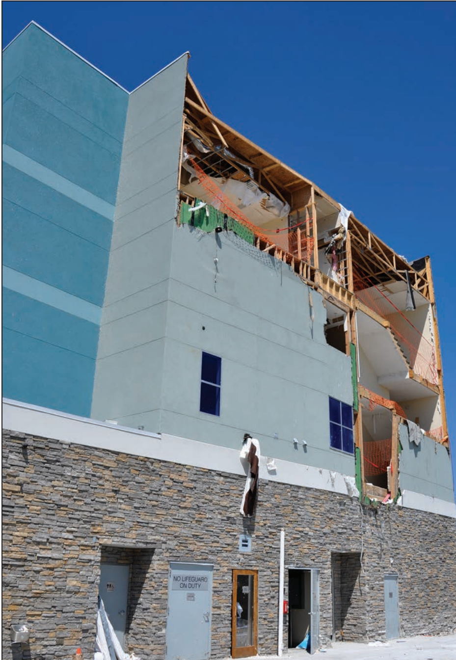
Figure 4-136: End wall failure at hotel (Rockport)
