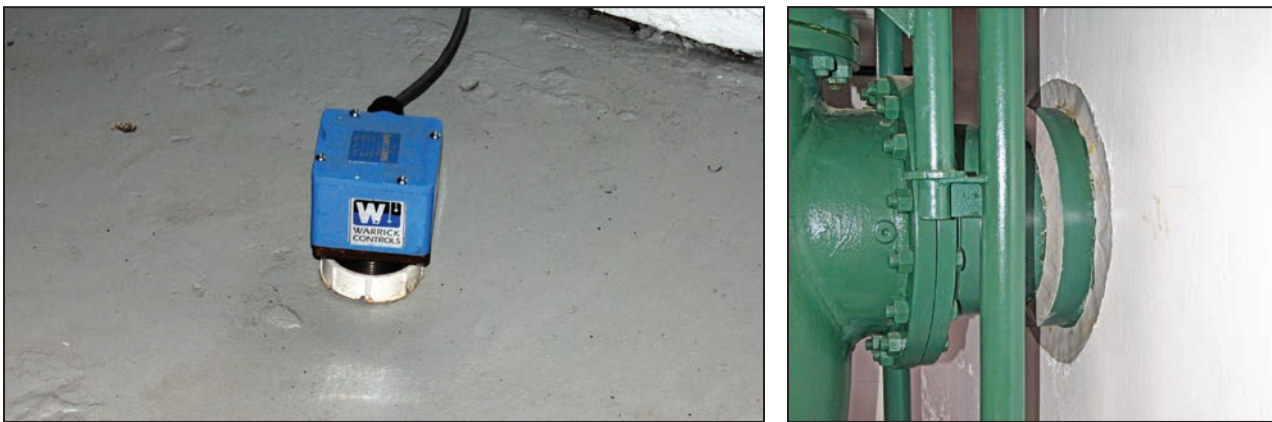
Figure 3-82: Wet alarm (left) and sealed pipe penetration (right)
