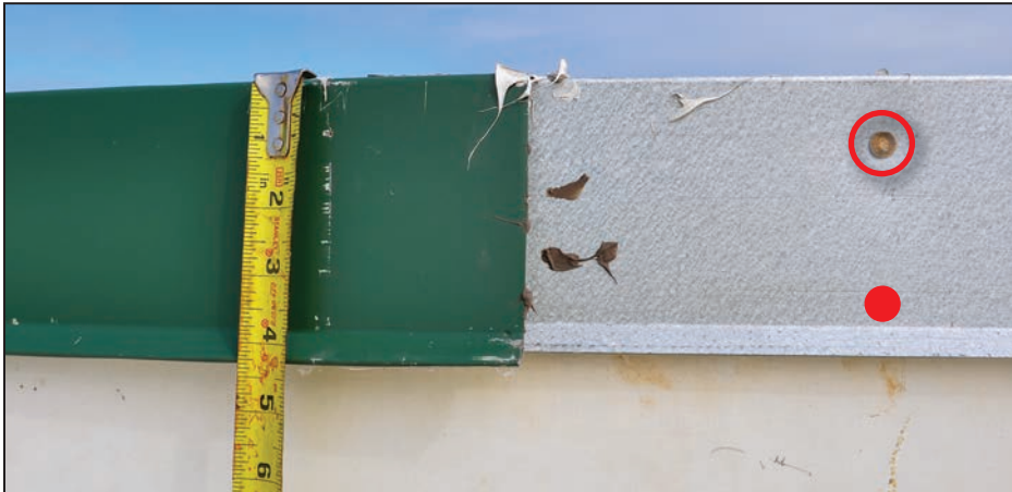
Figure 4-109: Cleat where a coping blew off
