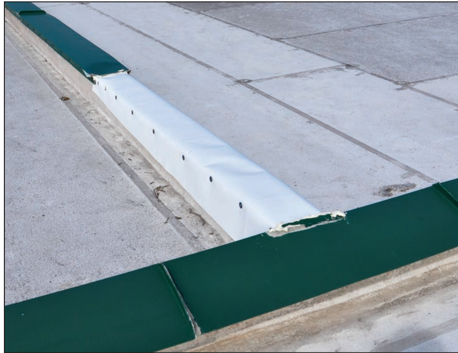
Figure 4-108: Blown-off coping at a curb. Depending on the curb design, interior water leakage may occur where copings are blown off
