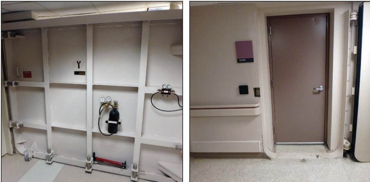
Figure 3-106: Flood doors in basement that subdivide basement areas within the Main Building
