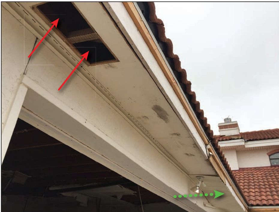
Figure 4-44: Vinyl soffit product (green dotted arrow) removed by the storm, exposing the vent opening (red arrows) (120 mph, Exposure B) (Cape Valero)
