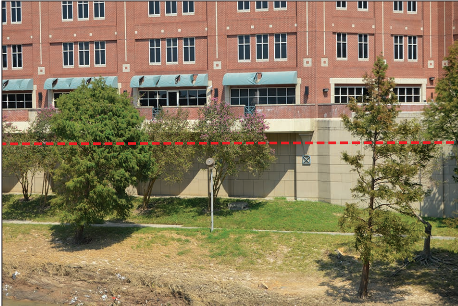
The approximate HWM (red line) was reported by jail staff. Staff reported that water flowed down the interior surface of this wall.
