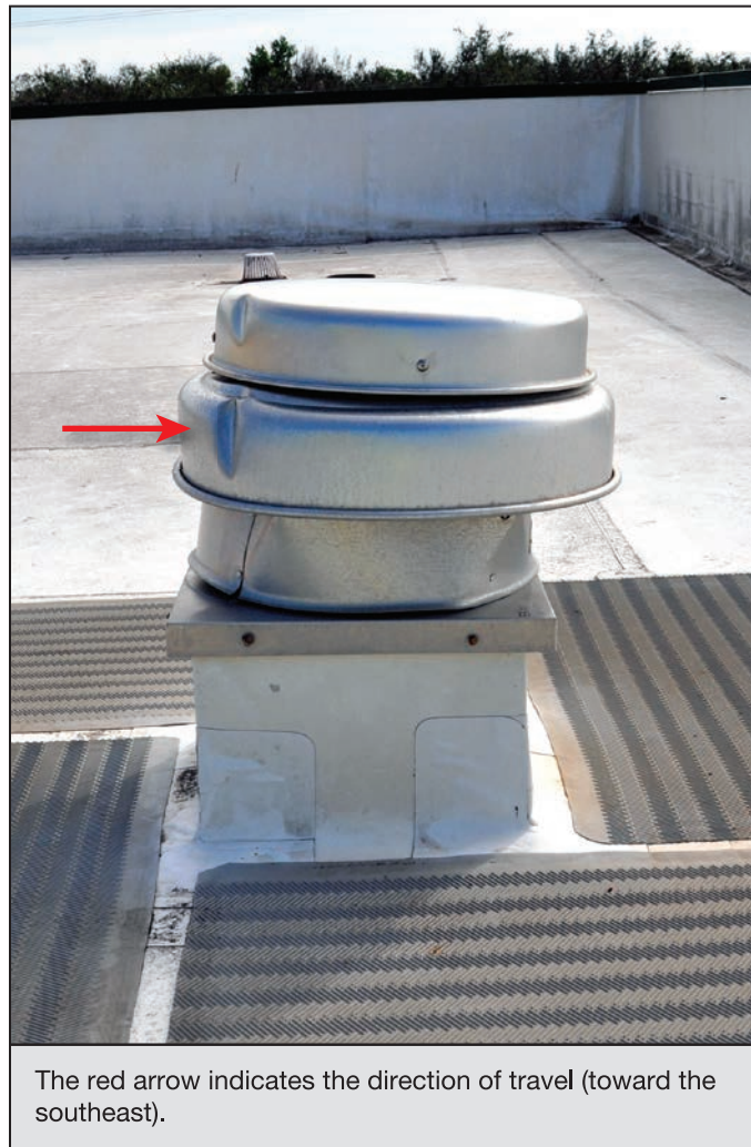
Figure 4-111: Exhaust fan struck by wind-borne debris
