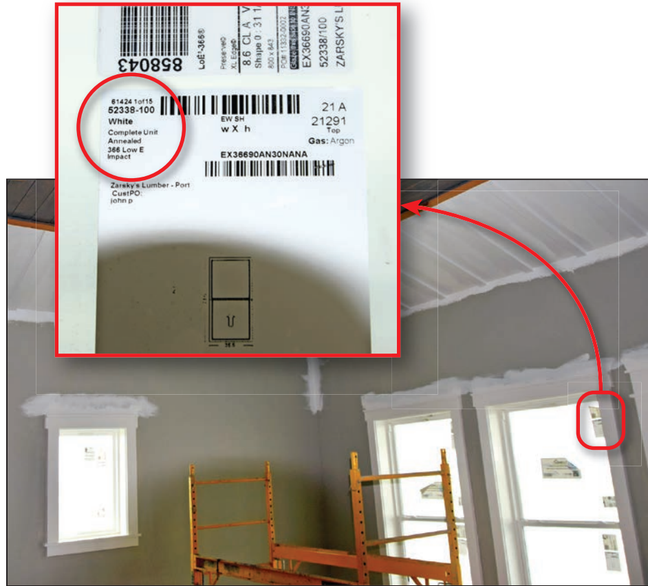
Figure 4-51: Impact-resistant glazing in new construction (red circle) (Cape Valero)
