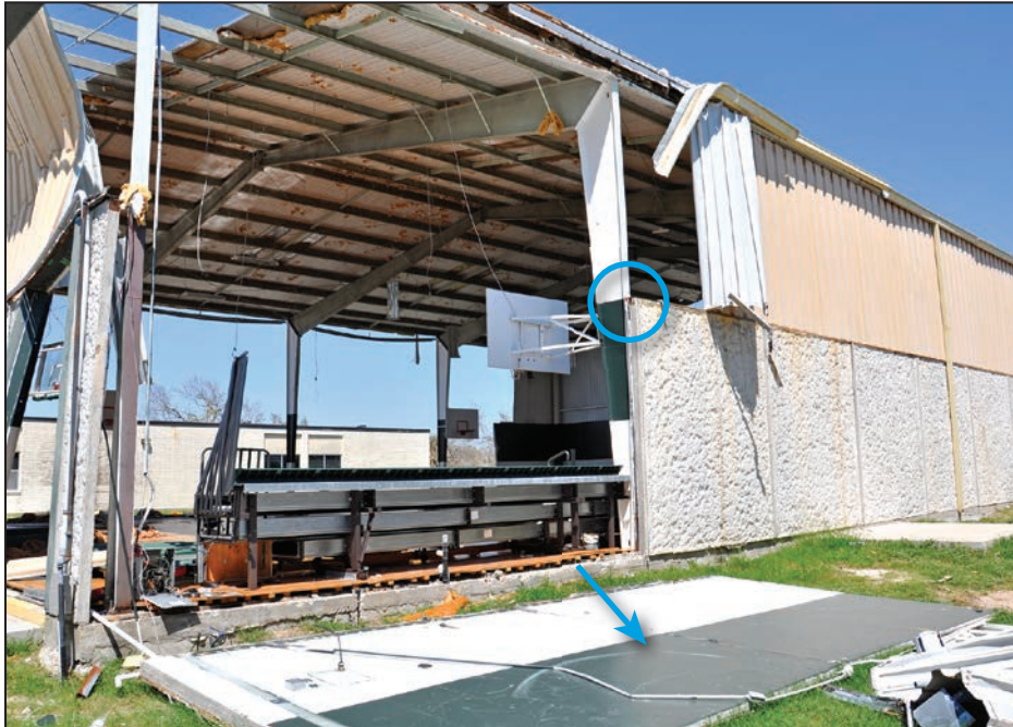
Figure 4-139: High school gymnasium damage (Rockport)
