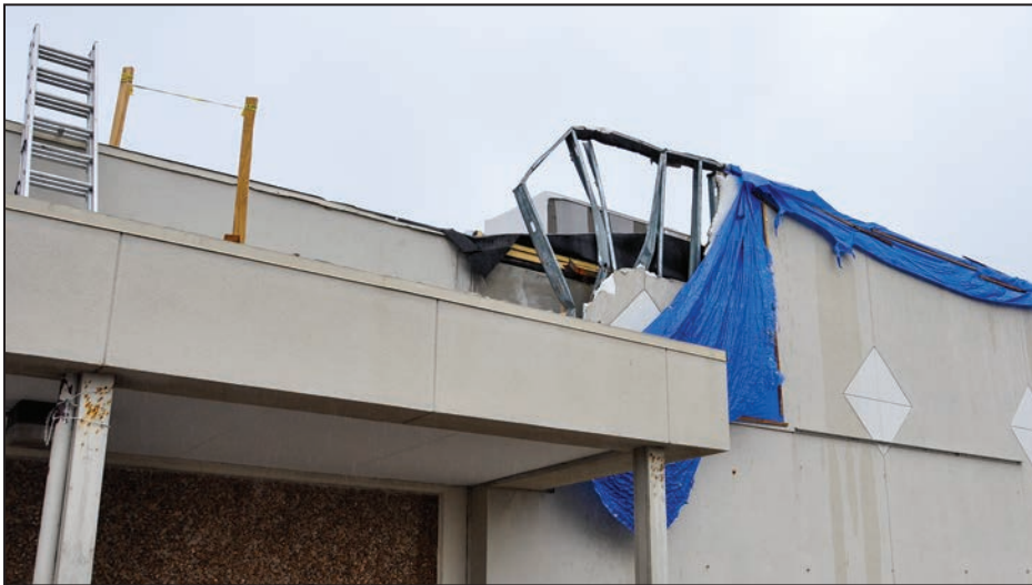
Figure 4-129: Damaged parapet; Exterior Insulation and Finish System (EIFS) over metal framing
