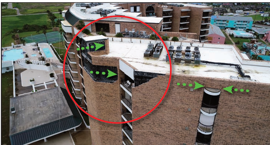
Brick wall damage is shown in the red circle and thermal expansion control is shown with the green arrows.
