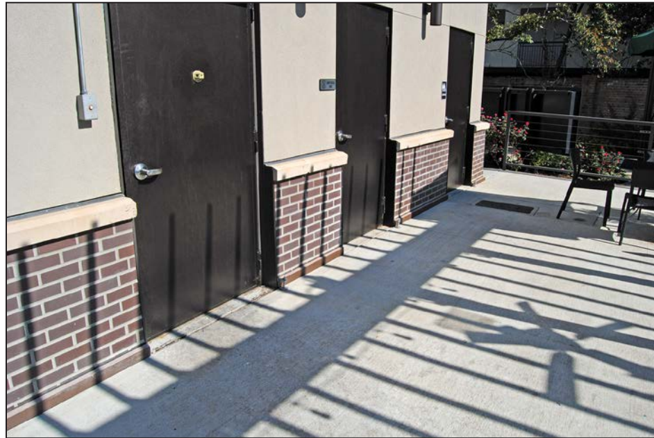
Figure 3-91: Pedestrian flood doors installed to access restrooms, storage room, and employee entrance
