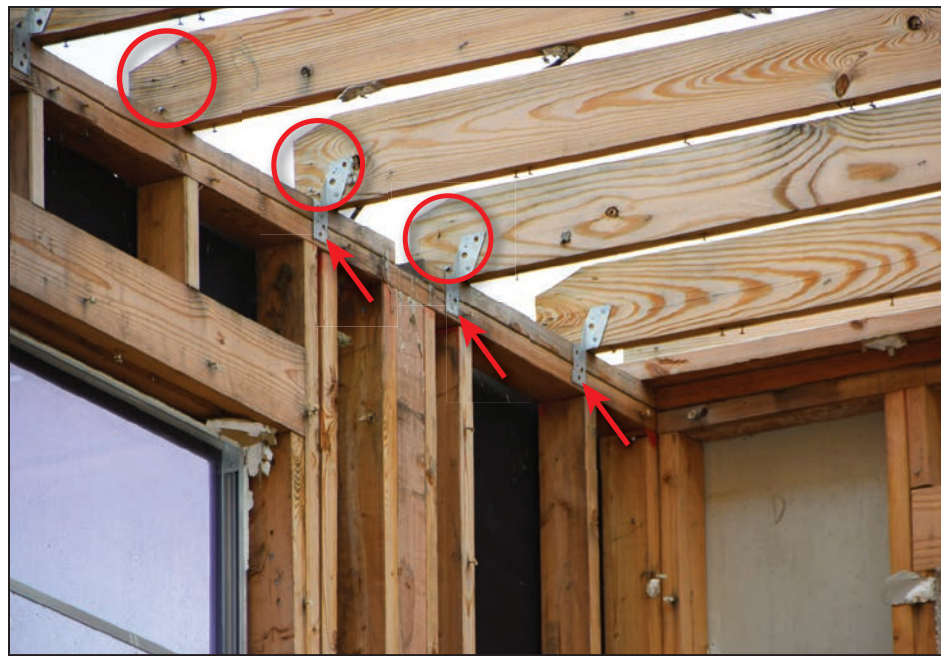
Ceiling joists clipped to top wall plate (red arrows). Missing roof rafters appeared to be either toe-nailed or nailed to the ends of the ceiling joists (red circles).
