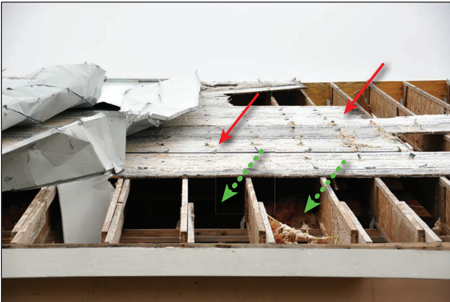
Figure 4-38: Residence with failed substrate (green dotted arrows) and no membrane underlayment (red arrows) (Copano Village)
