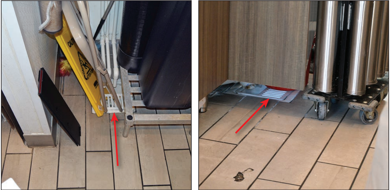
Figure 3-93: Floor drains (red arrows) where floodwater entered
