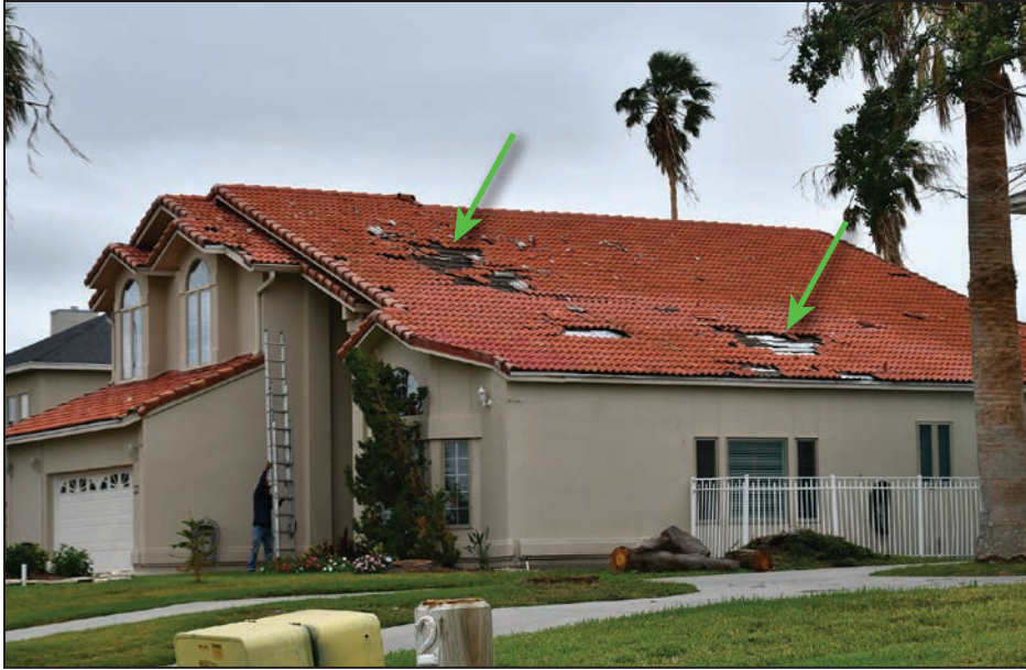
Figure 4-40: Home with clay tile roof failure (green arrows) (120 mph, Exposure C) (Key Allegro)
