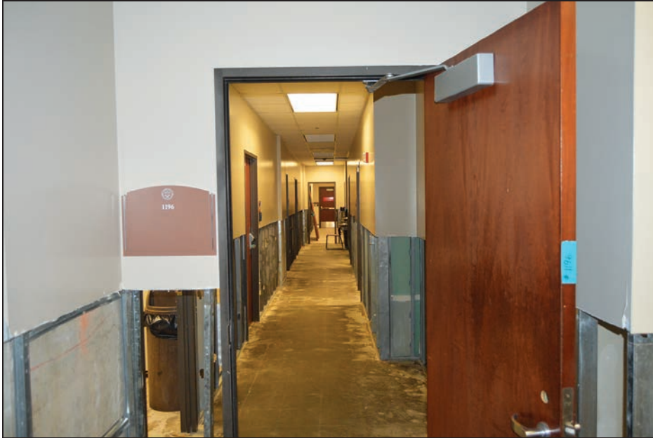
Figure 3-41: Wall finishes were removed from the first floor as a result of sewage leakage
