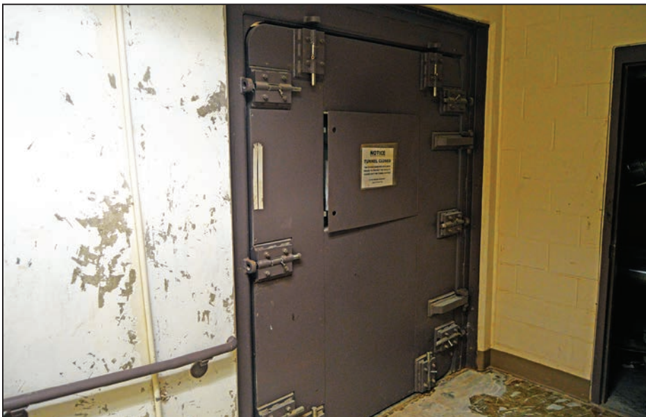
Figure 3-46: Submarine door that separates the Civil Courthouse basement from the underground pedestrian tunnel
