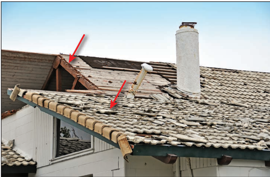
Figure 4-41: Home with concrete tile roof failure (red arrows) (120 mph, Exposure B) (Copano Village)
