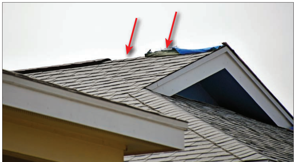
Figure 4-46: Home with a portion of ridge vent removed by Hurricane Harvey winds (red arrows) (120 mph, Exposure B) (Rockport)
