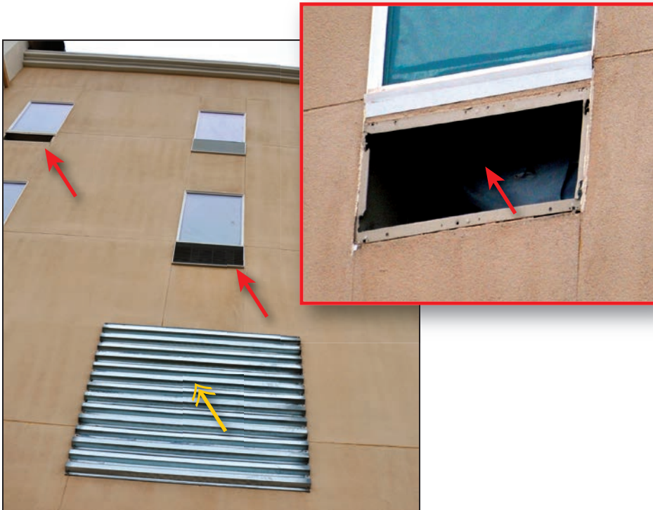
Figure 4-124: The red arrows indicate where PTAC wall louvers were blown away. The lower level windows were protected with metal shutters (yellow double arrow)
