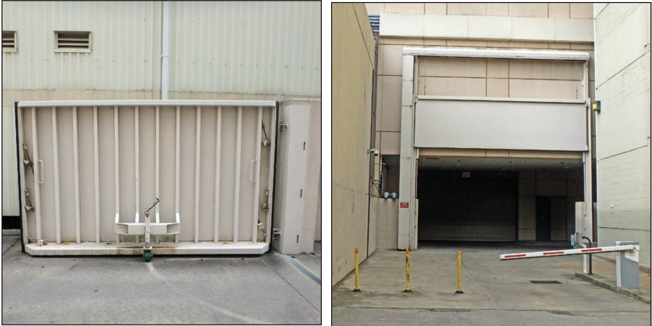
Figure 3-114: Swing flood door (left) and guillotine floodgate (right)
