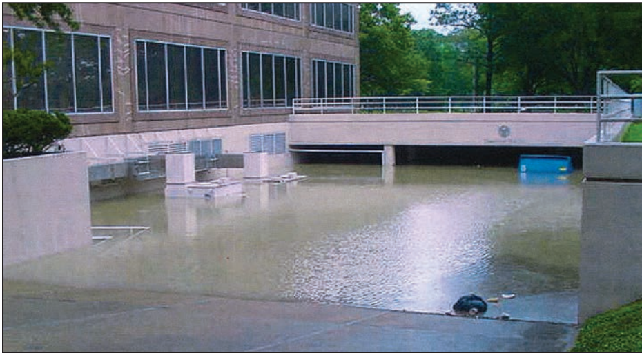
Figure 3-74: Flooding of the loading dock during a severe thunderstorm in 2009
