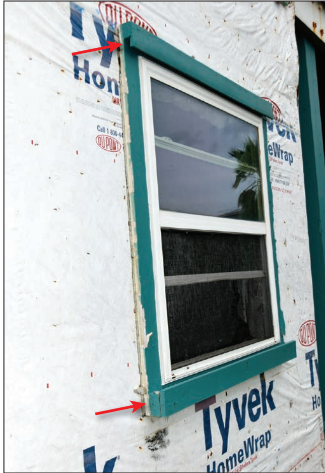
Figure 4-59: Sliding plywood shutter frame system (red arrows) on house (Port Aransas)
