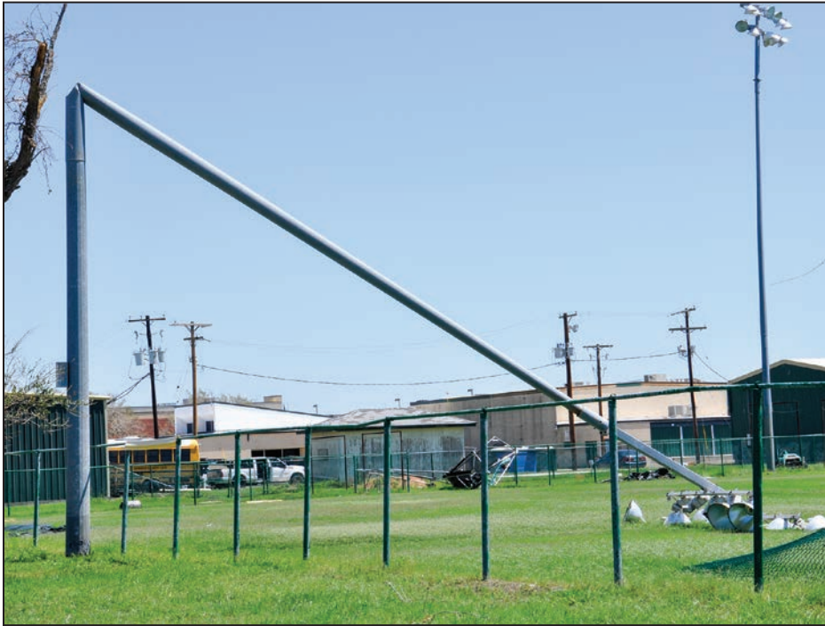
Figure 4-142: Collapsed light fixture pole (high school buildings are in the background)
