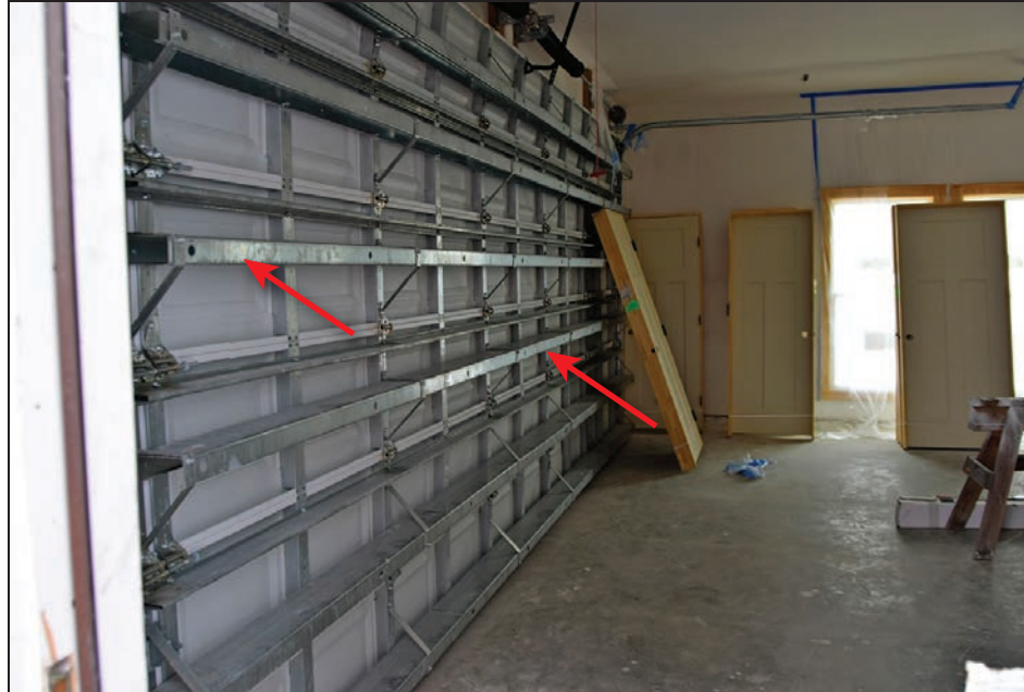
Figure 4-64: 20 feet x 9 feet hurricane-rated garage door that was not tested by debris impacts; red arrows show hurricane door stiffeners (Cape Valero)
