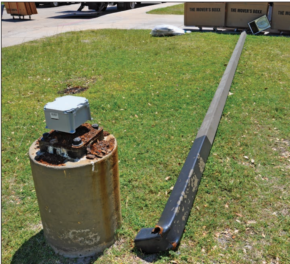
Figure 4-104: Collapsed light fixture. There was significant corrosion of the tube near the base plate
