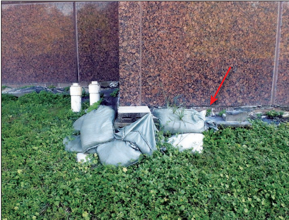
Figure 3-63: Unsealed joint between the concrete foundation wall and reinforced masonry wall with granite façade where significant seepage into the Wortham Theater occurred
