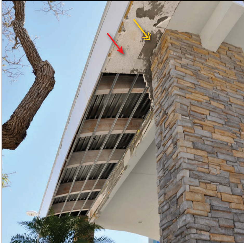
Figure 4-137: Soffit failure at the porte cochere
