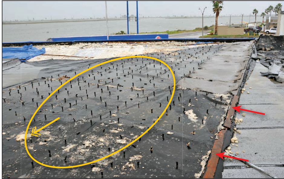
Figure 4-130: Underside of the base sheet (yellow oval)
