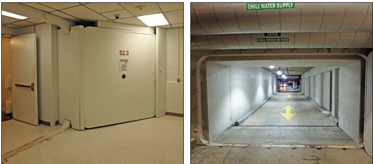
Figure 3-99: Flood doors in basement tunnel (left) and below-grade parking garage (right)
