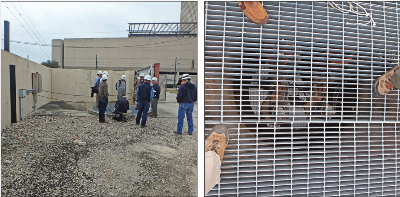
Figure 3-121: Substation sump pit and pumps
