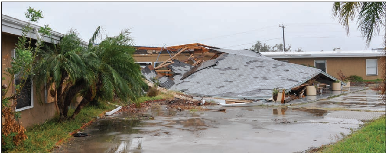
Figure 4-72: Collapsed porte cochere at a nursing home
