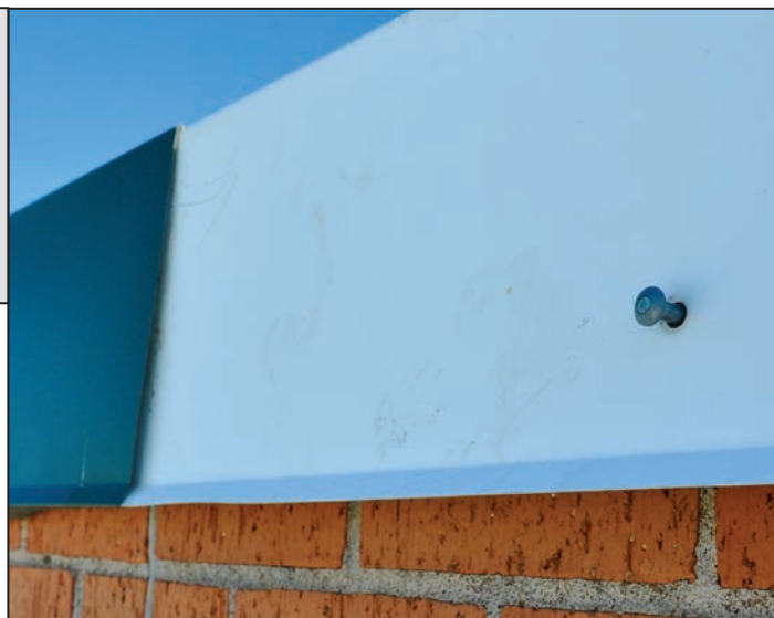
Figure 4-115: Area where a section of newer coping blew off
