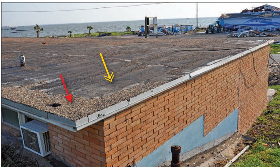
Figure 4-97: Roof of the building shown in Figure 4-96 showing extensive aggregate blow-off
