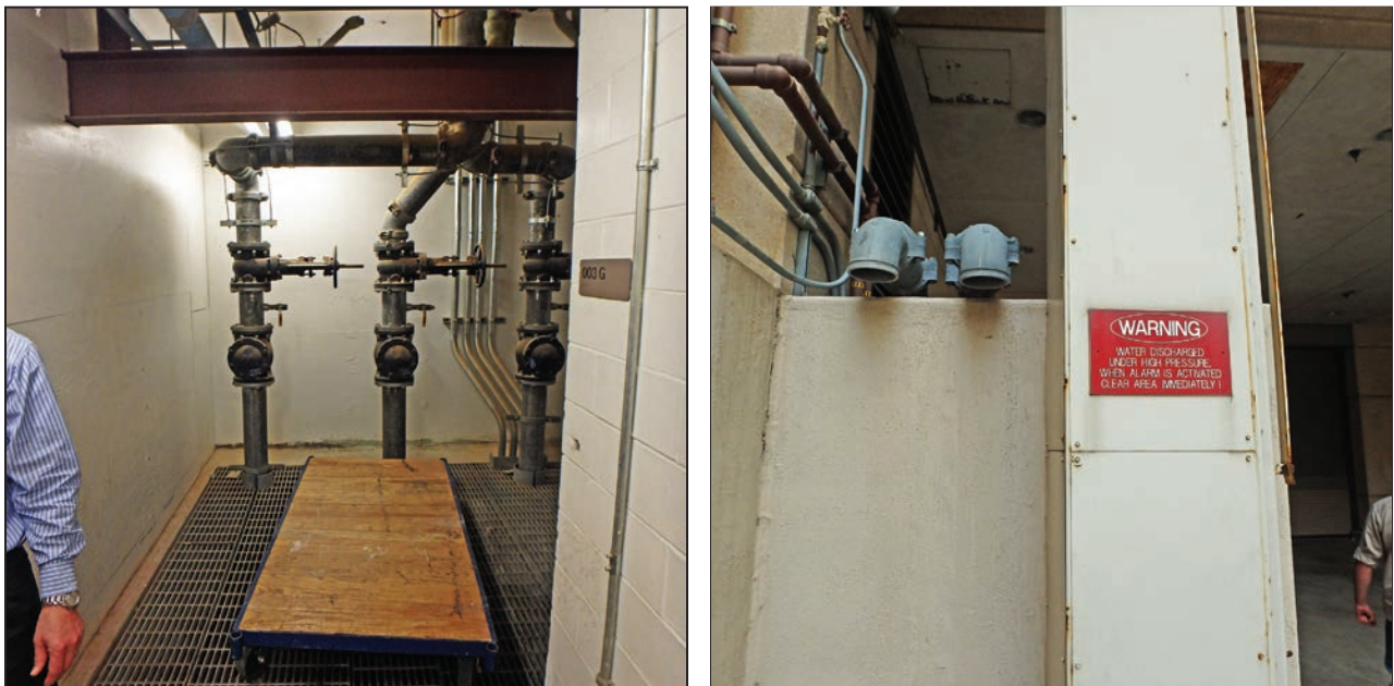
Figure 3-115: Typical sump pit in basement (left) and ejection pipes over floodwall (right)
