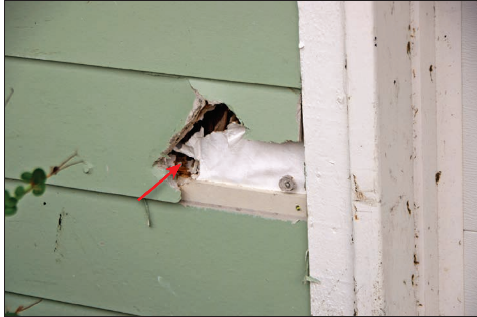
Figure 4-67: Impact from 2x4 on fiber cement siding (red arrow) (120 mph, Exposure C) (Key Allegro)
