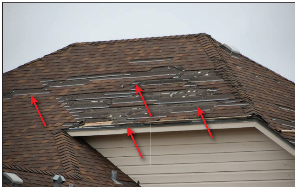
Figure 4-34: Home that lost shingles due to poor adhesion of the leading edges of the shingles (red arrows) (Port Aransas)
