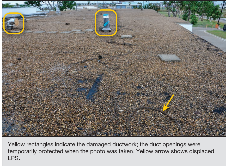
Figure 4-95: Damaged ductwork at the fisheries laboratory
