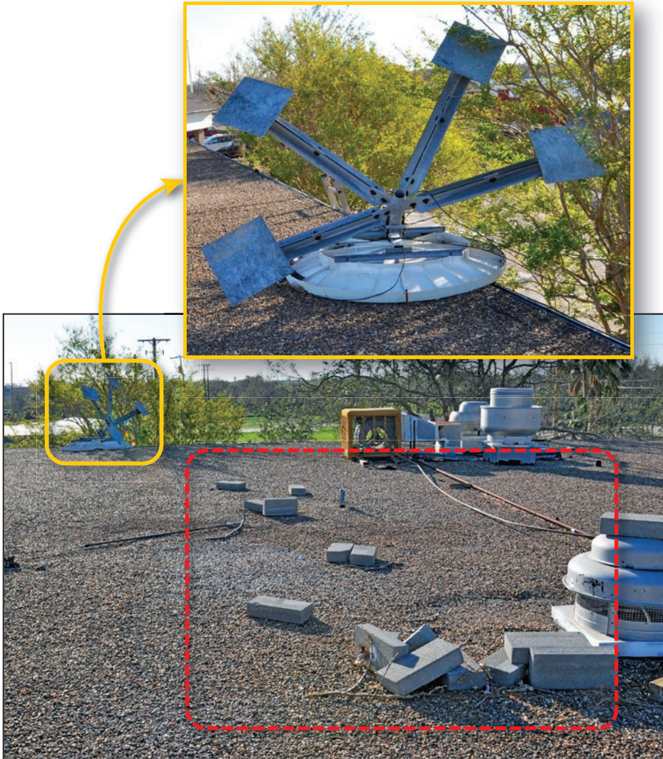
Figure 4-91: Displaced satellite dish (yellow box) and masonry ballast (red dashed box)
