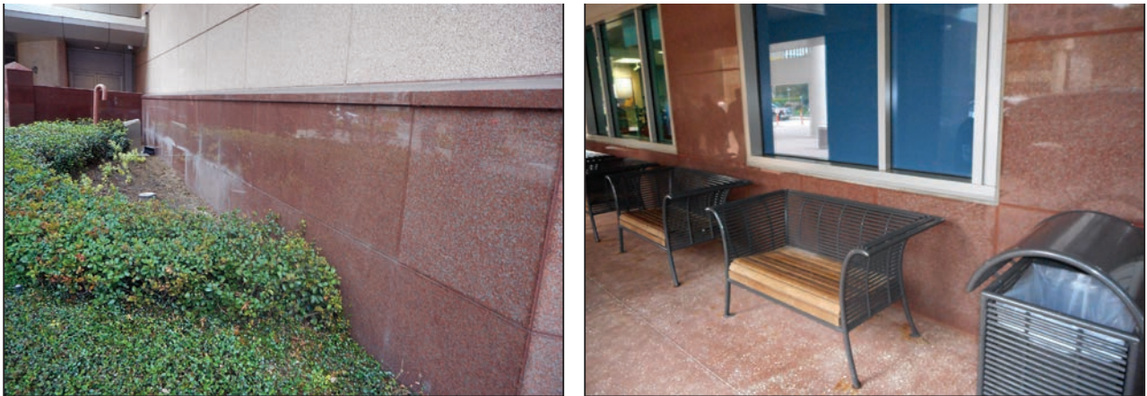
Figure 3-104: Marble-faced floodwall (left) and aquarium glass windows in floodwall (right) at the Main Building
