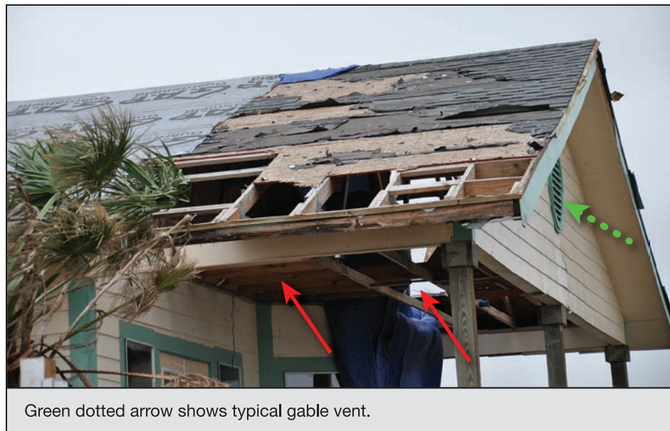
Figure 4-42: Home in which soffit and roof pressurization caused roof failure (red arrows) (120 mph, Exposure C) (Copano Village)
