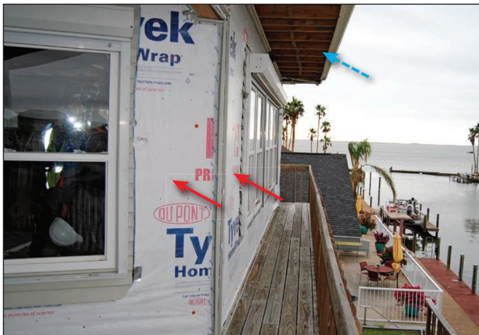
Figure 4-11: Home that lost vinyl siding (red arrows) and soffits (blue dashed arrow) (120 mph, Exposure C) (Holiday Beach)
