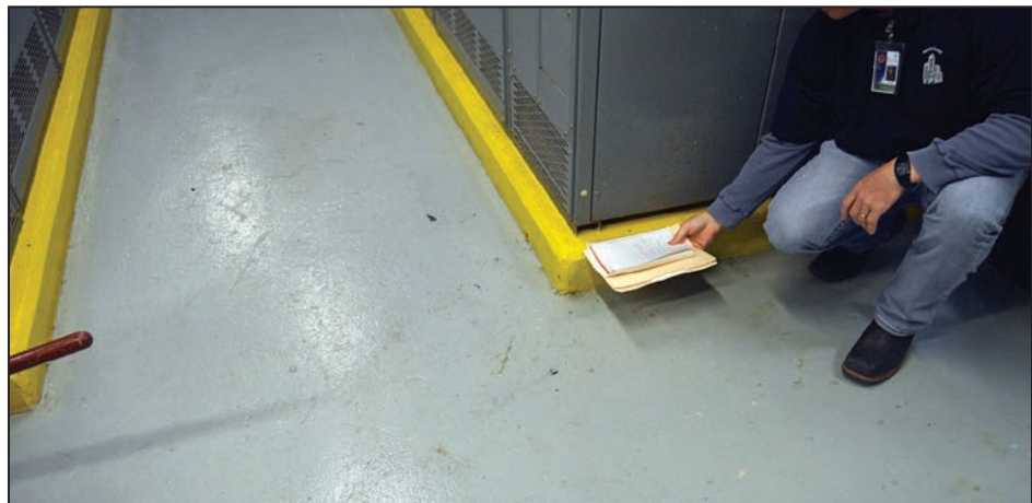
Figure 3-31: Maximum water depth at the electrical service equipment
