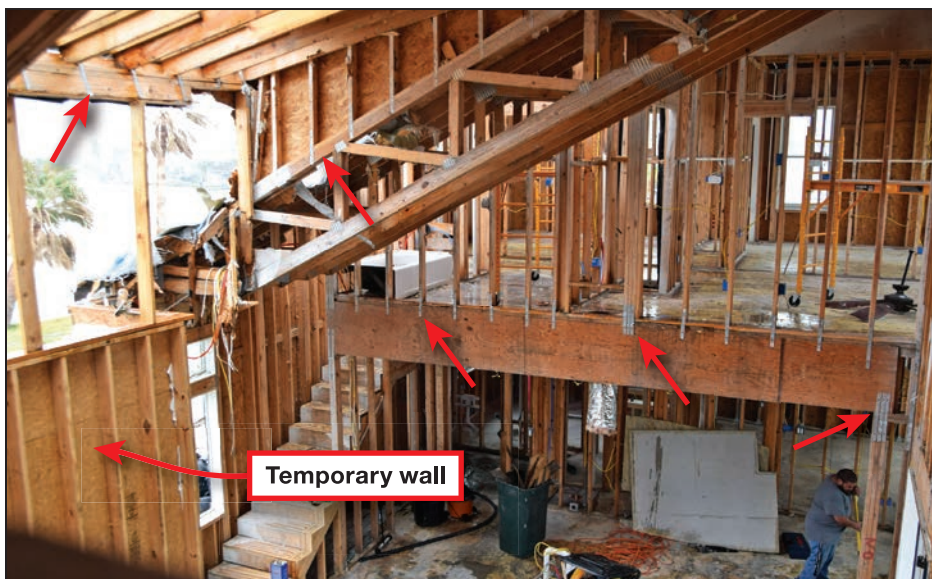
Figure 4-8: Wind-resistant connections (red arrows) (same building as Figure 4-7) (Rockport)
