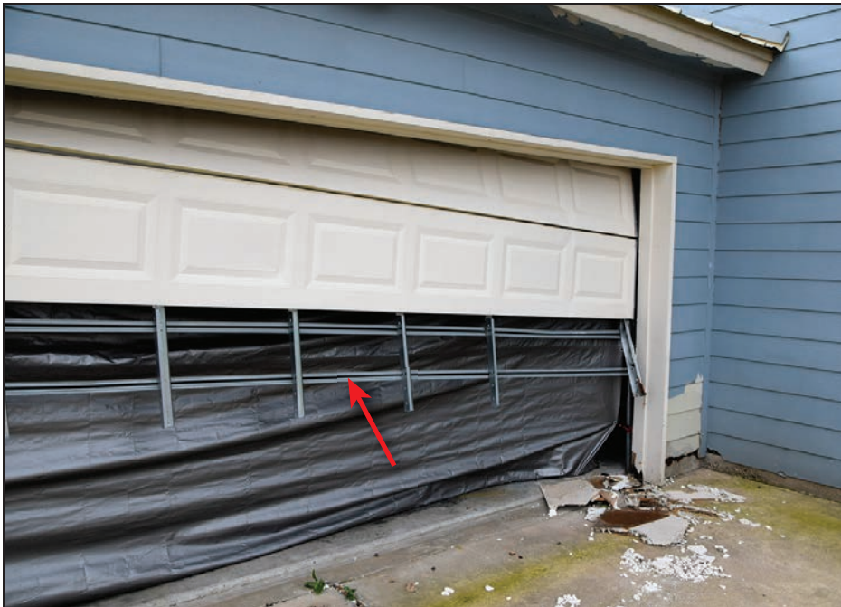
Figure 4-63: Hurricane-rated garage door that was damaged (red arrow); cause of failure unknown (Cape Valero)
