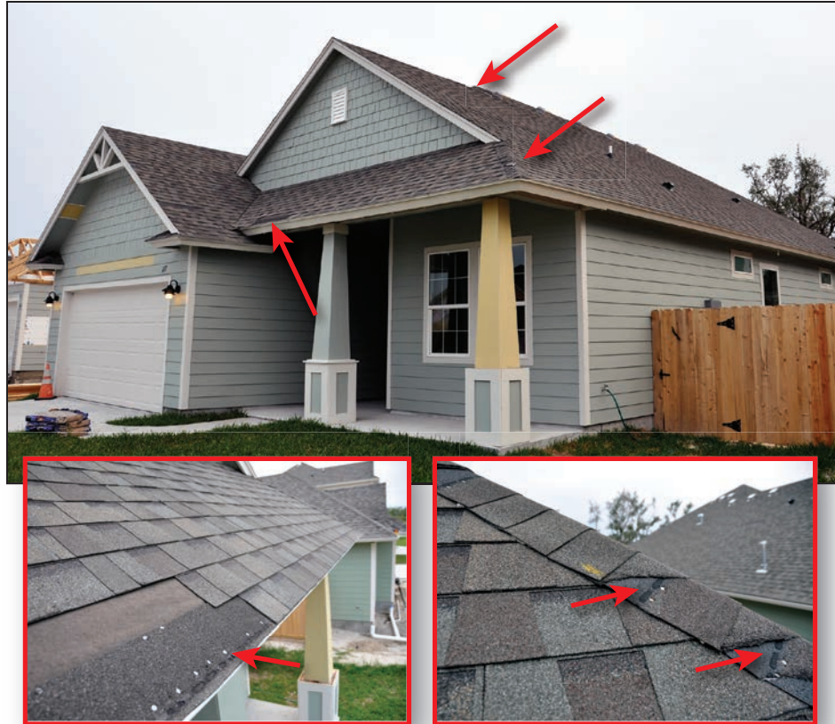
Figure 4-36: Home with damaged ridge, hip-ridges, and eave shingles (red arrows) due to poor adhesion of the shingle tabs (Fulton)
