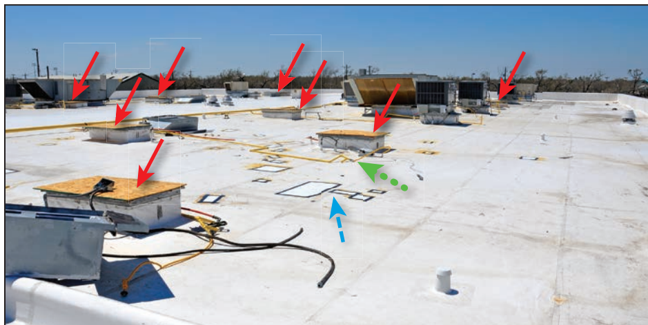
The red arrows indicate where HVAC units were blown off their curbs (the curb openings were temporarily covered with plywood). Emergency patches had been installed at membrane punctures (blue dashed arrow). The gas lines (green dotted arrow) had ruptured.
