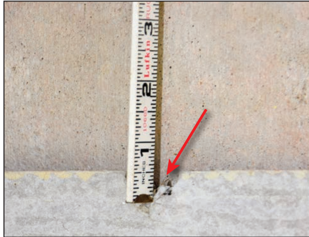
Figure 4-15: Fastener installed in fiber-cement siding ½ inch from edge, which led to failure of the plank attachment (Port Aransas)
