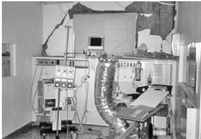
FIGURE C13.1-3 Collapsed Duct and HVAC Diffuser
