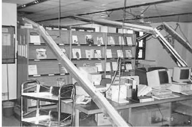
FIGURE C13.1-2 Collapsed Light Fixtures
