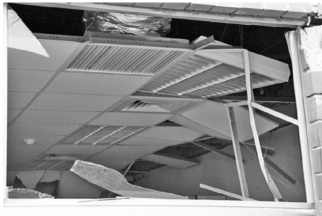
FIGURE C13.1-4 Damaged Ceiling System
