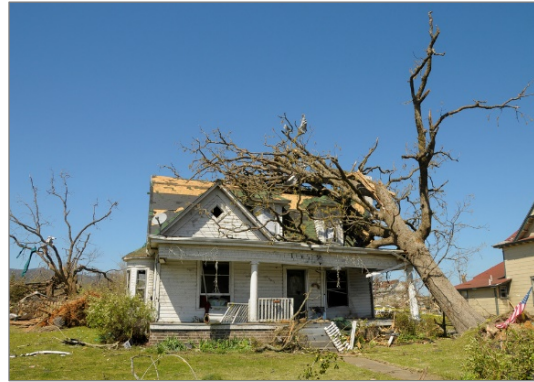
A home in Arkansas is damaged by a fallen tree.
