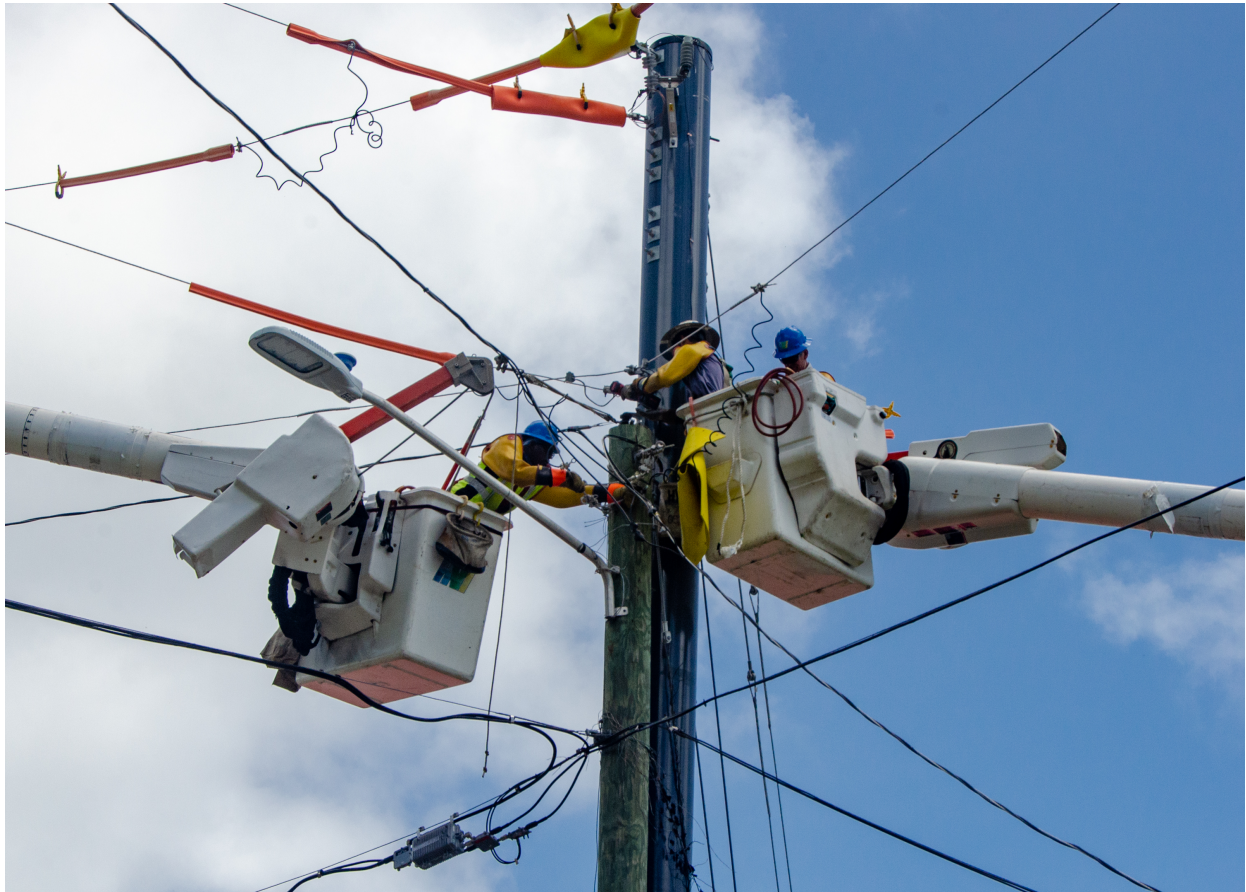
Haugland Virgin Islands line workers finish installation of a composite power pole in July 2021 in Upper Contant on St. Thomas. The Virgin Islands Water and Power Authority is leading operations to install 2,333 composite poles on the island. FEMA/Eric Adams
