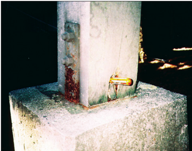
Wood decay at the base of a wood post supported by concrete.
