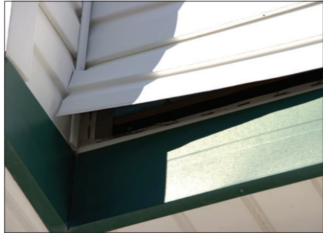
Figure 4. Utility trim was substituted for the starter strip and the bottom lock was cut off the siding. Siding was able to pull loose under wind pressure.
