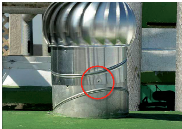
Figure 13. This turbine head is attached to the standpipe with dimple punches. Sheet metal screws should be added to strengthen the connection.
