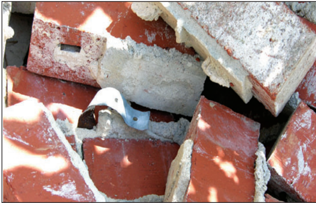
Figure 4. This tie remained embedded in the mortar joint while the smooth-shank nail pulled out from the stud.
