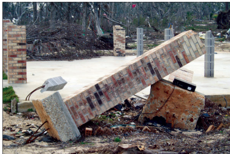
Figure 2. Performance comparison of pier foundations. Piers on discrete footings (foreground) failed by rotating and overturning while piers on more substantial footings (in this case a concrete mat) survived (Pass Christian, Mississippi)
