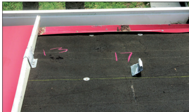
Figure 4. These eave clips were too far from the panel ends. The clip at the left was 13" from the edge of the deck. The other clip was 17" from the edge. It would have been prudent to install double clips along the eave.
