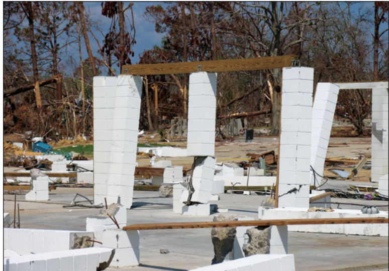
Figure 2. Pier breakage (Long Beach, Mississippi)
