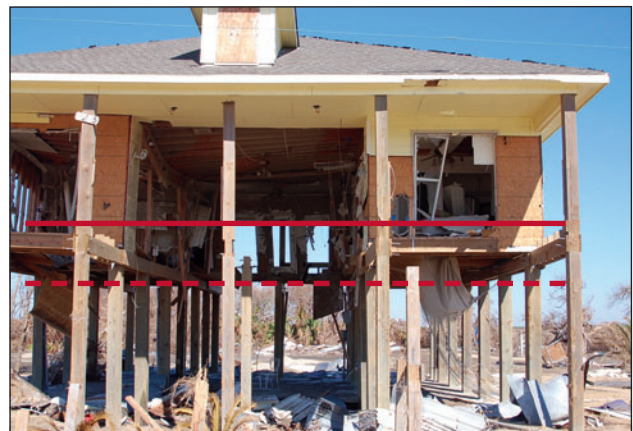
Figure 2. Bolivar Peninsula, Texas, V Zone house constructed with the lowest floor (bottom of floor beam) at the BFE (dashed line). The estimated wave crest level during Hurricane Ike (solid line) was 3' to 4' above the BFE at this location.
