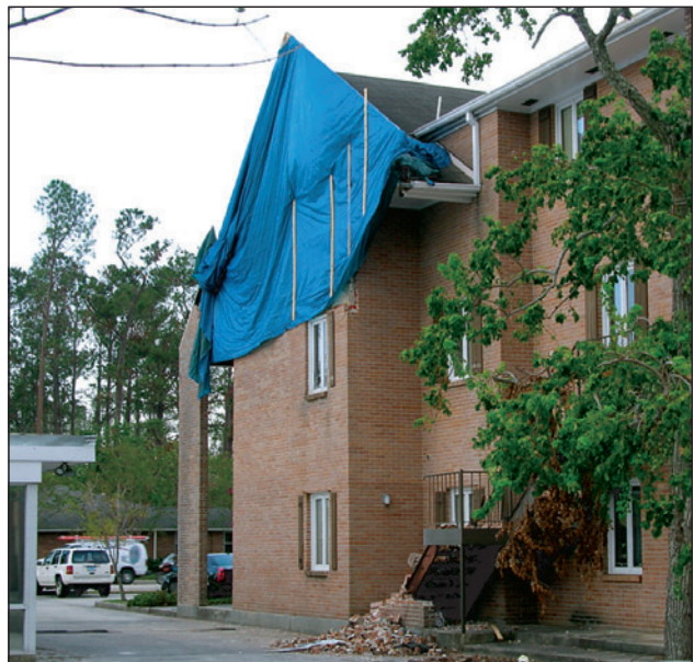
Figure 2. The upper portion of the brick veneer at this apartment building collapsed. Pedestrian and vehicular traffic in the vicinity of the damaged wall are vulnerable to injury and damage if remaining portions of the wall were to collapse during subsequent storms.
