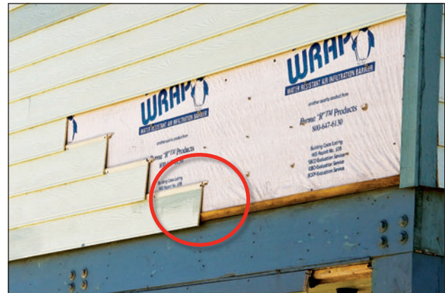
Figure 12. Blind nailed siding installed with exposed gap at bottom (red circle) is vulnerable to failure.
