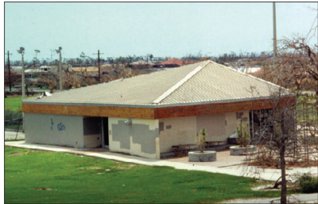
Figure 1. This structural standing seam roof system survived Hurricane Andrew (Florida, 1992), but some hip flashings were blown off. The estimated wind speed was 170 mph (peak gust, at 33 feet for Exposure C).
