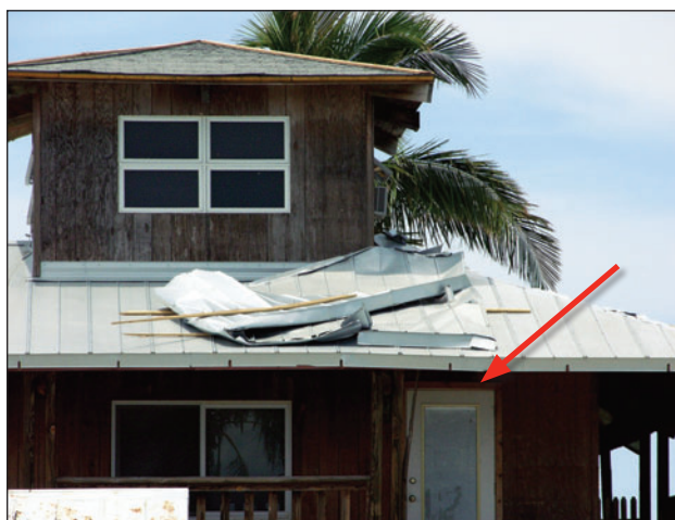
Figure 5. The panels blew off the upper roof and landed on the lower roof of this house. The upper asphalt shingle roof shown had been re-covered with 5V-Crimp panels that were screwed to nailers. The failure was caused by inadequate attachment of the nailers (which had widely-spaced nails) to the sheathing. Note that the hip flashing on the lower roof blew off.
