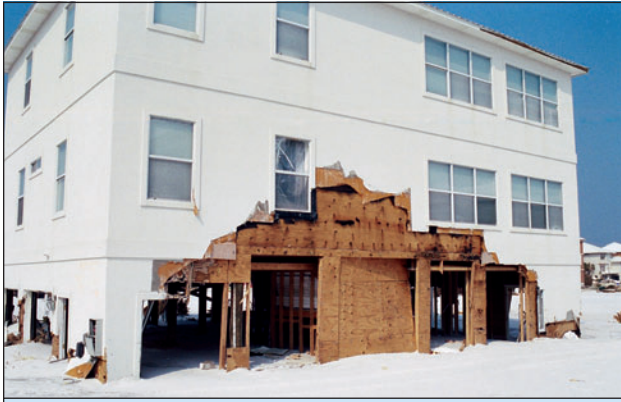
Figure 4. Building siding extended down and over the breakaway wall. Lack of a clean separation allowed damage to spread upward as the breakaway wall failed.
