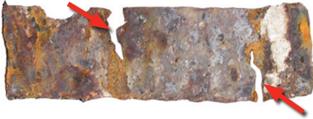
Figure 3. Significant tie corrosion caused the brick at a fire station to fail, even though the building is not near the coast. Note that metal is missing for half of the width of the tie at two locations (red arrows). The left end of the tie was still embedded into a concrete masonry unit back-up wall. The right end is where the tie failed in tension, thus leaving a portion of the tie embedded in the collapsed brick.
