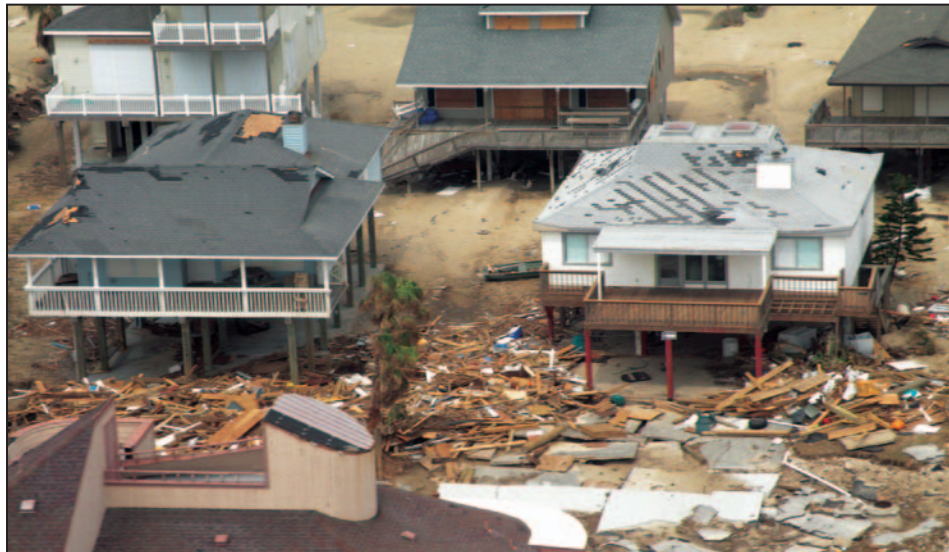
Figure 2-11. Galveston Island beach house with wind damage to roof in high pressure zones at roof edge and roof corners, Hurricane Ike, 2008
