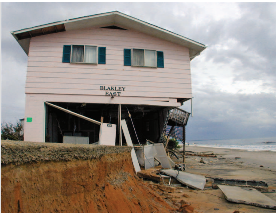
Figure 3-33. Erosion undermining a coastal residence in Oak Island, NC, caused by Hurricane Floyd in 1999
