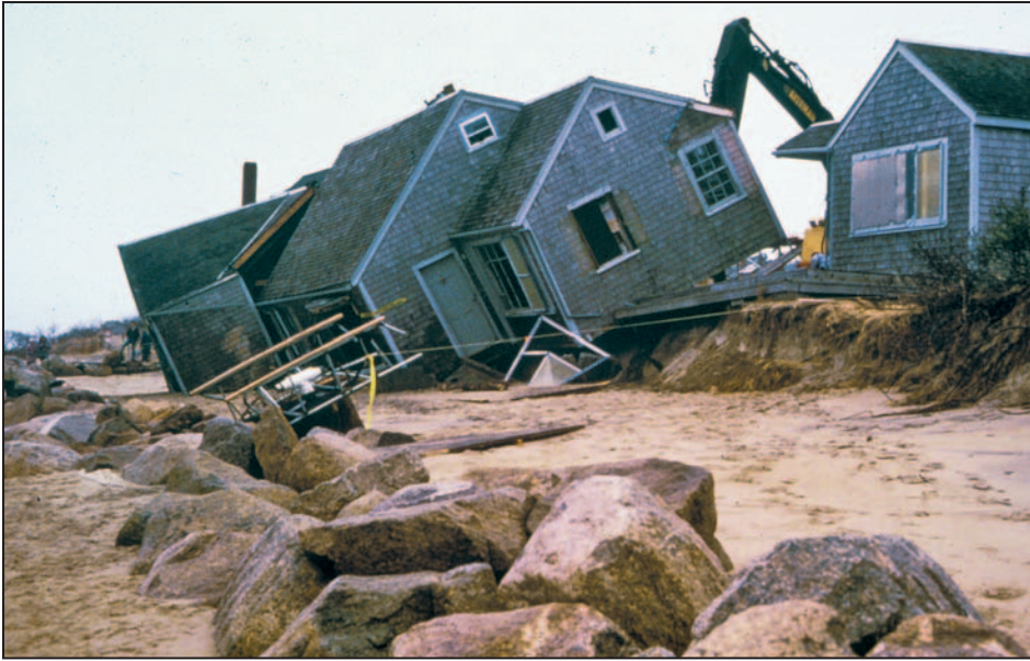
Figure 3-36. Undermined house at Chatham, MA, in 1988; nine houses were lost as a result of the formation of the new tidal inlet shown in Figure 3-35 SOURCE: JIM O'CONNELL, USED WITH PERMISSION
