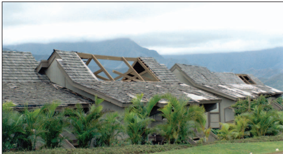
Figure 3-9. Loss of roof sheathing due to improper nailing design and schedule in Kauai County, HI (Hurricane Iniki, 1992)
