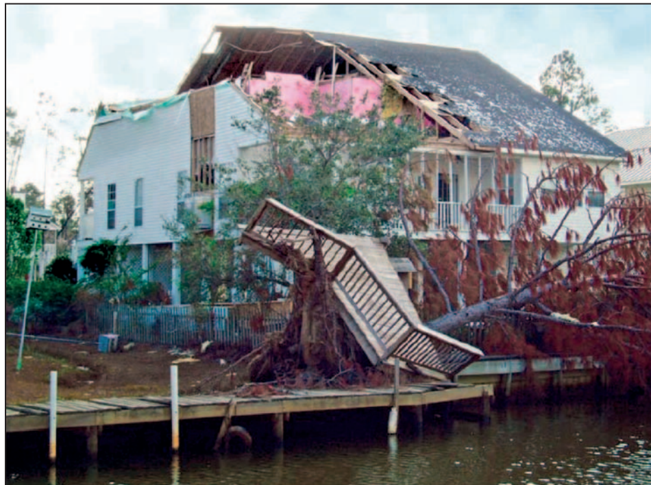
Figure 2-17. Wind damage to roof structure and gable end wall, Hurricane Katrina (Pass Christian, MS, 2005)
