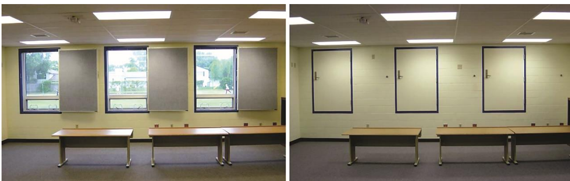
Figure A4-5: Interior operated safe room shutters in a multi-purpose classroom/safe room. Image on left is normal usage; image on right shows shutters in "lock down" position where they are closed and latched
