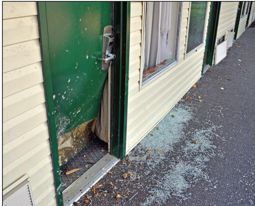
Figure B8-18: This metal door was damaged by wind-borne debris generated by a weak tornado. The bottom hinge was damaged, but the single latch was able to resist the modest wind and impact load. The door was on the verge of failing. (St. Louis, Missouri, 2013 tornado)
