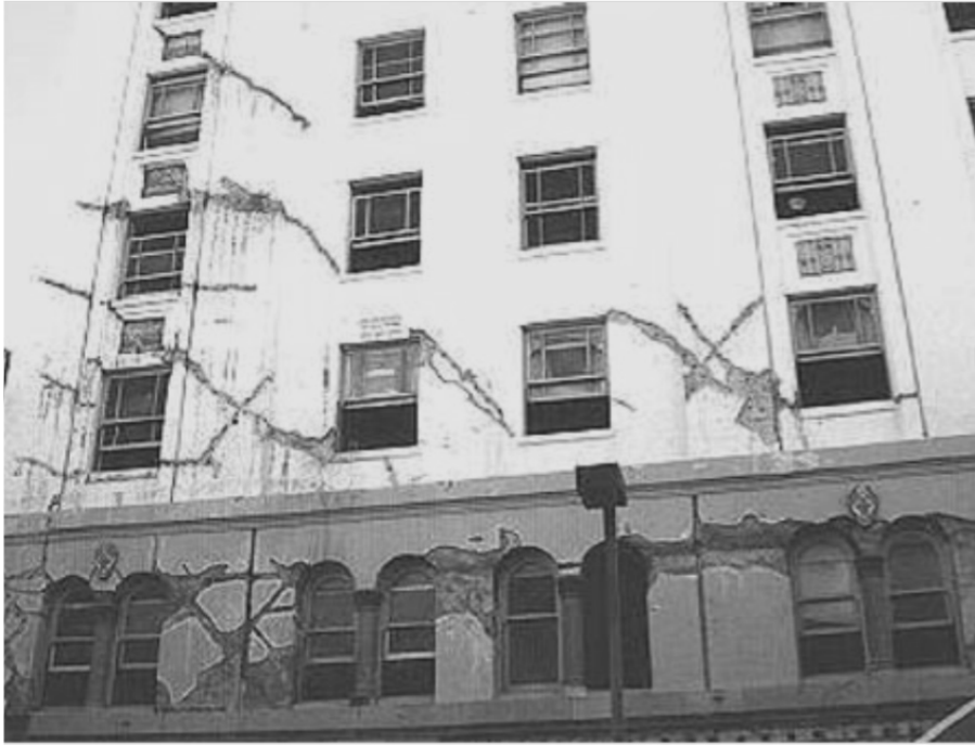
Figure E-31 Shear wall damage, 1989 Loma Prieta earthquake.
