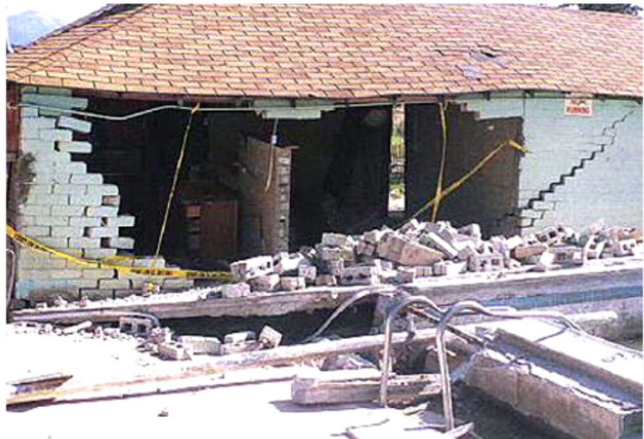
Figure E-53 Damaged URM building, 1992 Big Bear earthquake.
