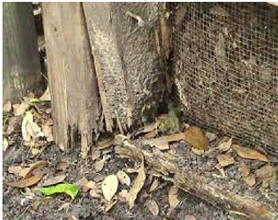
Figure F-2 Damaged wood post.
