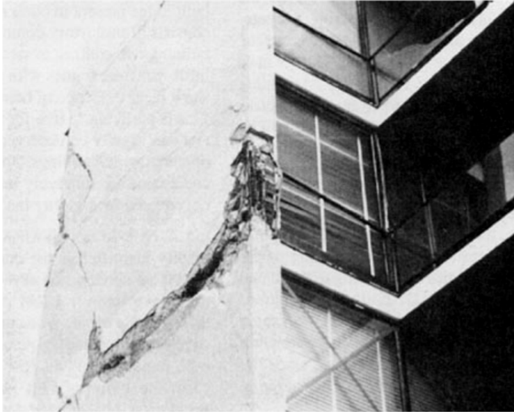
Figure E-21 Close-up of exterior shear wall damage during a major earthquake.
