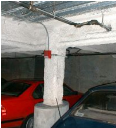
Figure 3-42 Interior view showing fire-proofed columns and beams, which indicate a steel building (S1, S2, or S4).
