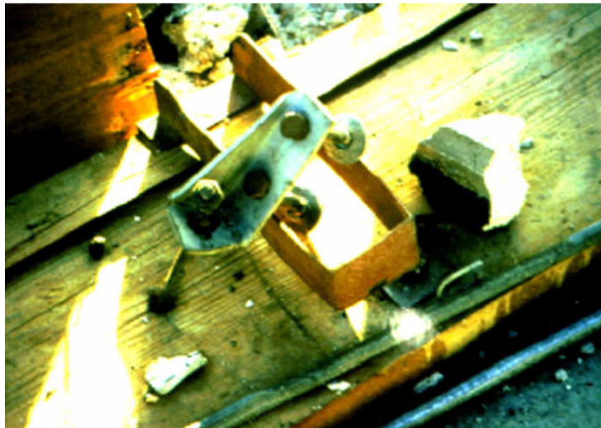
Figure E-37 Tilt-up construction anchorage failure.
