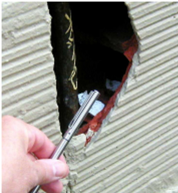
Figure D-14 Hollow clay tile wall with punctured tile.
