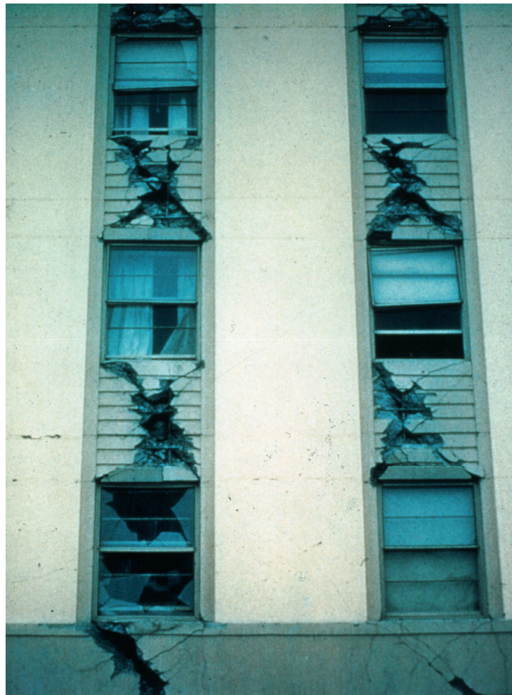
Figure E-30 Tall concrete shear wall building: walls connected by damaged spandrel beams.
