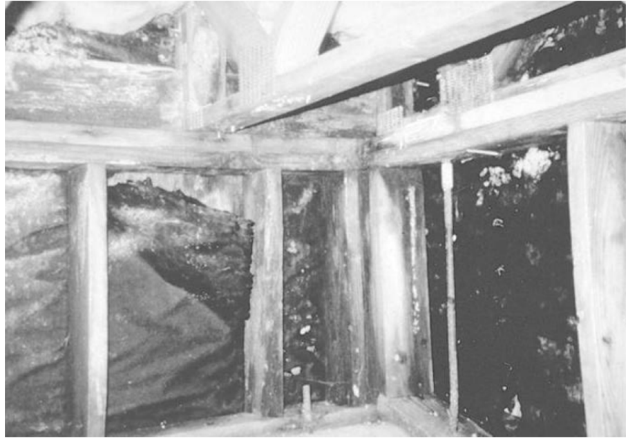
Figure F-1 Wood decay in cripple wall.
