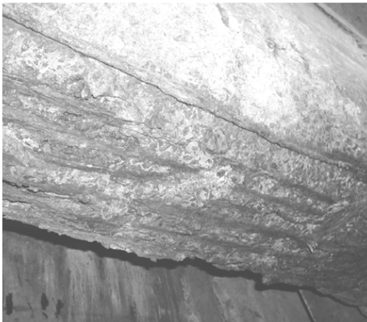
Figure F-6 Exposed reinforcing steel.
