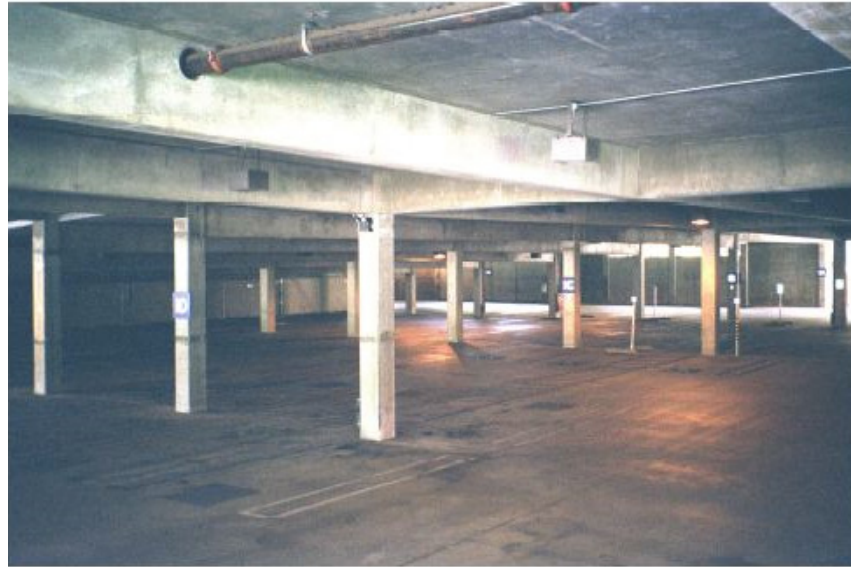
Figure 3-43 Interior view showing concrete columns and girders with no identifiable shear walls, which indicates a concrete moment frame (C1).
