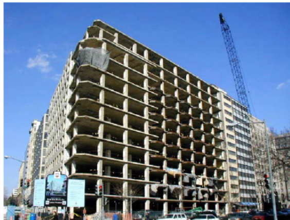
c. New precast façade units being applied to reinforced concrete frame buildings.
