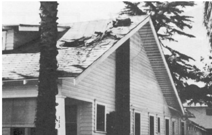
Figure G-4 Collapsed chimney with damaged roof, 1987 Whittier Narrows earthquake.
