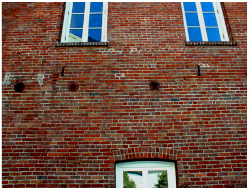
Figure E-54 Two existing anchors above three new wall anchors at floor line using decorative washer plates.
