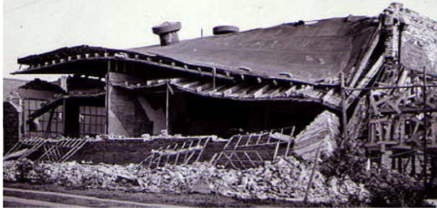
Figure G-8 Collapse of unreinforced masonry bearing wall, 1933 Long Beach earthquake.
