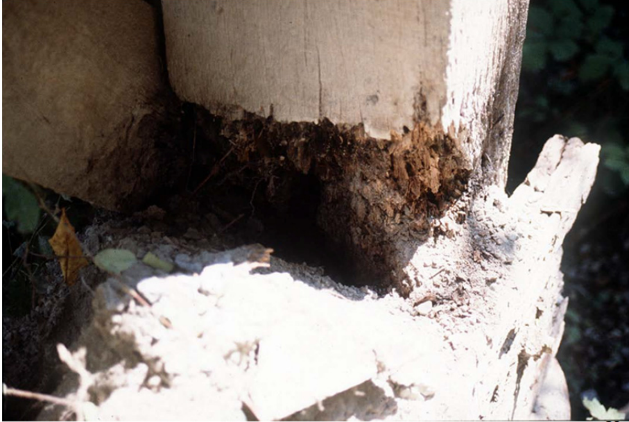
Figure F-3 Rotted timber column.
