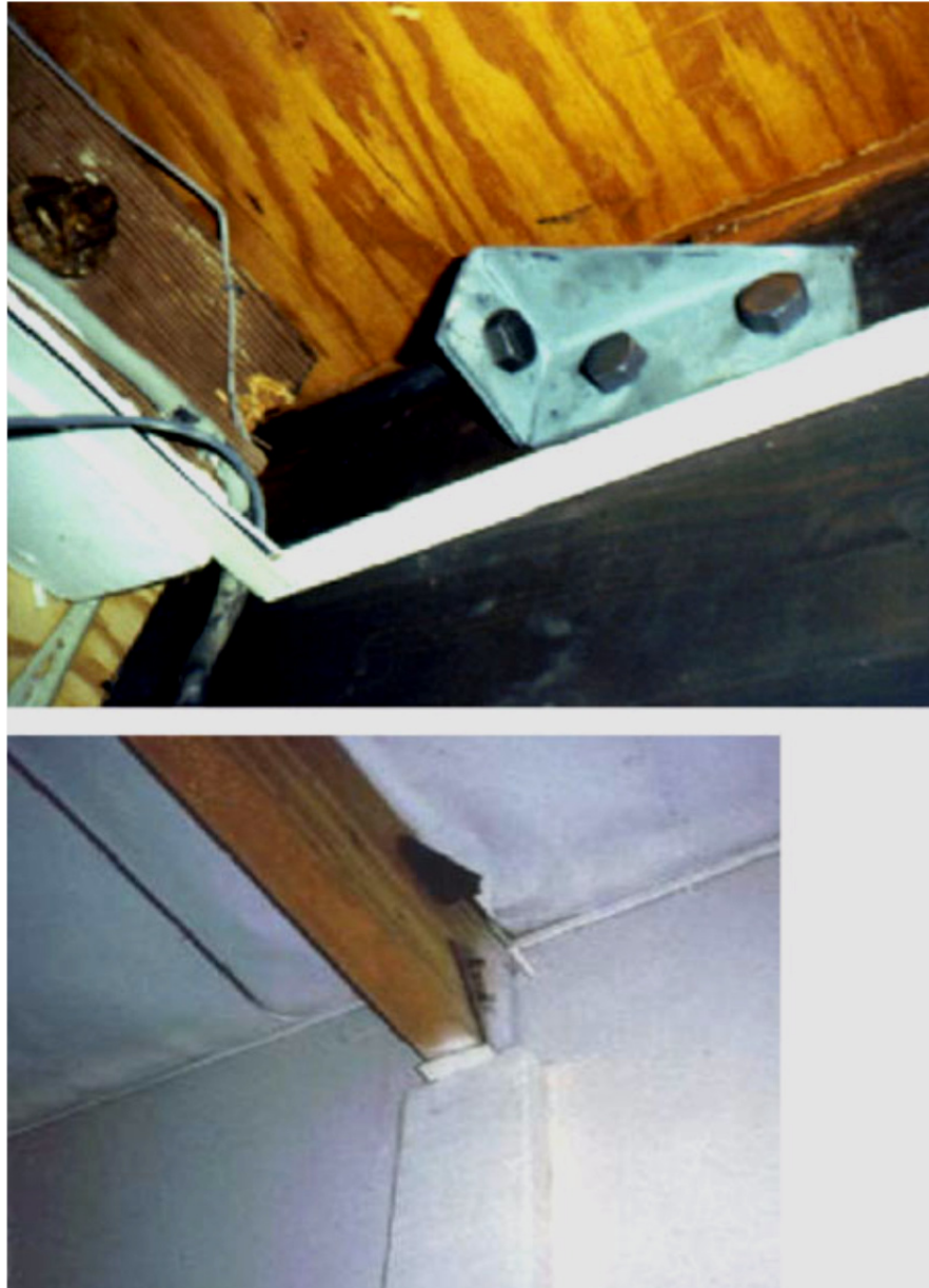
Figure E-39 Newly installed anchorage of roof beam to wall in tilt-up building.
