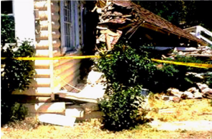
Figure G-6 Collapsed cripple stud walls dropped this house to the ground, 1992 Landers and Big Bear earthquakes.
