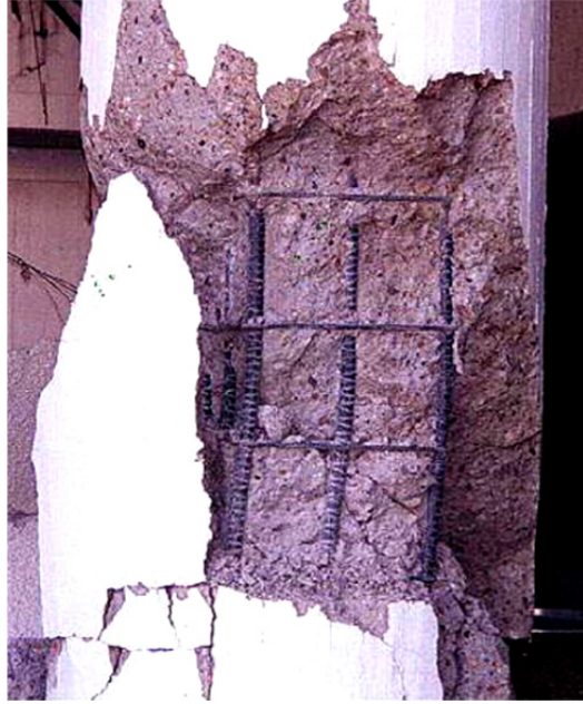
Figure E-26 Example of ductile reinforced concrete column, 1994 Northridge earthquake; horizontal ties would need to be closer for greater demands.
