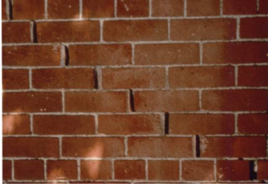
Figure F-9 Masonry joint separations.
