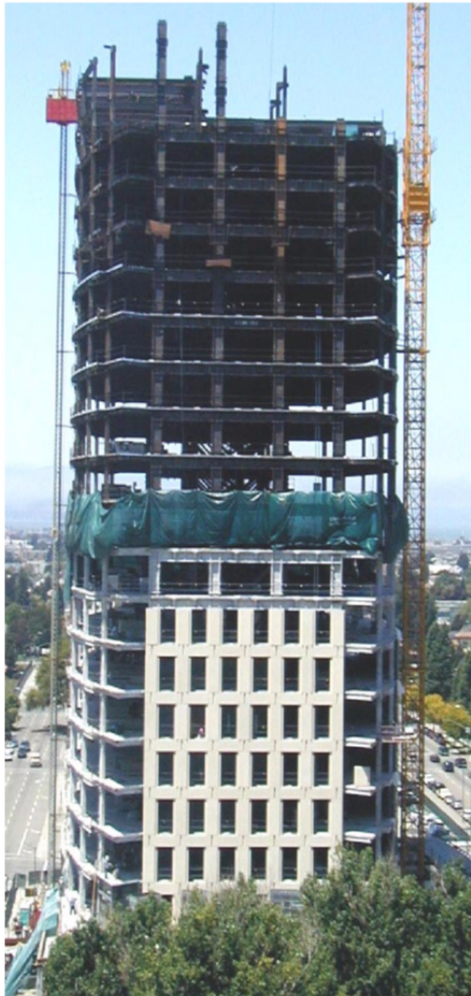
a. Building above is a high-rise steel dual system: moment frame (heavy columns and beams on upper façade) with bracing around elevator core. Fireproofing is being applied to steel at mid-height (inside the shroud) and precast façade elements are being attached to frame in lower stories.
