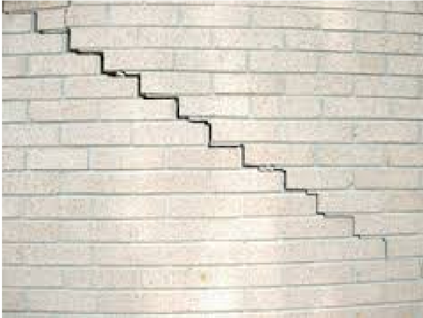
Figure F-8 "Stair-step" cracking.
