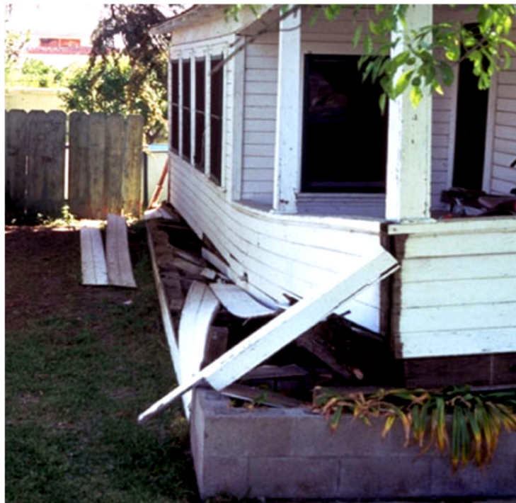
Figure E-8 House off its foundation, 1983 Coalinga earthquake.
