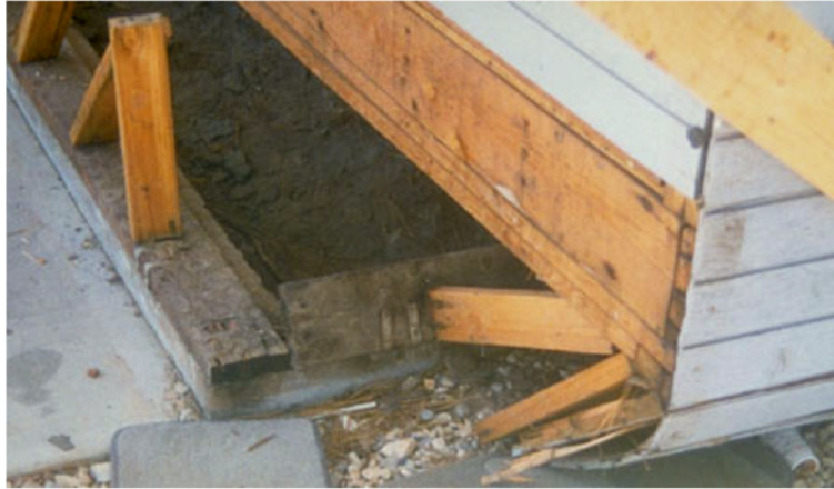
Figure E-9 Failed cripple stud wall, 1992 Big Bear earthquake.
