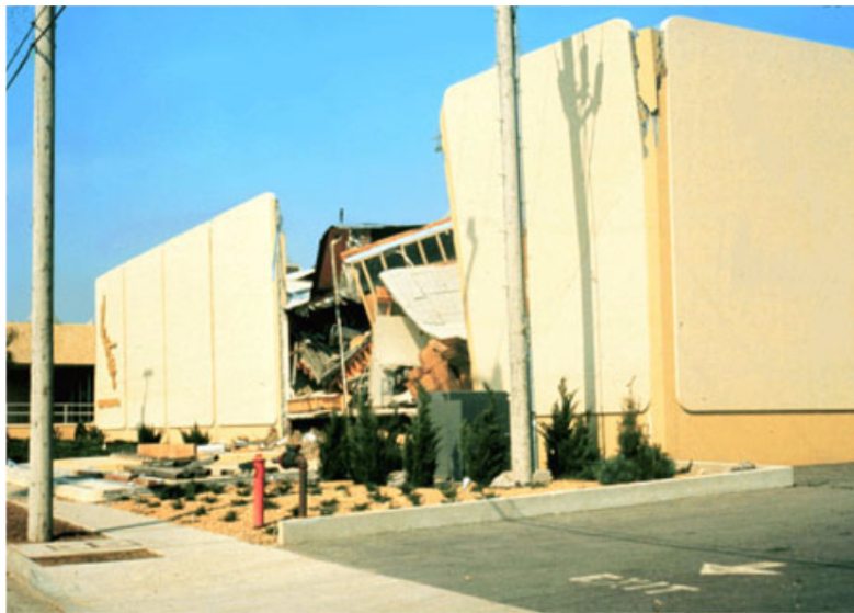
Figure G-9 Collapse of a tilt-up bearing wall, 1994 Northridge earthquake.
