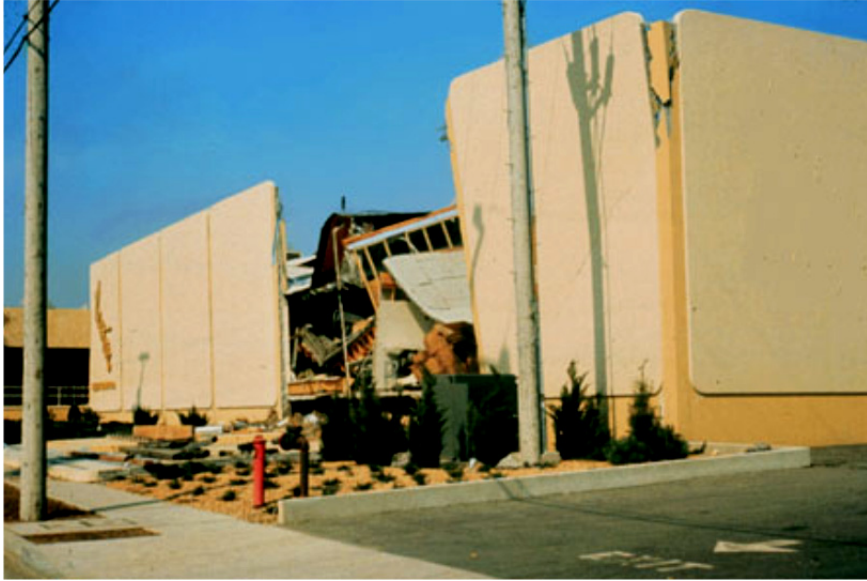
Figure E-38 Result of failure of the roof beam anchorage to the wall in tilt-up building.
