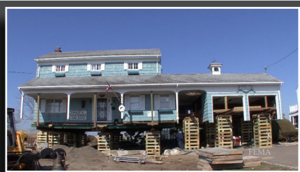
After being flooded by Hurricane Sandy, homeowners Al Grover and his wife raised their home 13 feet in order to mitigate from any future flood damage.
